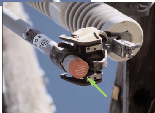
Figure 3-15 SMU-20 Fuse - Detail
