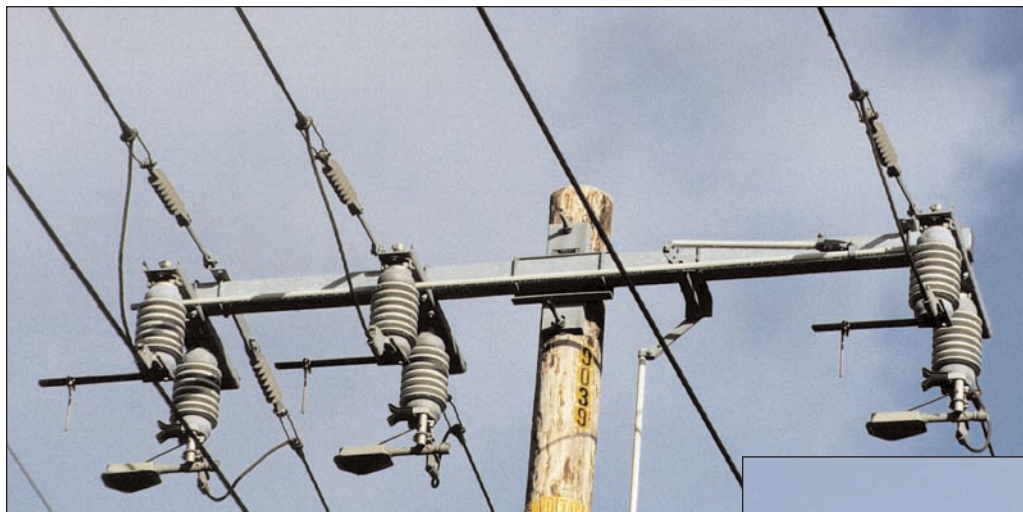
Figure 3-24 600 Amp Underarm Sidebreak Switch (open position)
