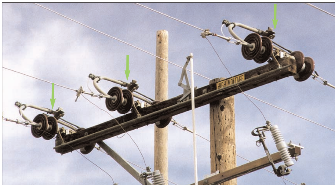
Figure 3-23 600 Amp KPF Air Switch, Crossarm Construction (closed position) without Arcing Horns or Snuffers
