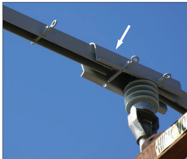
Figure 4-23 Close up of Insulator and Wire Cover
