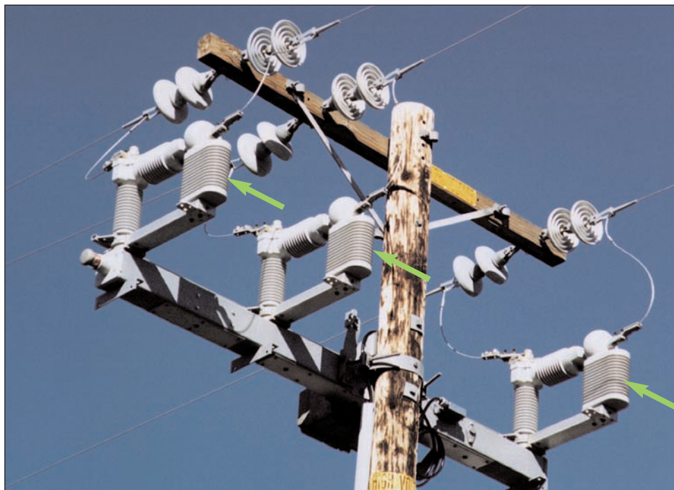
Figure 3-33 S&C Scada-Mate Switch
