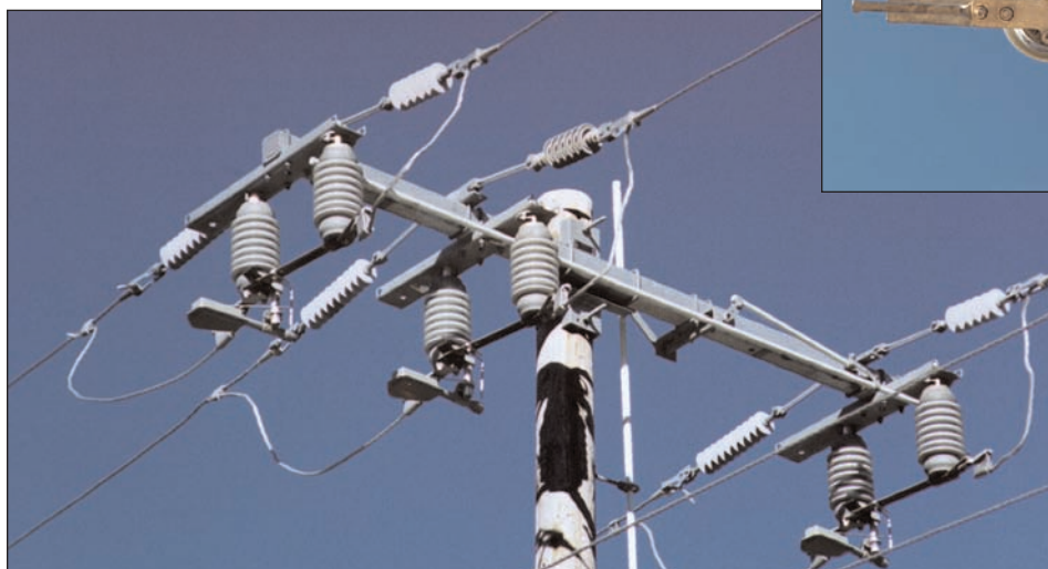
Figure 3-27 600 Amp Underarm Sidebreak Switch (closed position)
