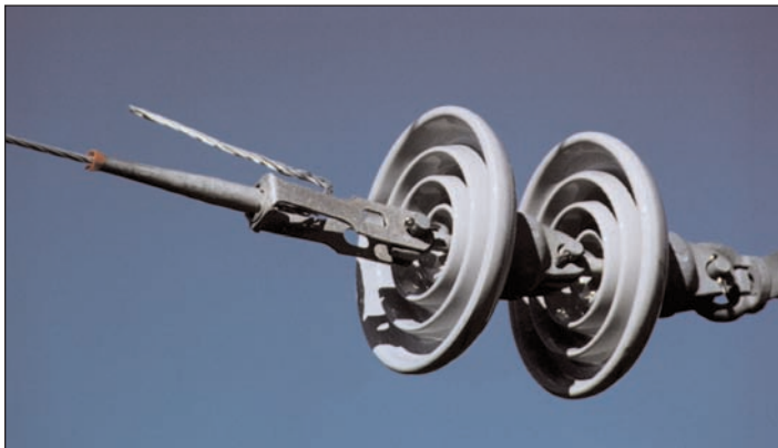
Figure 3-68 Automatic Deadends with Suspension Insulators
