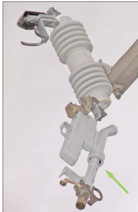
Figure 3-19 S&C Fault Tamer Fuse (Open)
