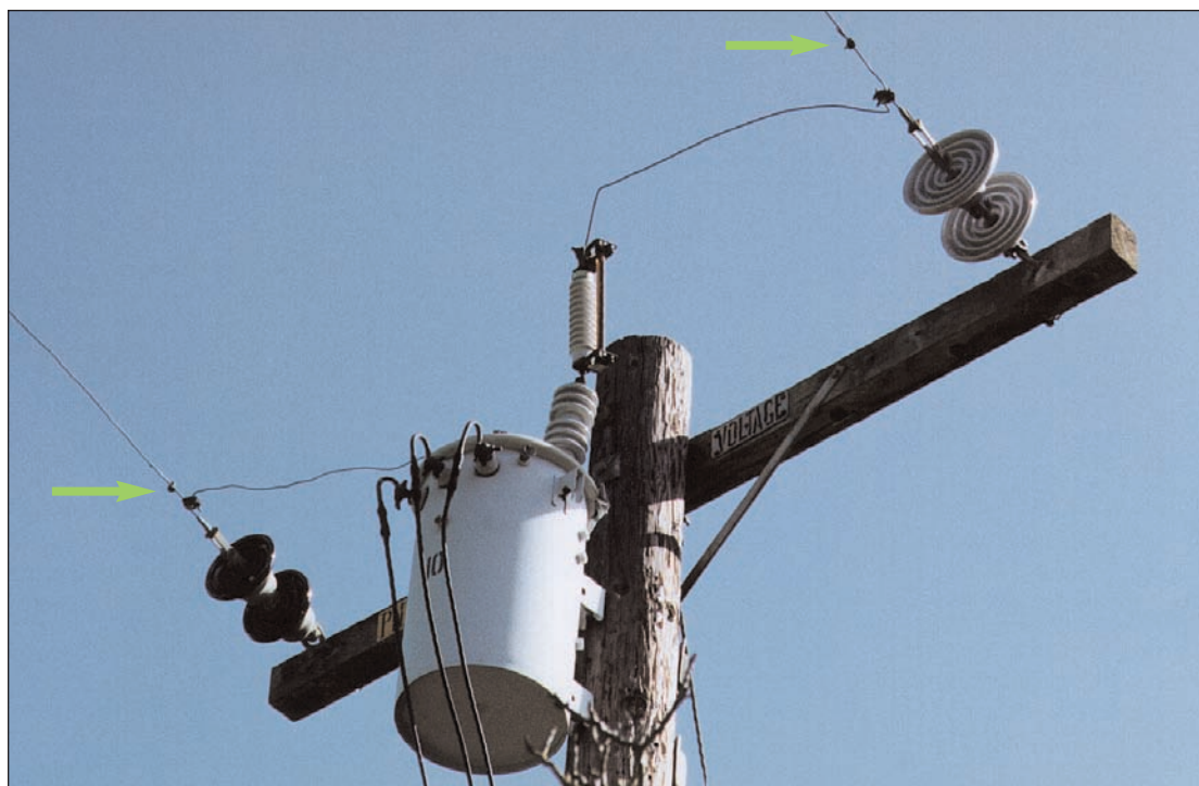
Figure 3-57 Idle Split Bolt Connectors
