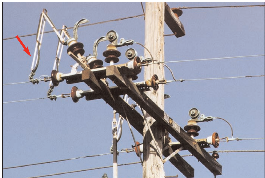
Figure 2-39 Grasshopper Air Switch (open position)
