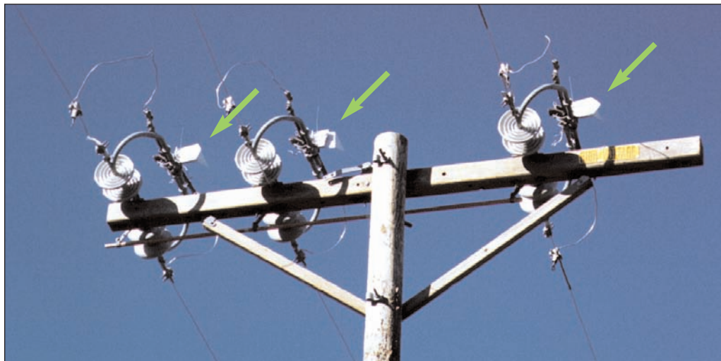
Figure 3-22 600 Amp KPF Air Switch, Crossarm Construction (closed position) with Arcing Horns and Snuffers
