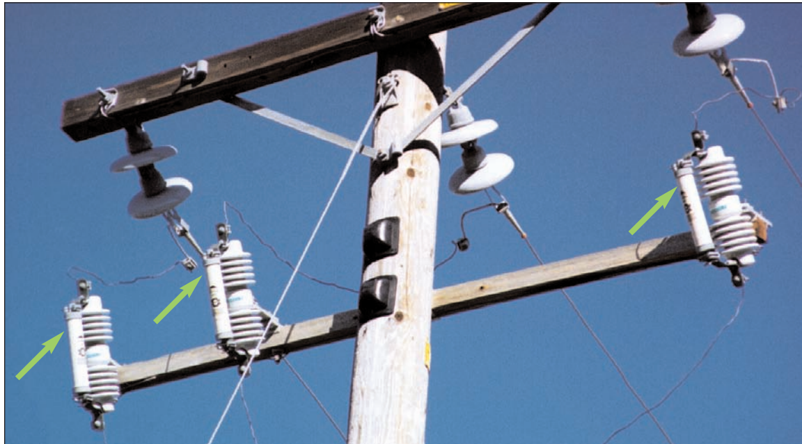
Figure 3-3 Arm Mounted Cutout with Non-Expulsion Fuses
