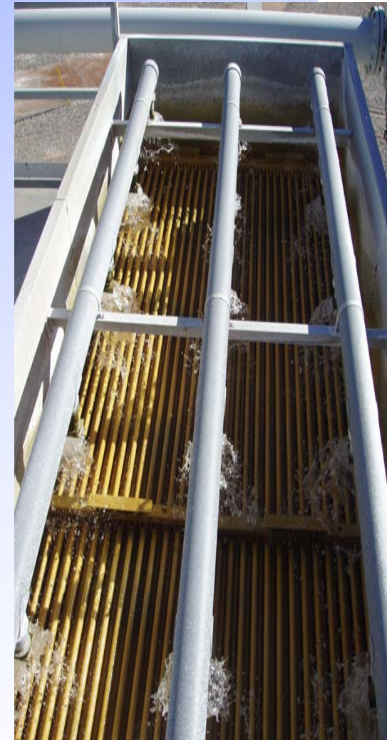
WSAC Spray Section (courtesy of Niagara Blower)
