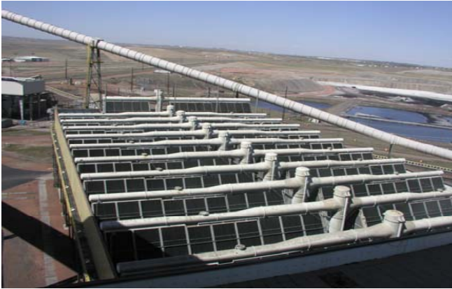
ACC at PacifiCorp's Wyodak Power Plant (courtesy of R. Garan)
