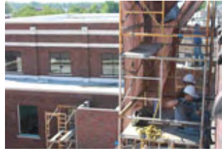
Construction of the new facilities at Gerald R. Ford is expected to be complete later this year.
