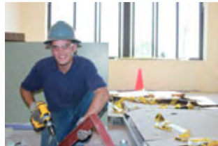
A student at Gerald R. Ford shows off his training skills and works hard on the construction of the center's new dorm.
