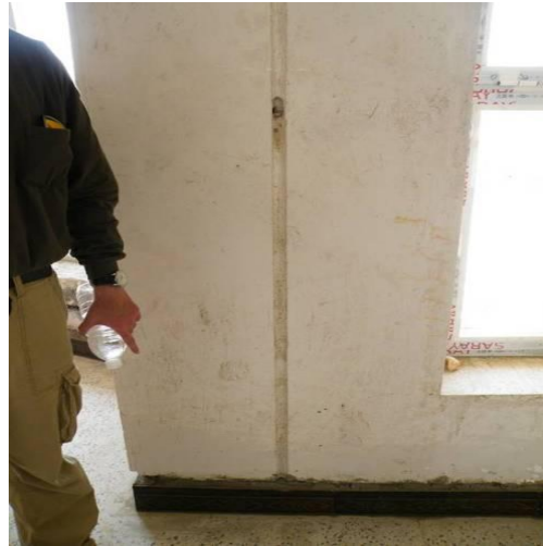
Site Photo 17. Wall expansion joint incorrectly filled with plaster
