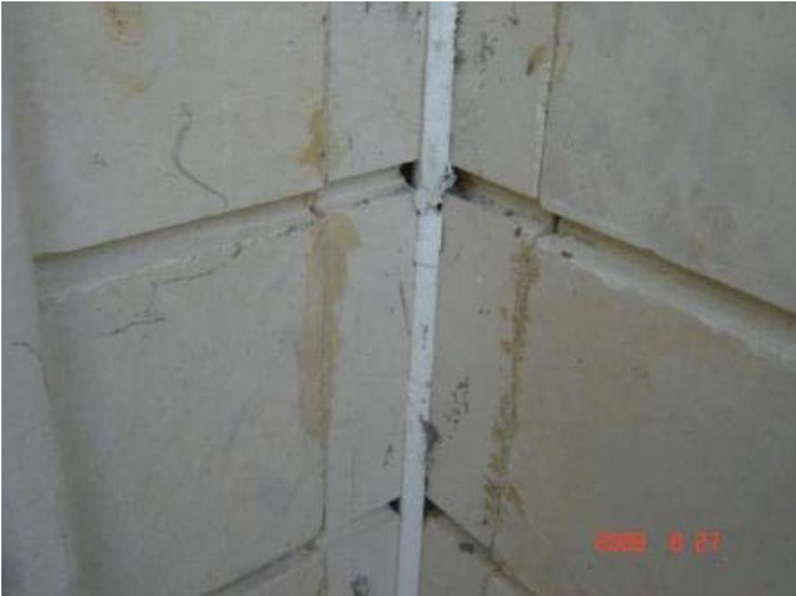
Site Photo 23. Contractor's initial attempts to add expansion joints to exterior of the facility (Courtesy of the USACE KRO)
