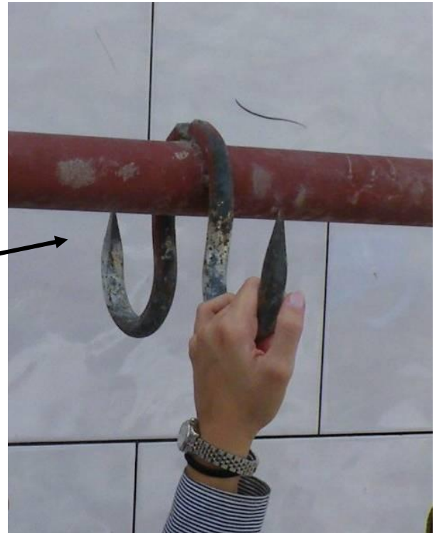
Site Photo 22. Close-up of exposed meat hook
