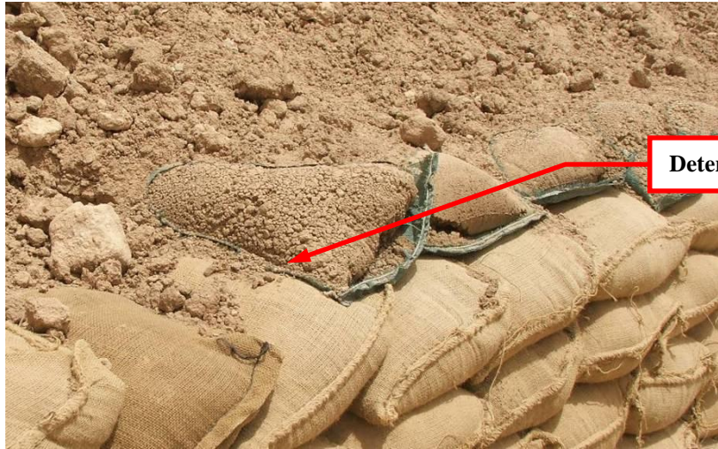
Site Photo 8. Deteriorating sandbags
