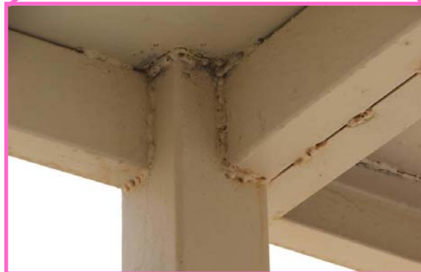
Site Photo 4. Poor weld quality at connections
