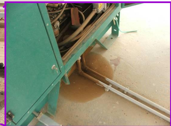
Site Photo 12. Fuel leak at joint
