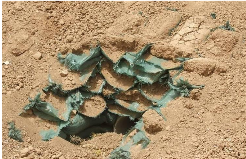
Site Photo 9. Deteriorating headwall
