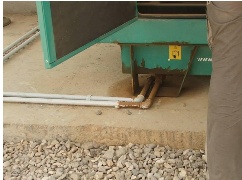
Site Photo 17. Fuel leak at joint
