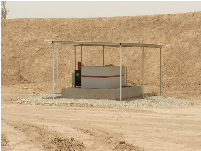
Site Photo 16. Sunshade with generator and fuel tank
