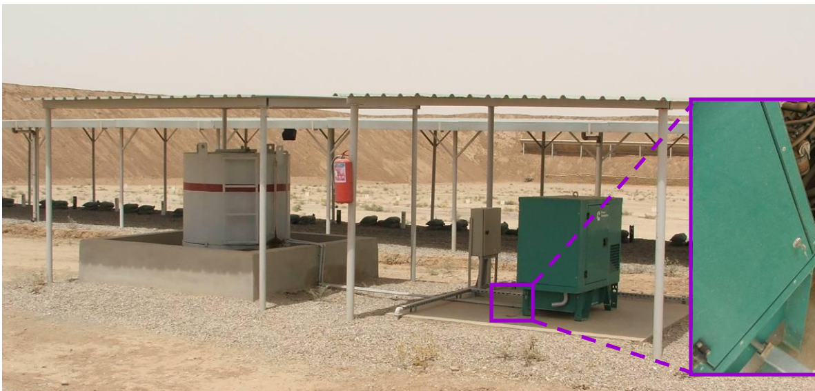
Site Photo 11. Sunshade with generator & fuel tank
