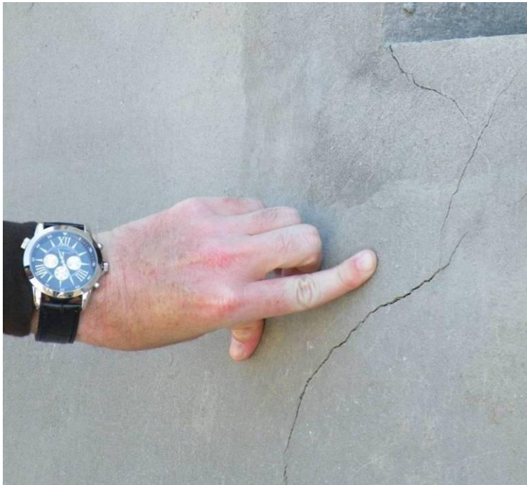
Site Photo 14. Cracking of the surface coating on the block walls and columns
