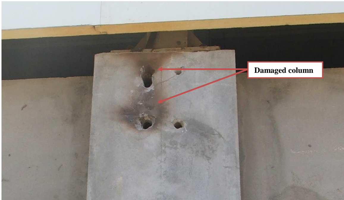
Site Photo 13. Column damage from drilling holes for anchor bolts
