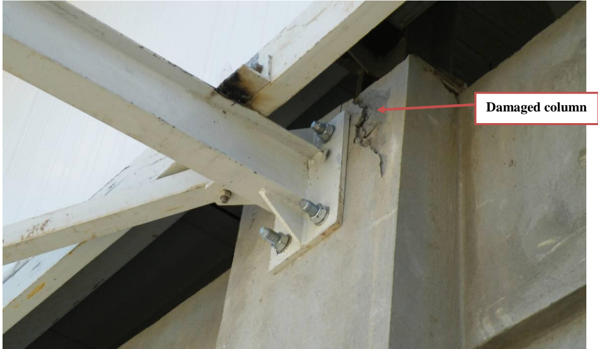
Site Photo 12. Column damage from unsecured anchor bolts
