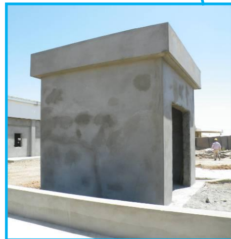
Site Photo 4. Pump room
