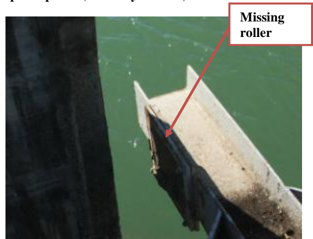
Site Photo 13. Missing rail/roller
