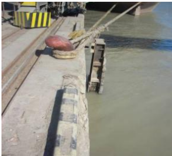
Site Photos 5 and 6. Berth 5 jetty fenders in disrepair (Courtesy of GRS)
