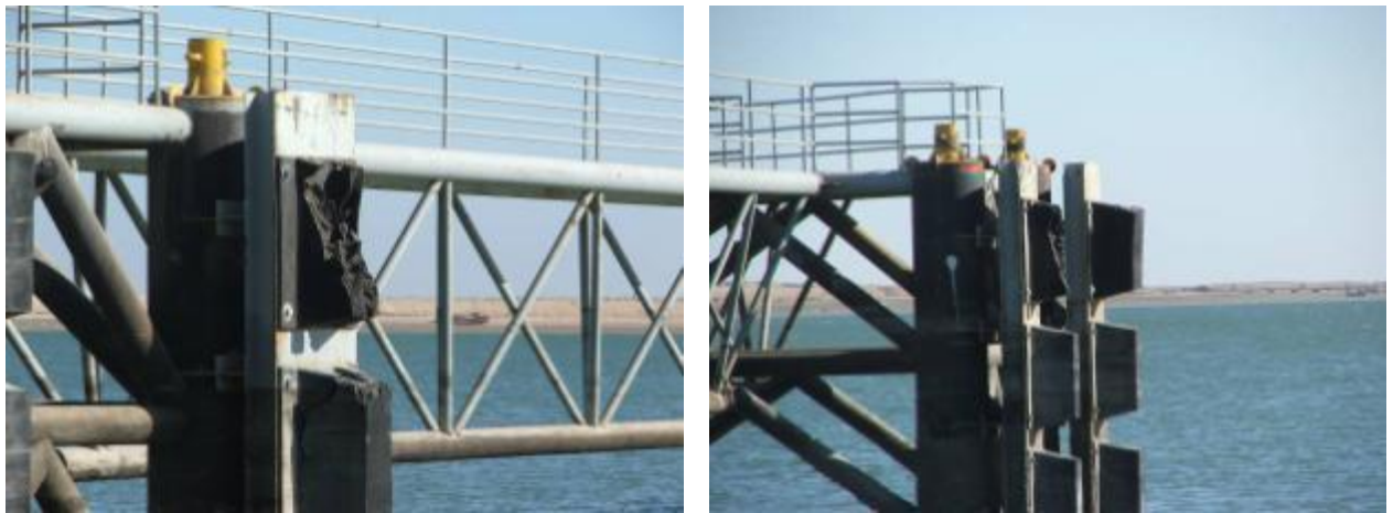
Site Photos 15 and 16. RORO Berth 22 sheared rubber fenders
