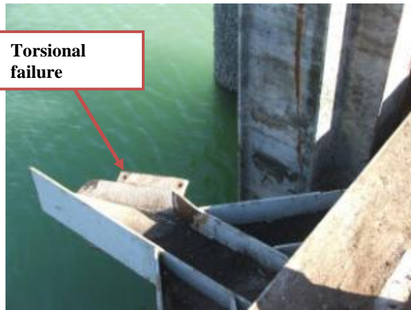
Site Photo 12. Torsional failure of rail/roller
