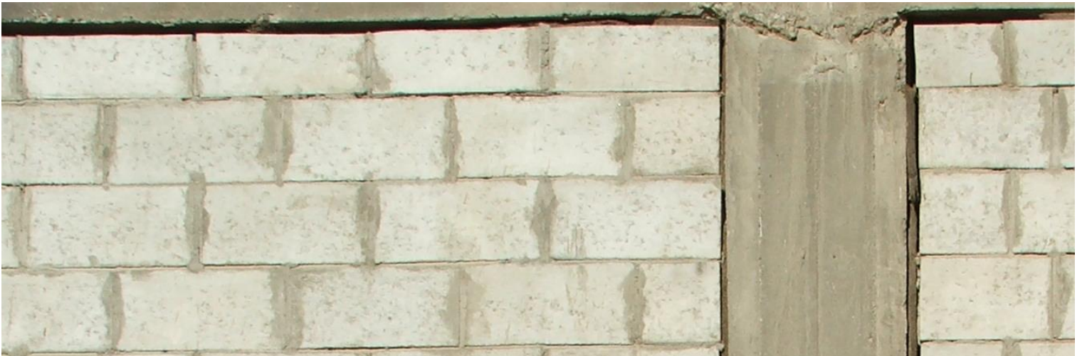
Site Photo 25. Poor block in-fill work
