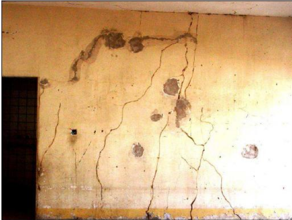
Photo 1. Termite tubes in a concrete structure in Basrah, Iraq (Courtesy of GRS)
