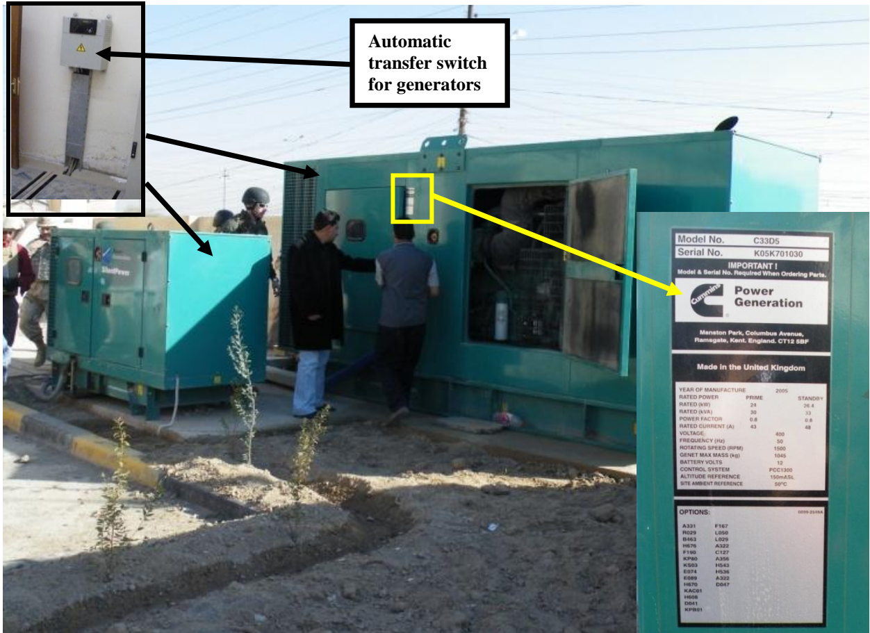
Site Photo 5. Two generators providing primary and emergency backup power for the PHC
