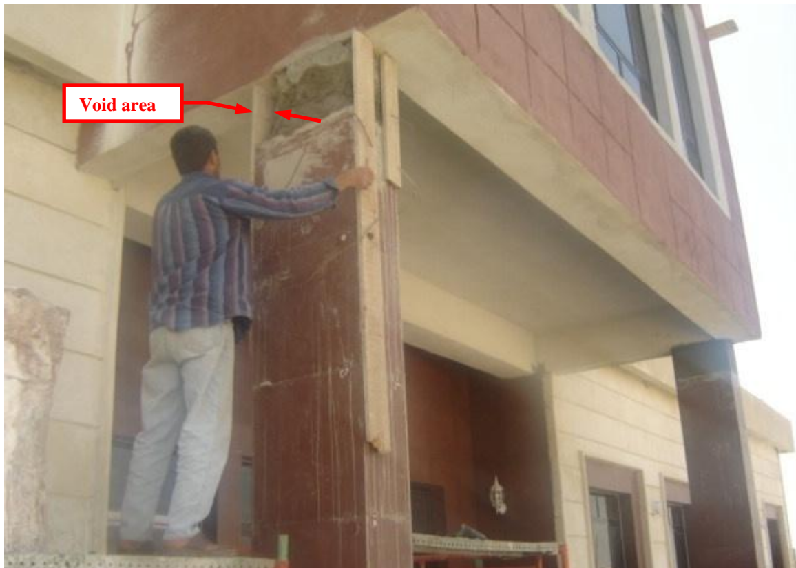
Site Photo 2. Apparent poor quality of beam/column connection (Courtesy of GRN)
