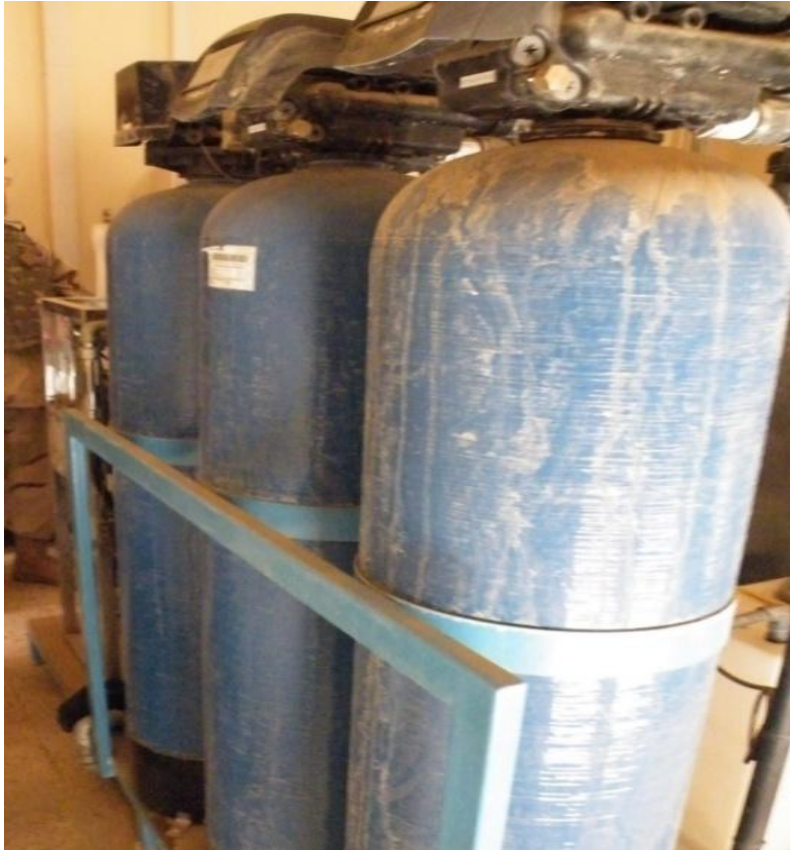
Site Photo 7. Functioning RO unit
