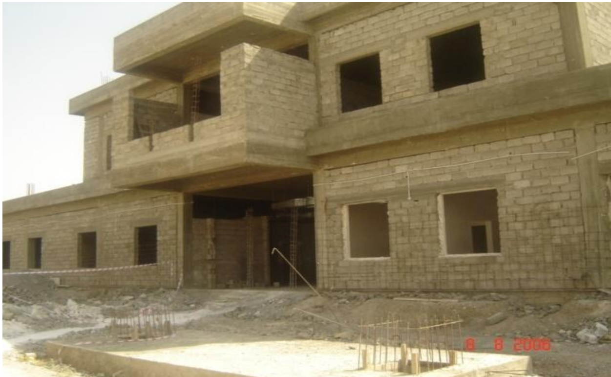
Site Photo 1. Condition of partially constructed PHC when the new contract was awarded (Courtesy of GRN)
