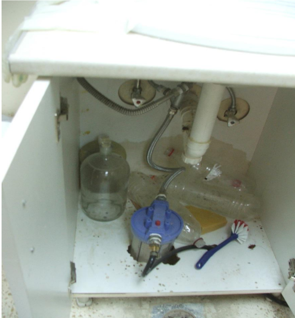
Site Photo 12. Dead insect and debris underneath the sink in the dentist's room
