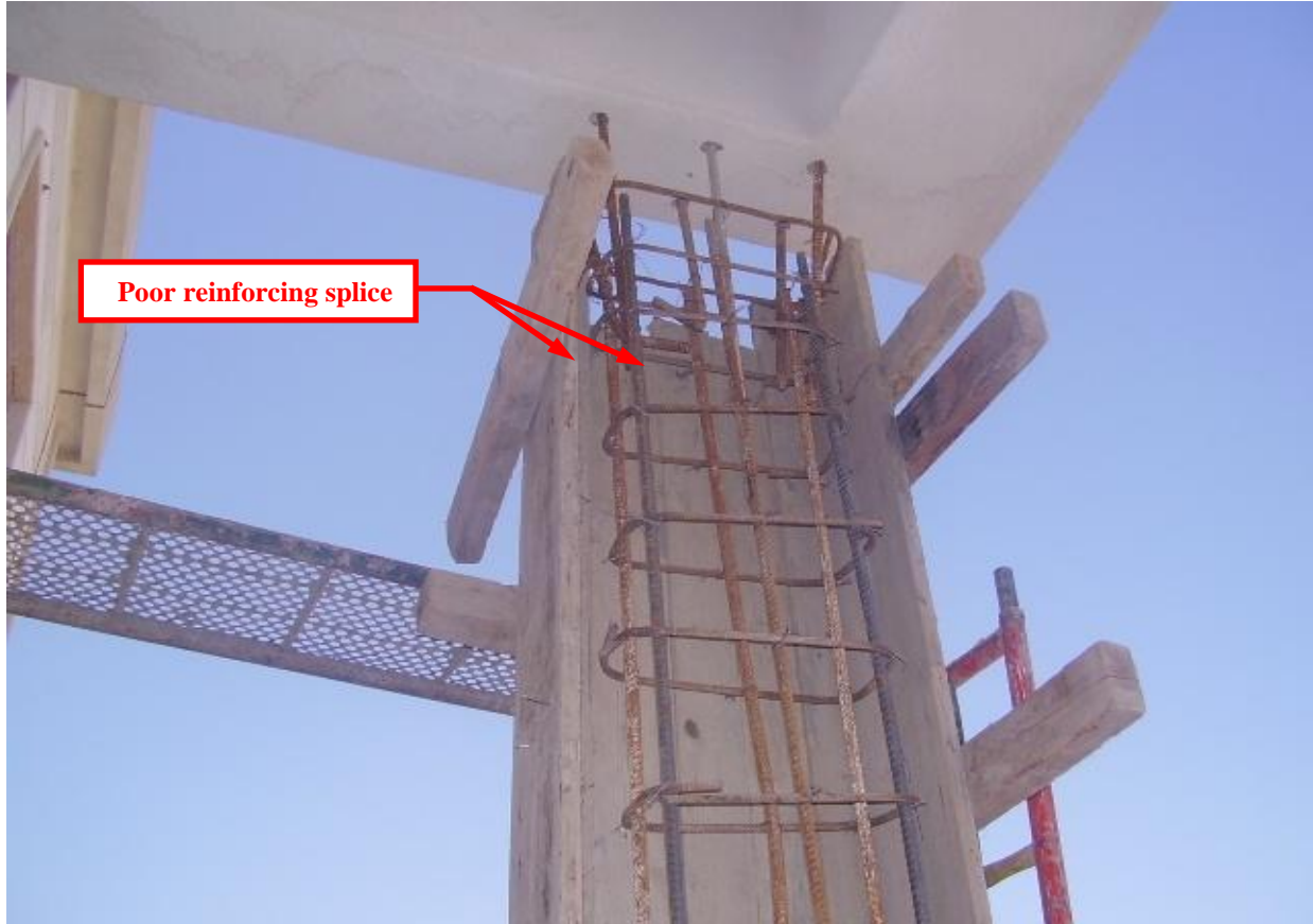
Site Photo 3. Poor quality reinforcing splice (Courtesy of GRN)
