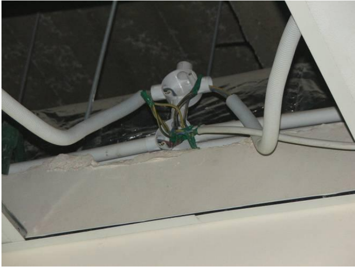
Site Photo 15. Poor electrical connection
