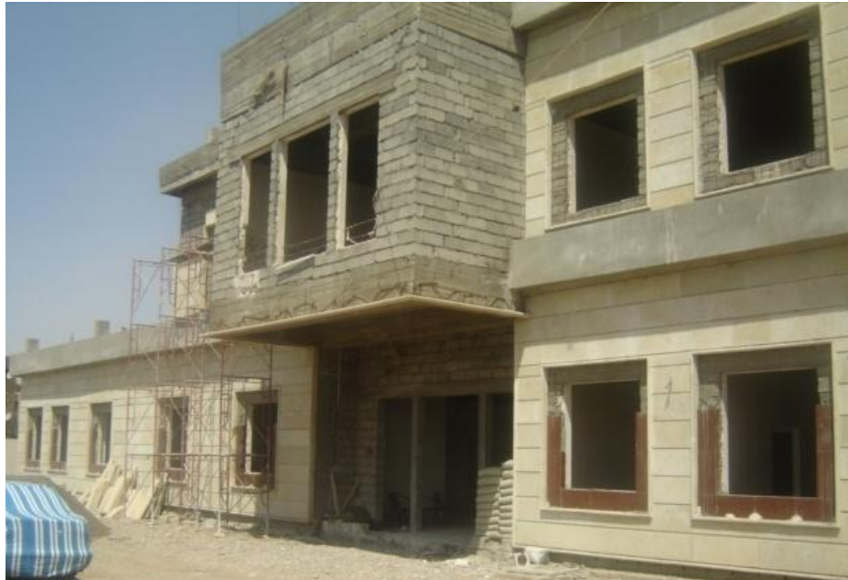
Site Photo 1. Condition of partially constructed PHC when new contract was awarded (Courtesy of GRN)
