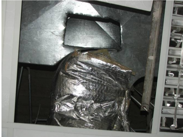
Site Photo 14. Modified HVAC duct
