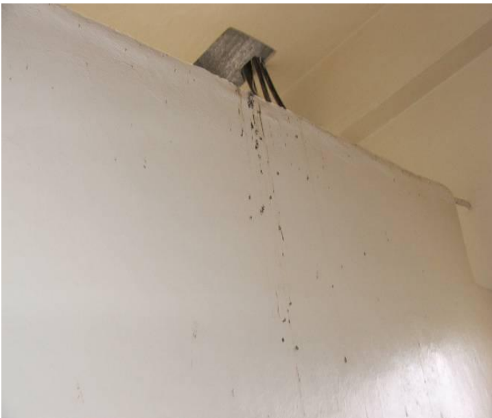
Site Photo 6. Possible water contamination source
