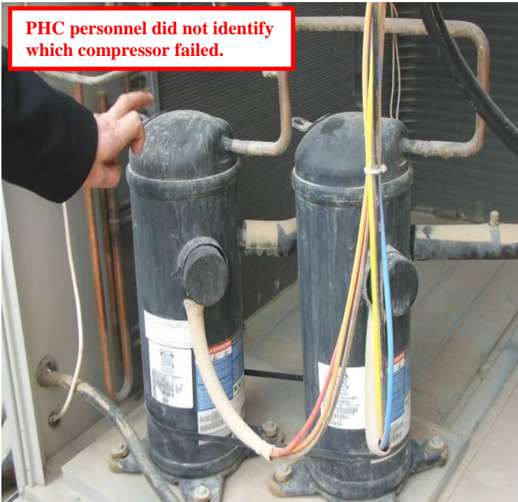
Site Photo 12. Failed HVAC compressor
