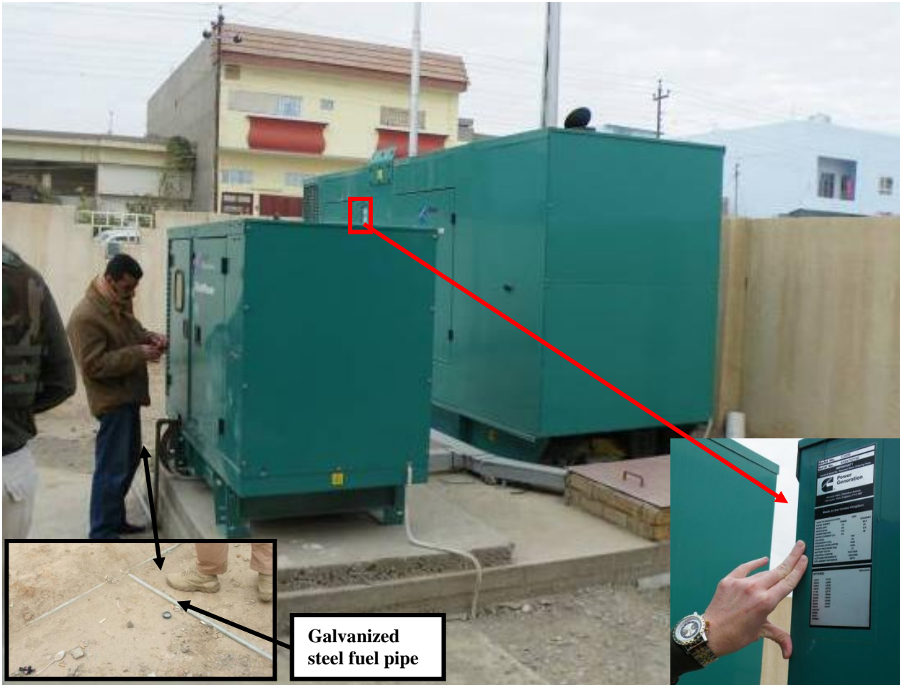
Site Photo 4. Two generators providing primary and emergency backup power for the PHC
