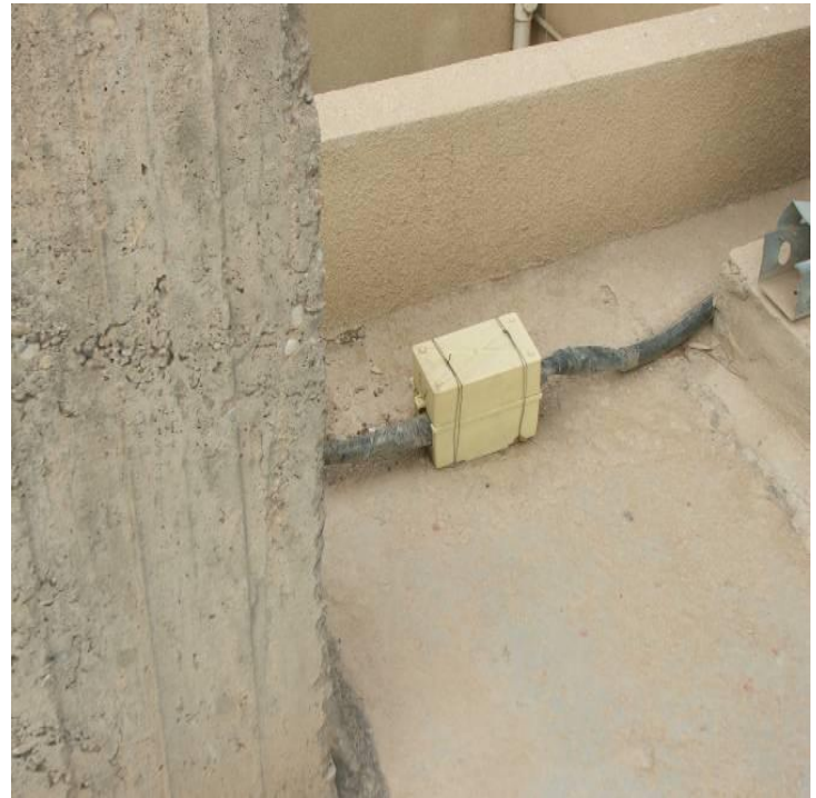
Site Photo 13. Makeshift electrical junction
