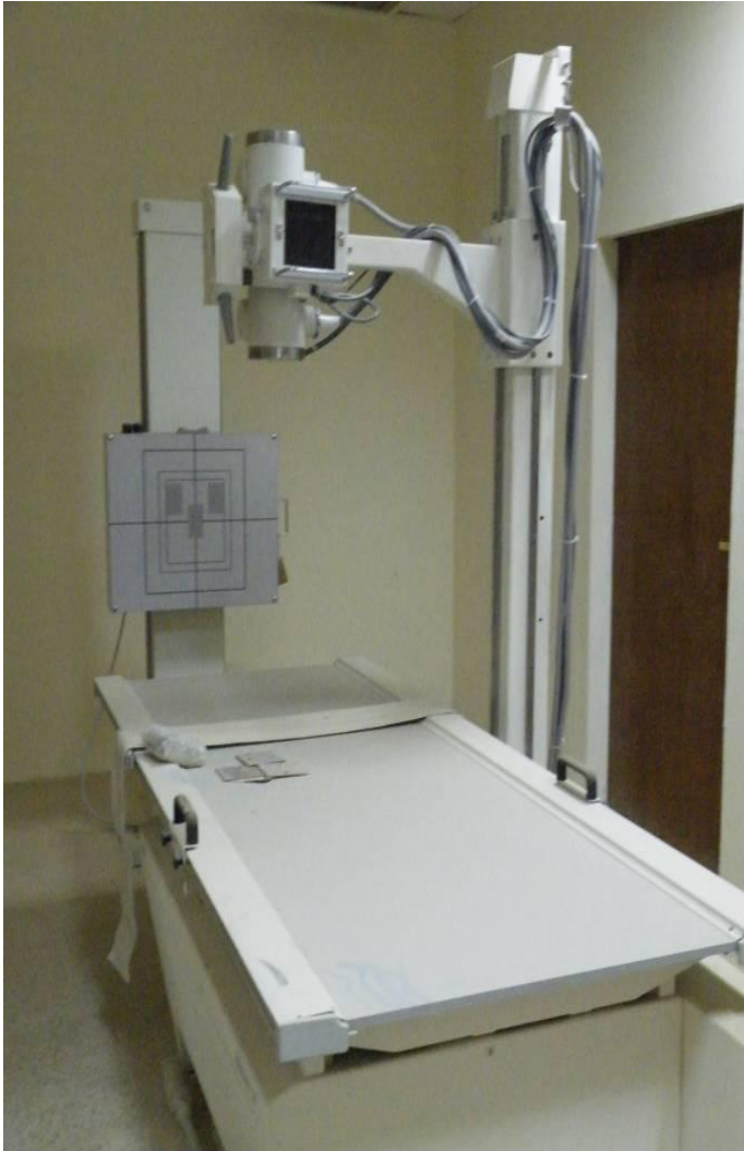
Site Photo 10. X-ray equipment
