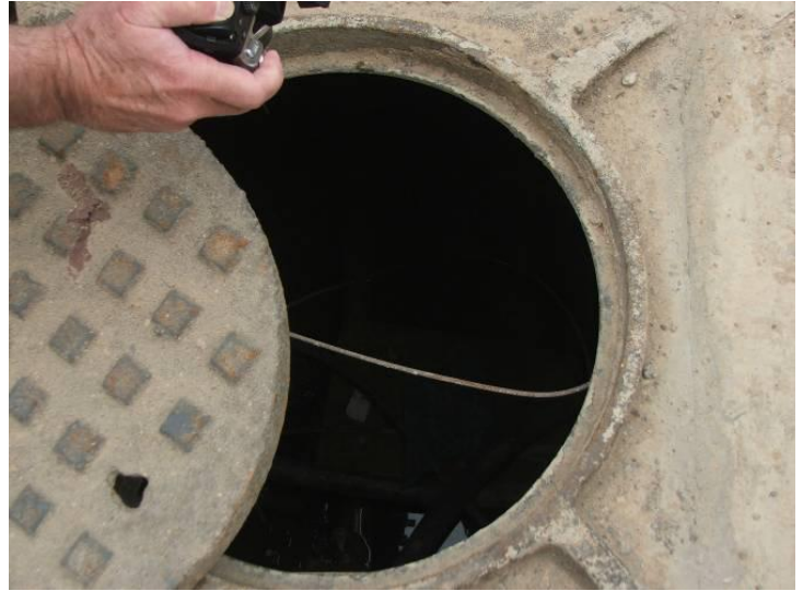
Site Photo 16. Debris and water in electric manhole
