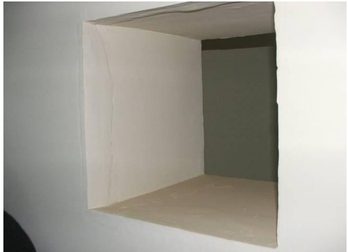
Site Photo 11. Missing observation window
