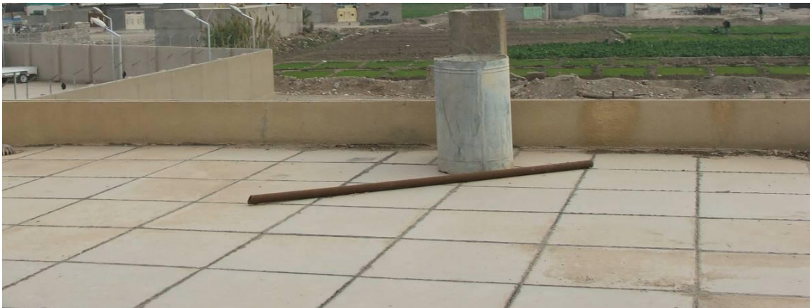
Site Photo 17. Quality of roof construction
