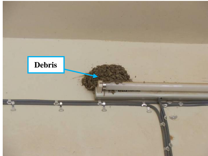
Site Photo 9. Debris on light fixture
