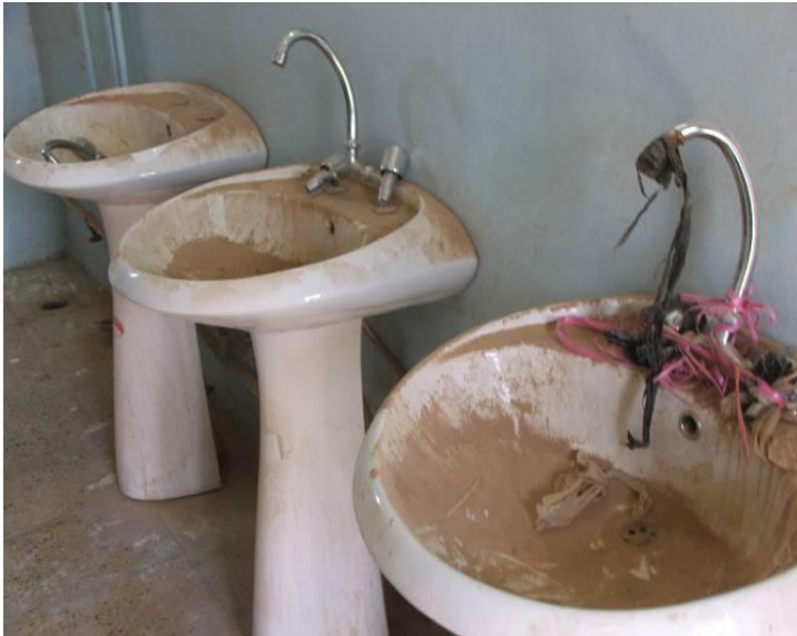
Site Photo 13. Damaged lavatories
