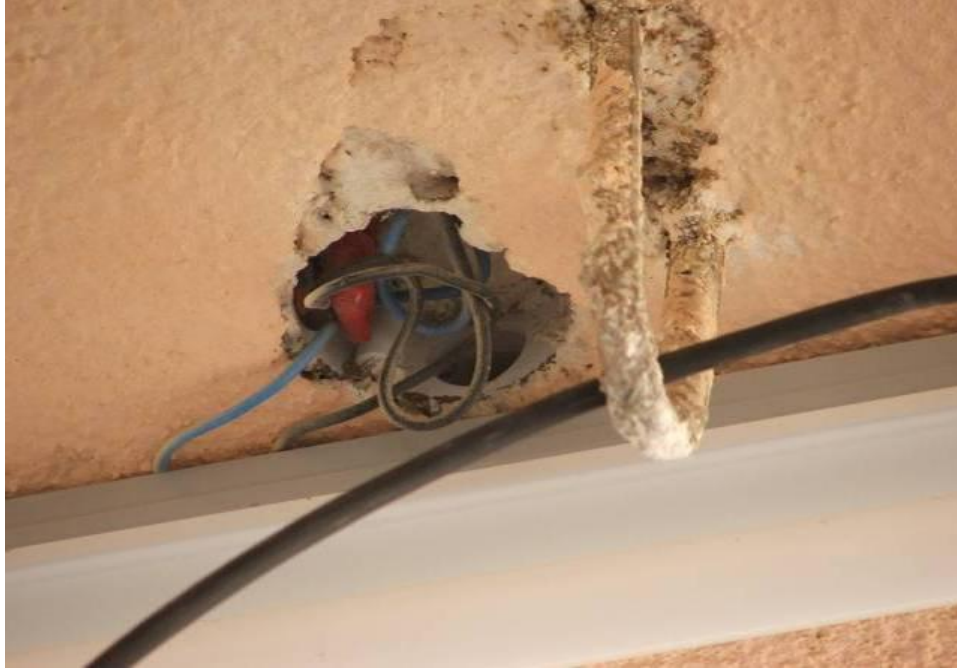
Site Photo 11. Example of deficient and potentially hazardous electrical connections
