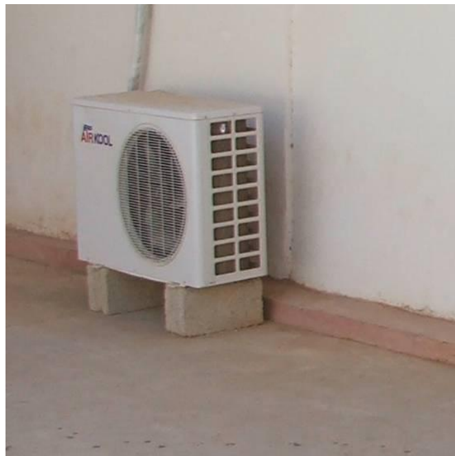
Site Photo 10. Split air-conditioning unit
