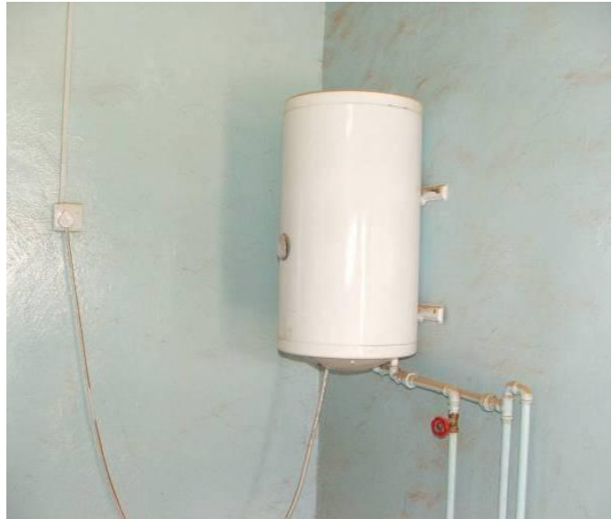
Site Photo 14. Hot water heater
