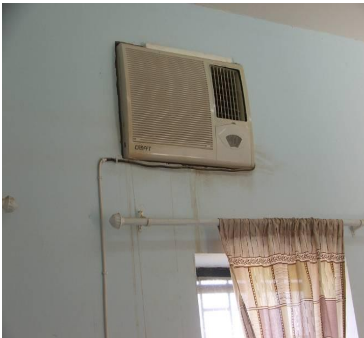
Site Photo 9. Wall mounted air-conditioning unit
