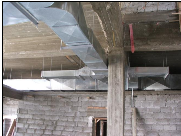
Poor concrete work and ductwork at the Hai Alasra Wa Al Mafqoodeen Primary Health Care Center
