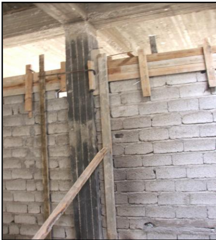
Ongoing construction work at the Shiqaq Hai Musalla Primary Health Care Center
