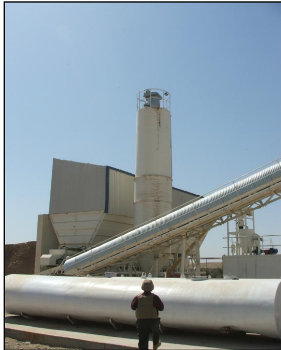
SIGIR Inspector at the grout mixing plant at the Mosul Dam
