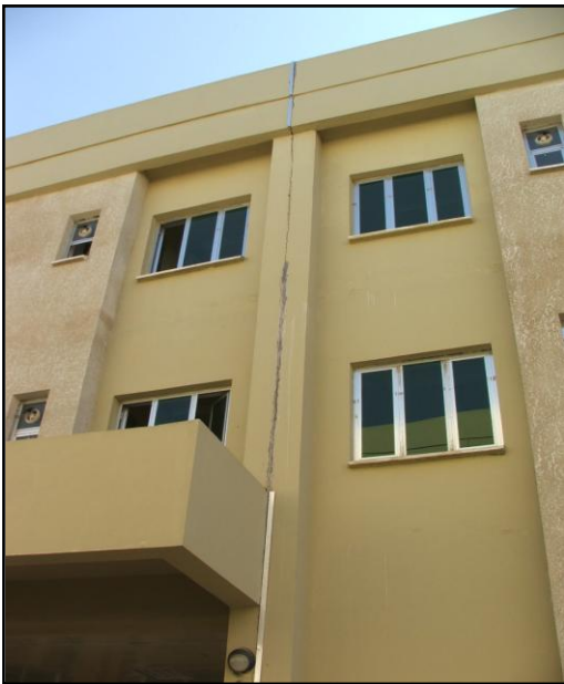
Large settlement crack running down the Baghdad Police College building
