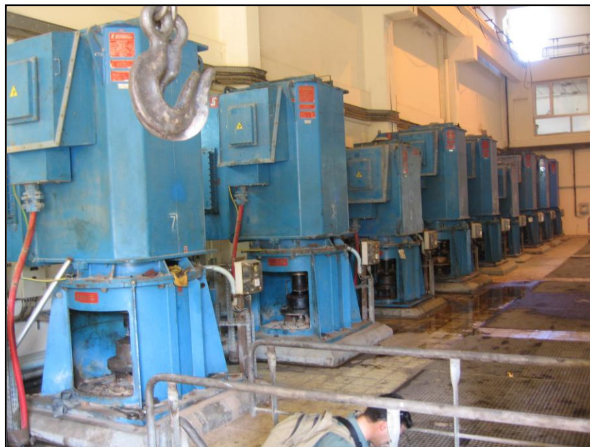
Sadr City Al Qana'at water pumping station
