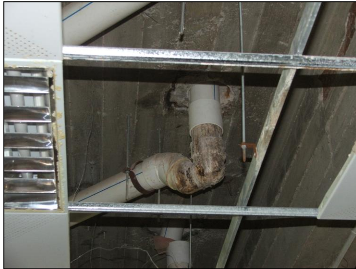
Inferior craftsmanship with plumbing installation
