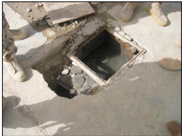
Tallil Military Base-broken drain cleanout hole
