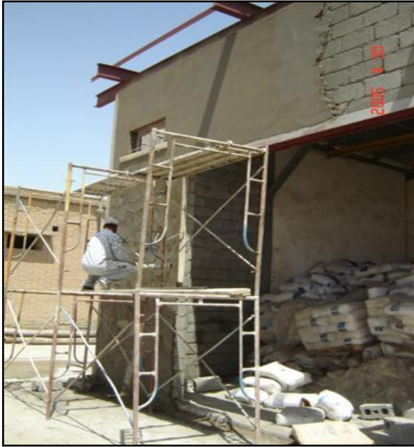
Construction work on the new chemical building at Al Wahda Water Treatment Plant
