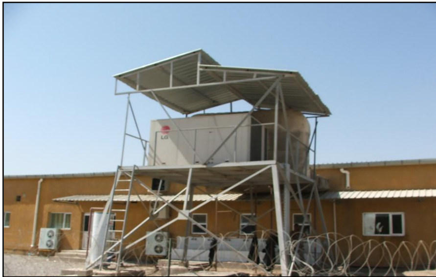
Generator located at the Al Rasheed Brigade Set
