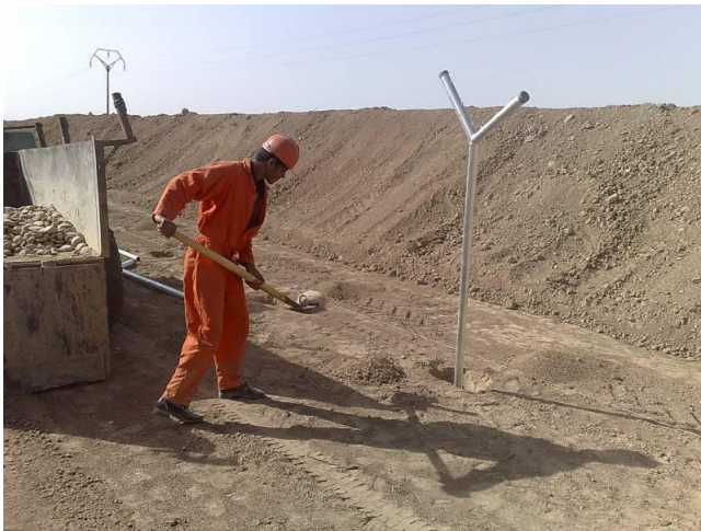
Site Photo 5. Installing posts for the PEZ fence post (Photo courtesy of the USACE)
