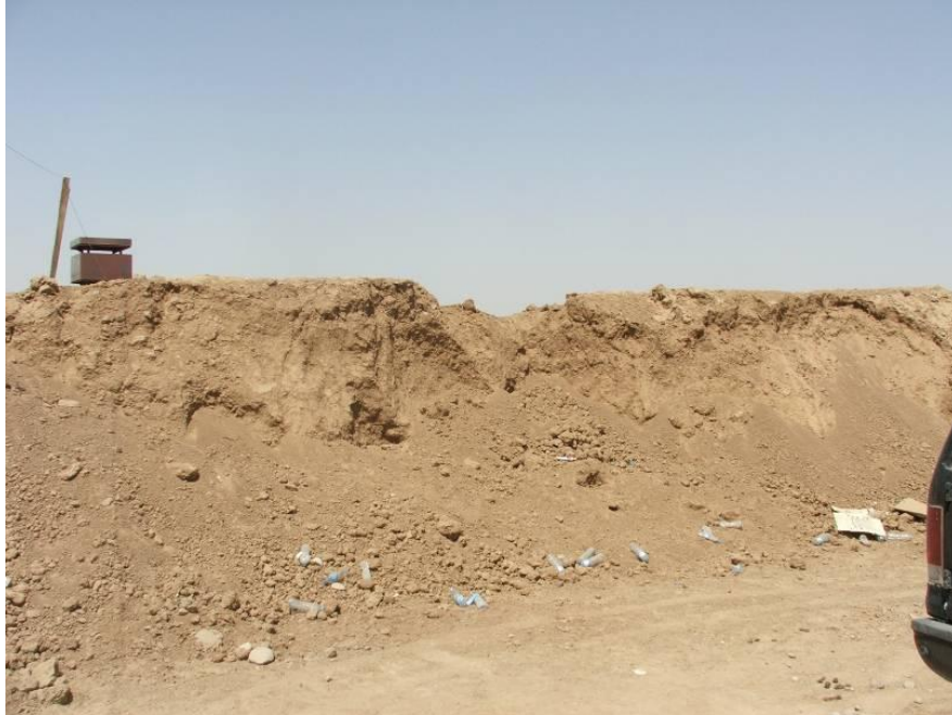
Site Photo 12. Example of earthen berm compaction degradation
