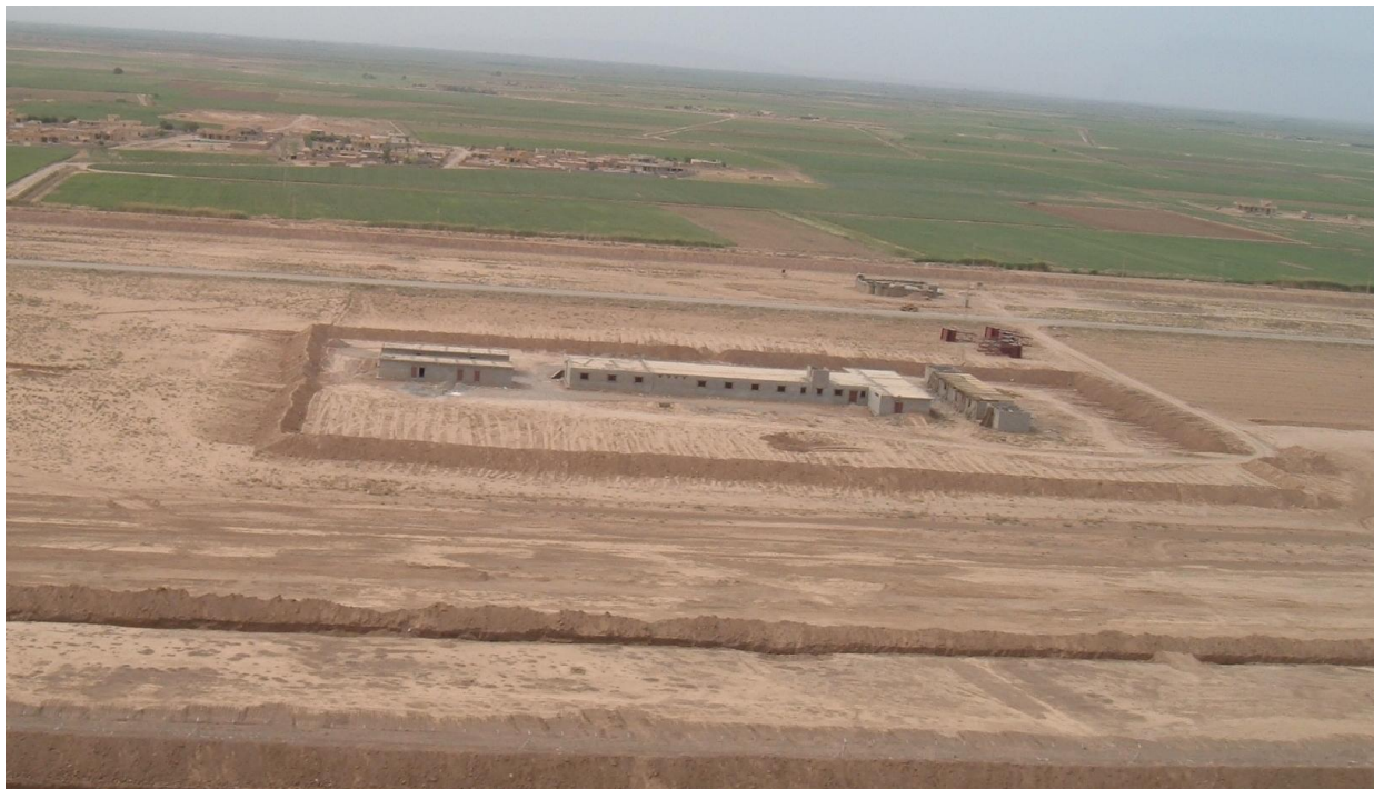
Site Photo 27. Aerial view of a partially constructed battalion headquarters facility (Photo courtesy of the USACE)
