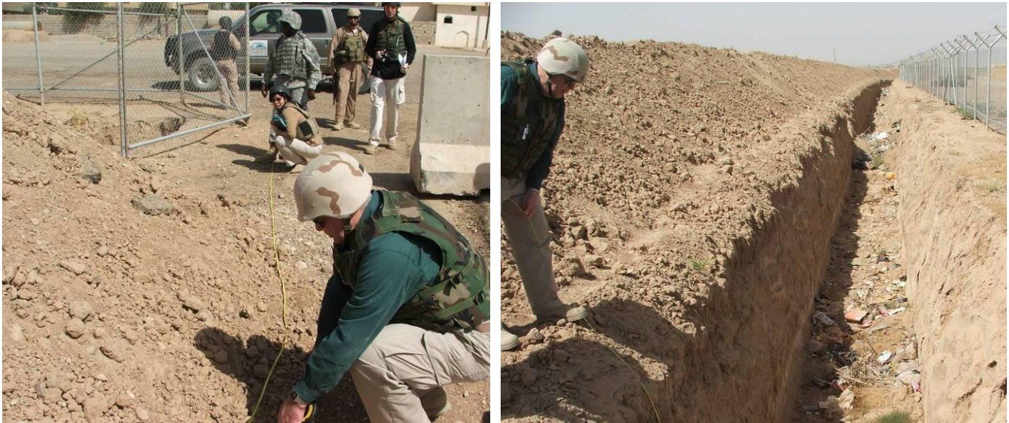
Site Photos 10 and 11. SIGIR inspectors ensuring the ditch and berm met contract design specifications
