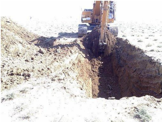
Site Photo 3. Excavation for the PEZ ditch (Photo courtesy of the USACE)
