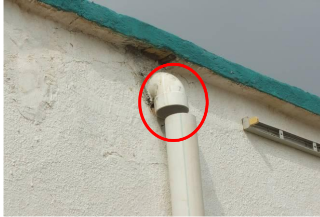
Site Photo 5. Loose connection
