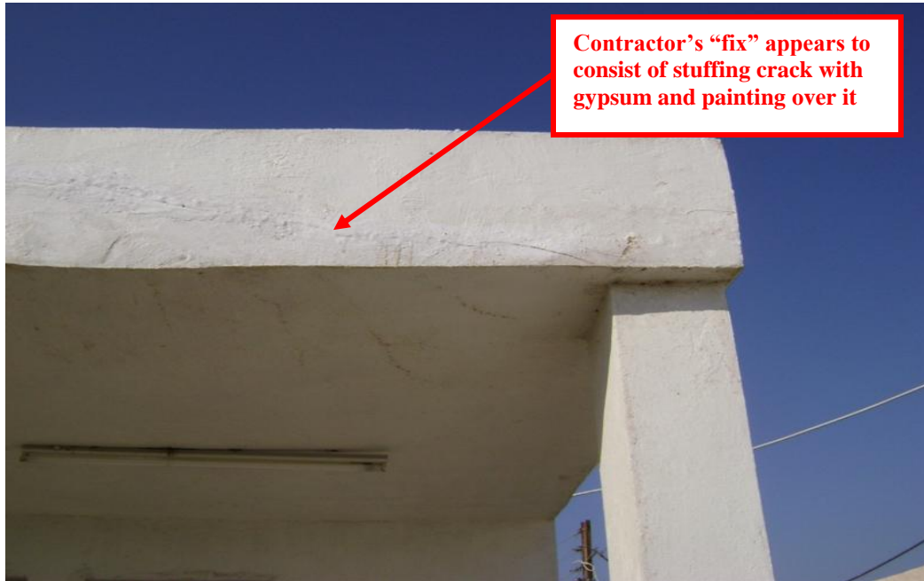
Site Photo 13. Contractor's fix for the reinforcement beam crack (Courtesy of GRC)
