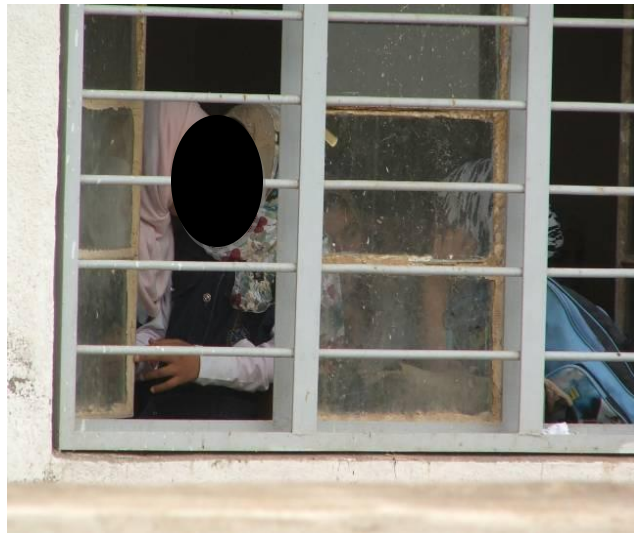
Site Photo 6. Missing window screen
