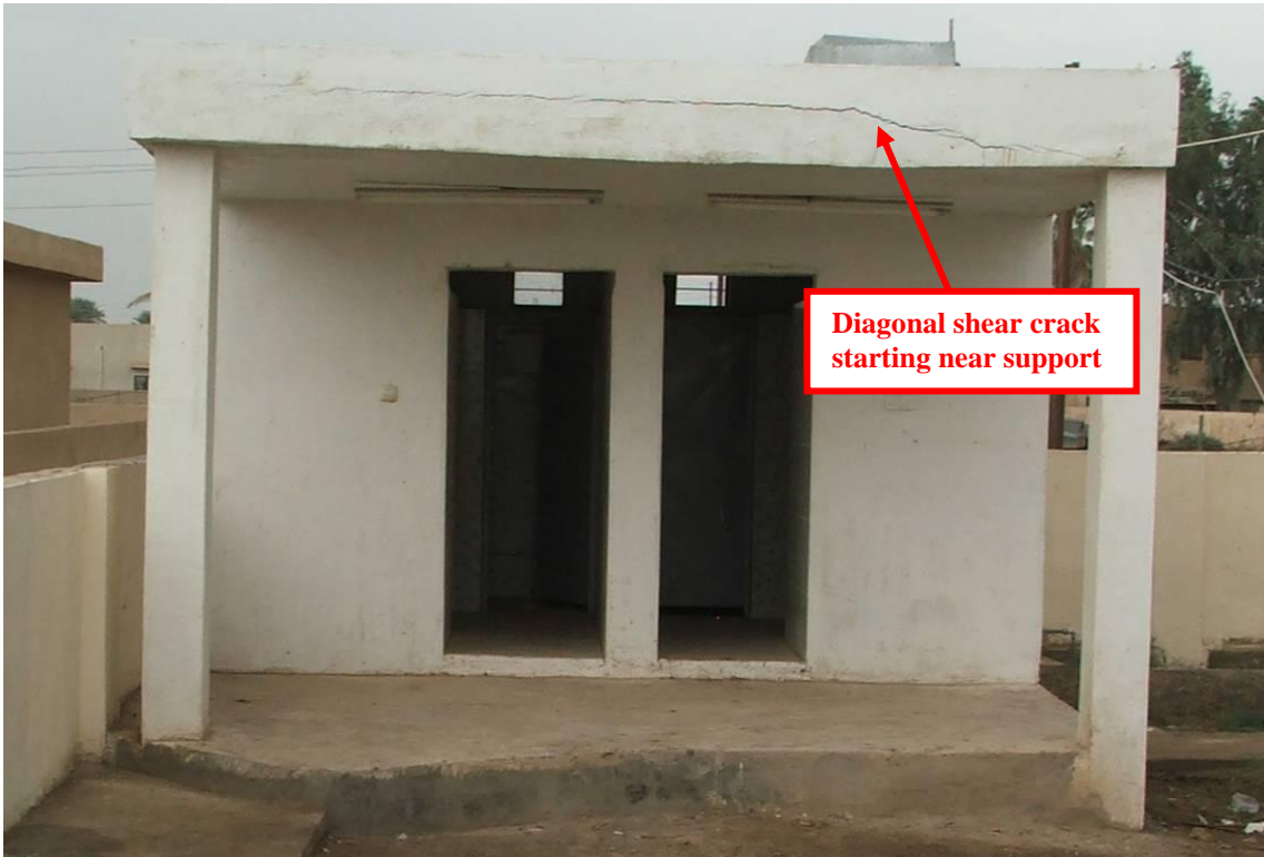
Site Photo 8. New latrine building with significant shear crack
