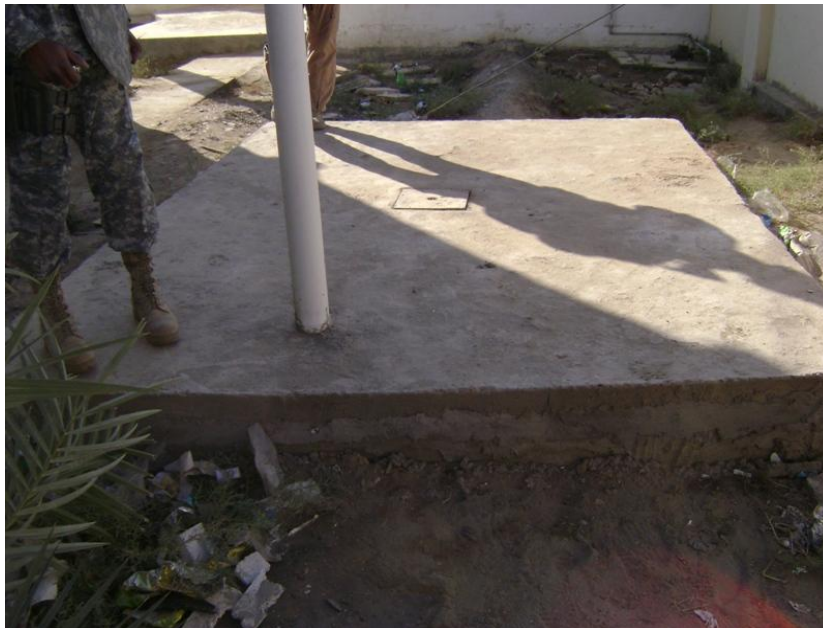
Site Photo 14. Newly installed access hatch for the sewage tank (Courtesy of GRC)
