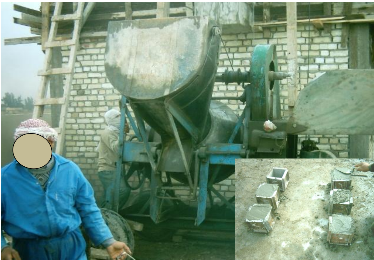
Site Photo 2. Site-mixed concrete and concrete test cubes (lower right corner) (Courtesy of GRC)
