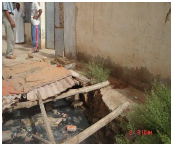
Site Photo 1. Open septic tank (Courtesy of GRC)
