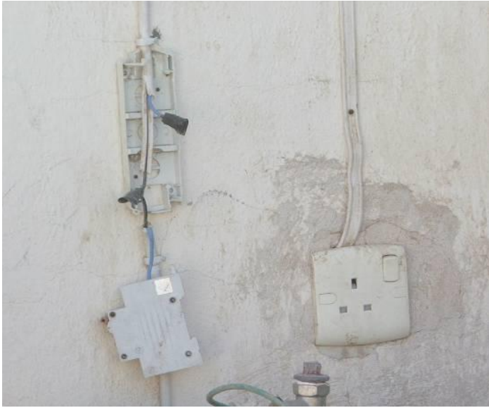
Site Photo 7. Unsafe electrical wiring and breaker
