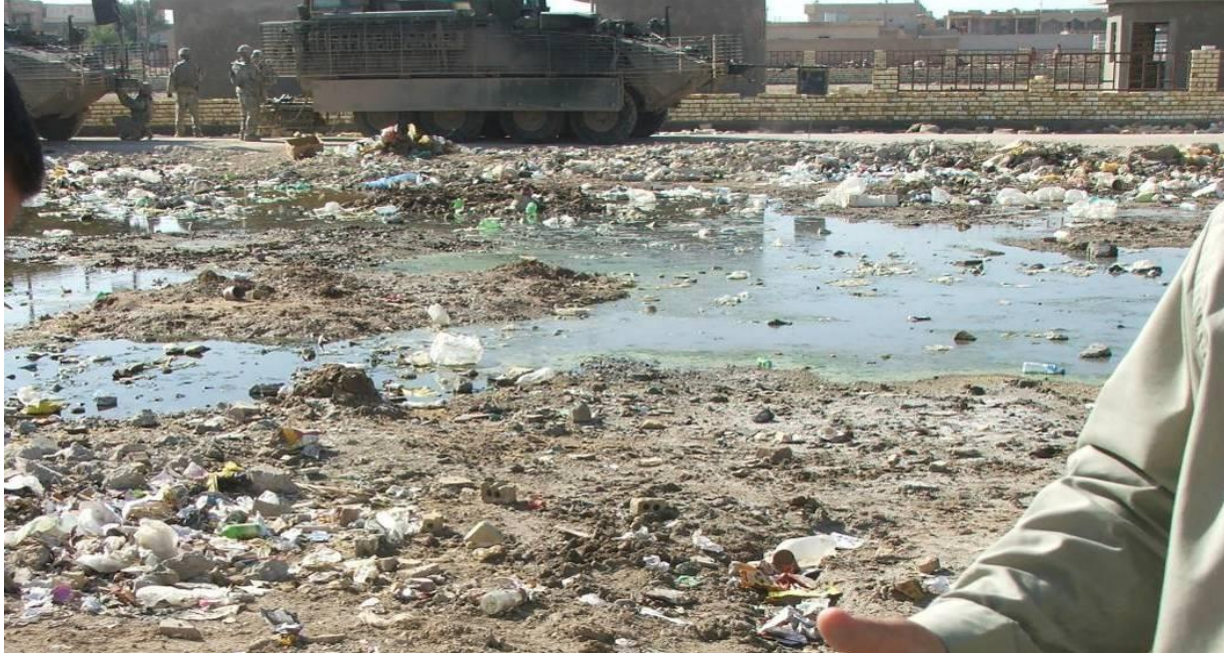
Site Photo 14. Trench dug to allow discharge out of the full septic tank
