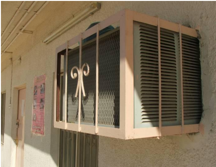
Site Photo 9. The only window air conditioner observed at the school
