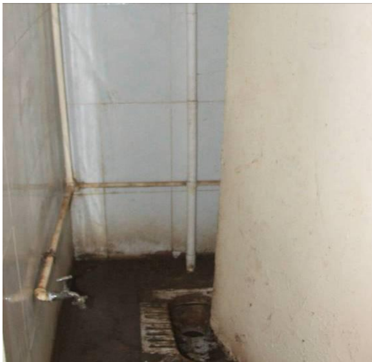
Site Photo 13. Unsanitary condition of school bathrooms
