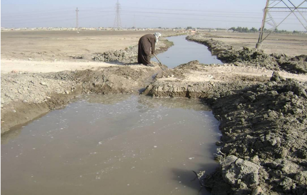
Site Photo 14. No pipe culvert on service road (Courtesy of the USACE))
