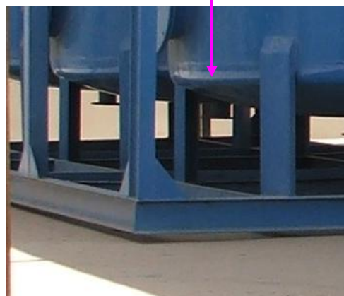
Site Photo 14. Equipment not bolted to slab.
