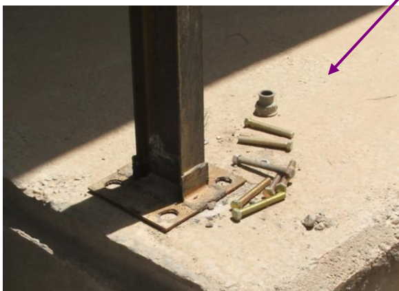
Site Photo 13. Unbolted sunshade post
