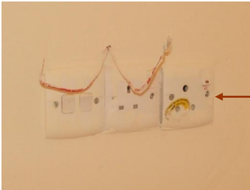
Site Photo 9. Inadequate electrical work
