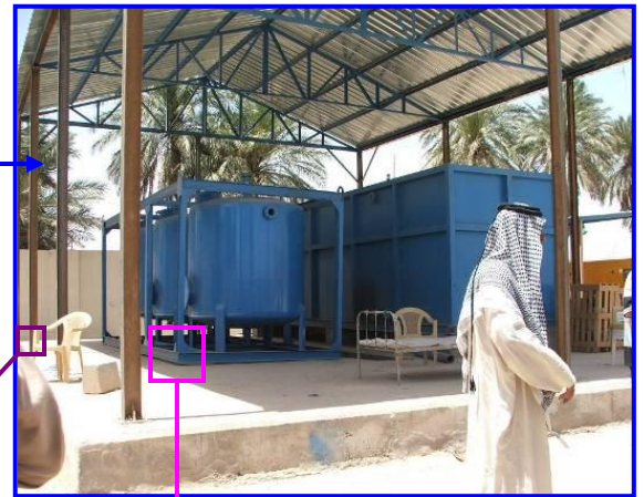
Site Photo 12. Water compact unit sunshade
