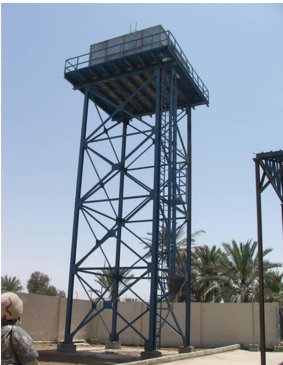
Site Photo 6. Elevated reservoir storage.
