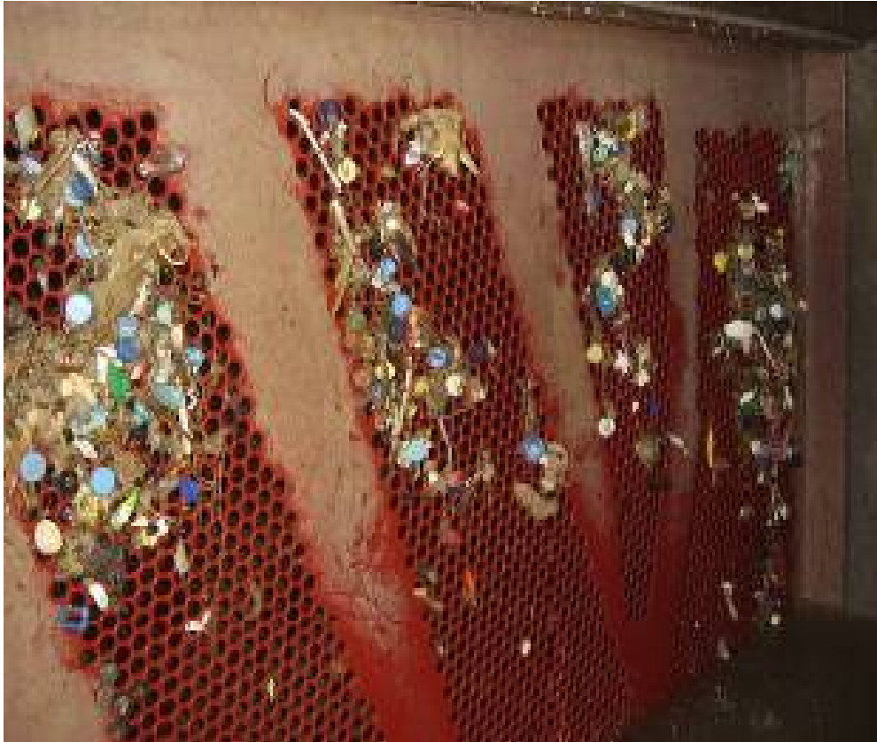
Site Photo 1. Condenser clogged with debris (Photo courtesy of GRD Electricity Sector)
