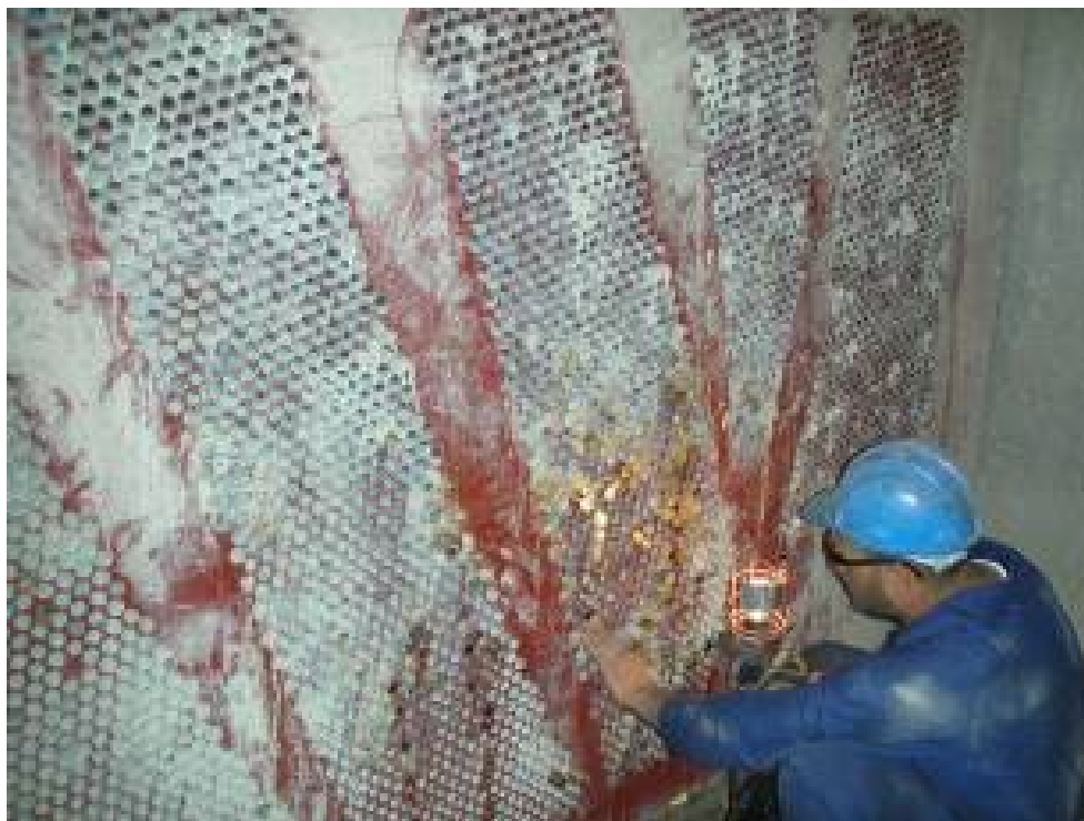
Site Photo 2. Condenser cleaning and repair. (Photo courtesy of GRD Electricity Sector)
