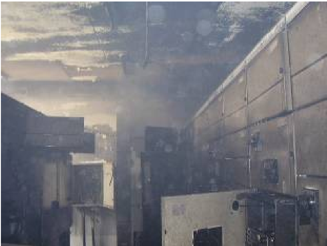
Site Photo 5. Oil Station control center after May 2007 fire. (Photo courtesy of Electricity Sector)
