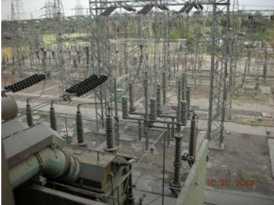
Site Photo 7. Unit 5 transformer and 132 kV switchyard is in questionable condition. (Photo courtesy of Electricity Sector)
