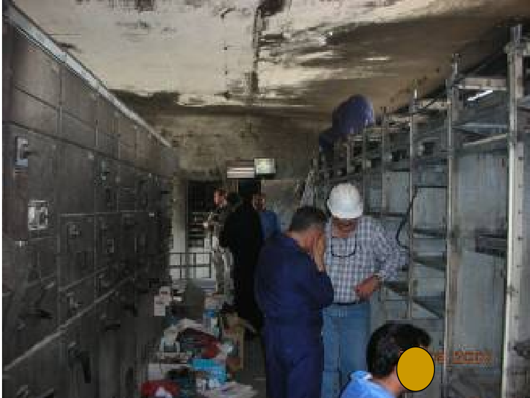
Site Photo 6. Control center cleanup and repair work in progress. (Photo courtesy of Electricity Sector)
