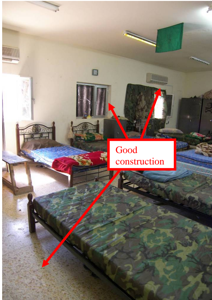
SIGIR Site Photo 2. Barracks residential area without noticeable construction or maintenance deficiencies.
