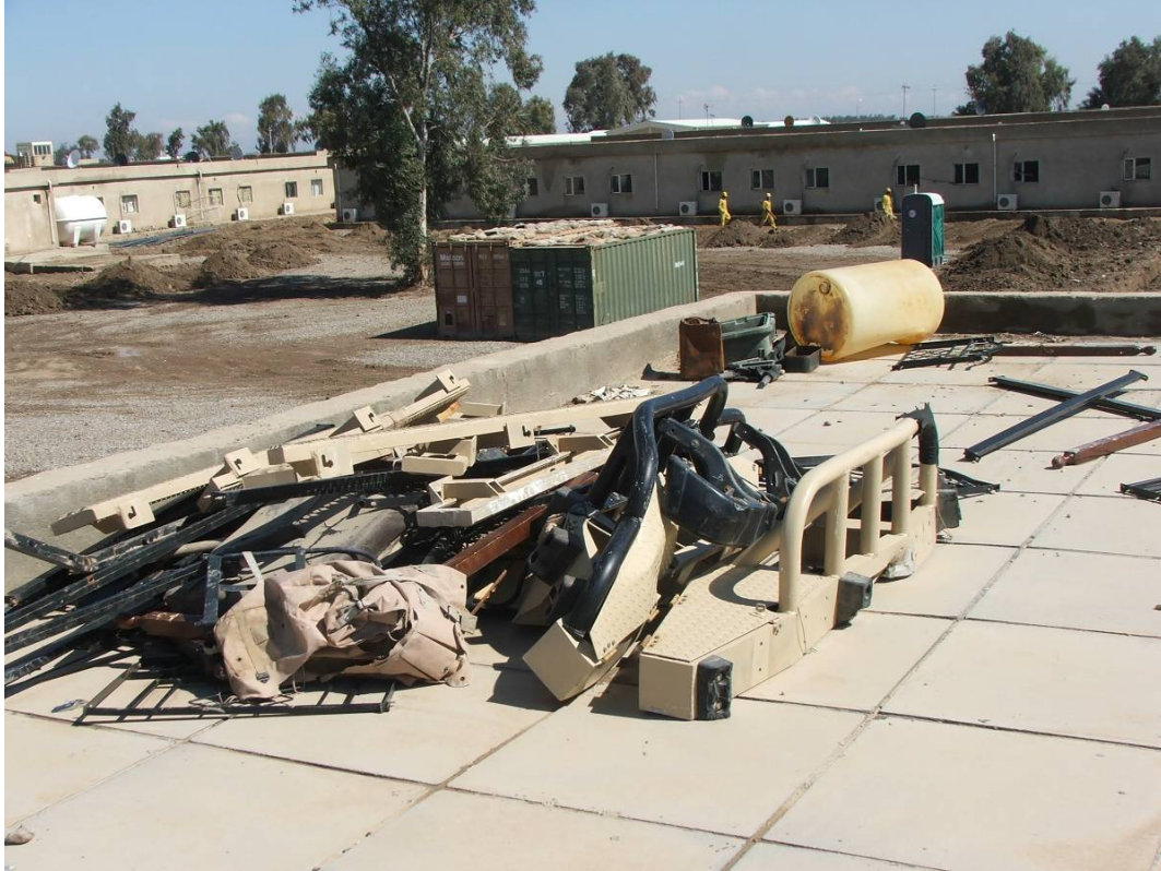
Site Photo 12. Old vehicle components, bed frames and other items were placed on the barracks' roof.
