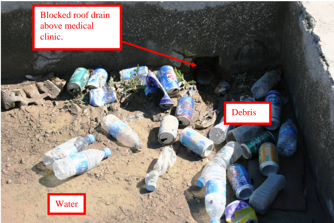
Site Photo 15. Roof drain blocked above clinic.
