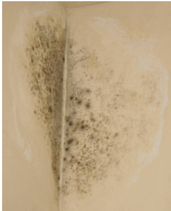
Site Photo 16. Water stain and biological growth in a barracks clinic.
