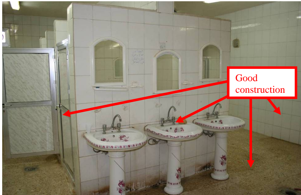
SIGIR Site Photo 3. Senior barracks bathroom with working sinks, showers, toilets and drains.
