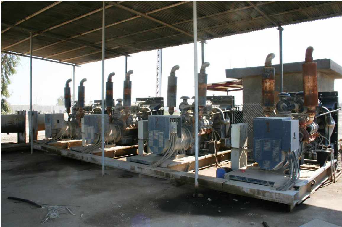
Site Photo 10. Four generators installed but not operational during site visits.
