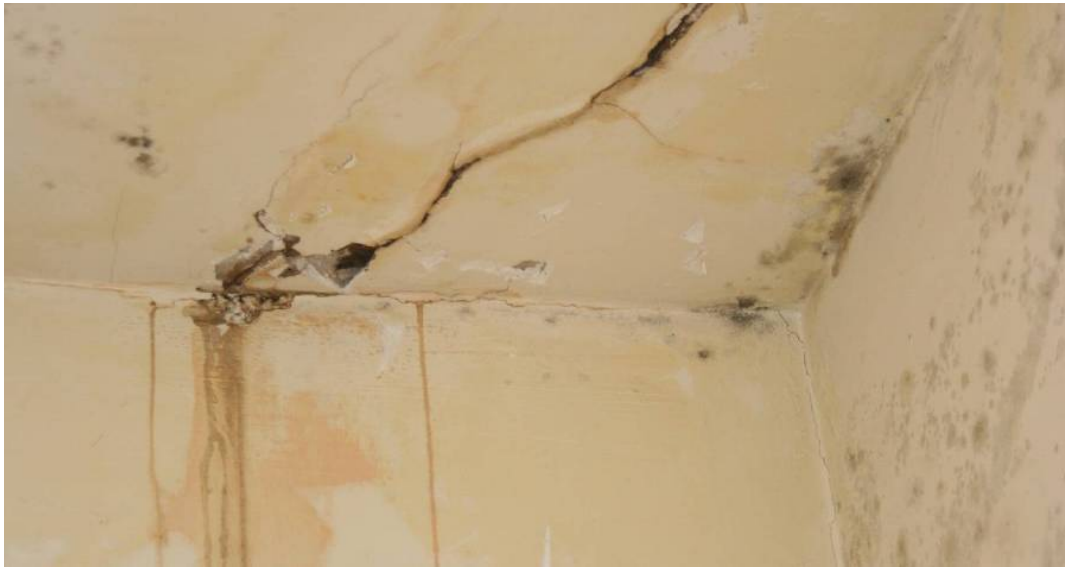
Site Photo 17. Evidence of water problem inside the senior barracks.
