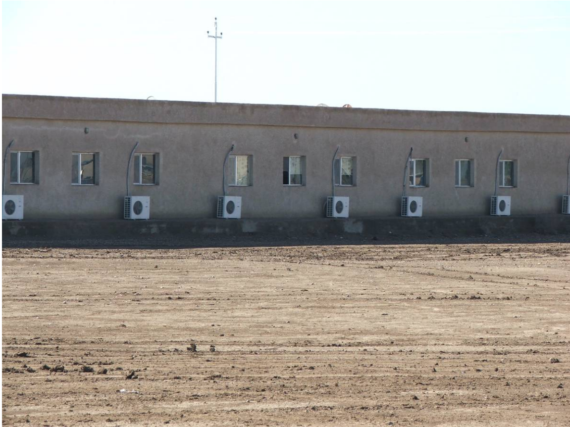
Site Photo 1. Barracks exterior appeared to be in good condition and did not show signs of settling or other major construction problems.
