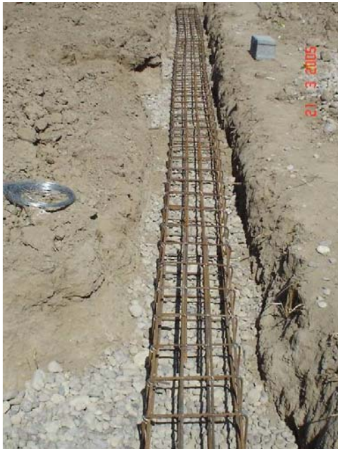
USACE Construction Progress Photo 2. Sub-foundation rock and tied rebar were properly placed.
