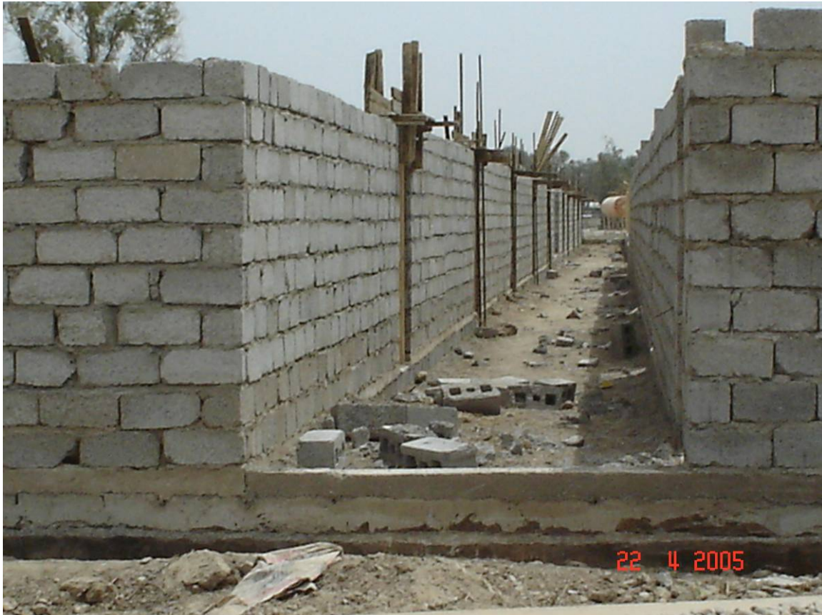
USACE Construction Progress Photo 4. Concrete blocks were used to make load bearing walls.
