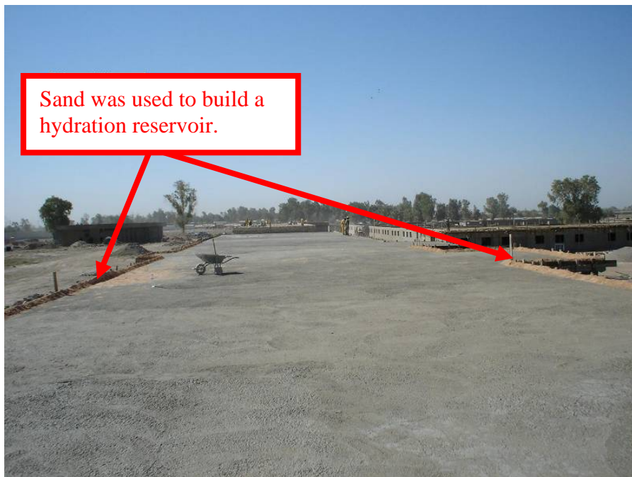
USACE Construction Progress Photo 6. Each Company Barracks roof was over 14,000 sq. ft.
