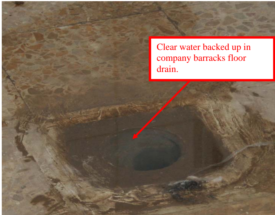
Site Photo 6. Clear water backed up in floor drain of company barracks.
