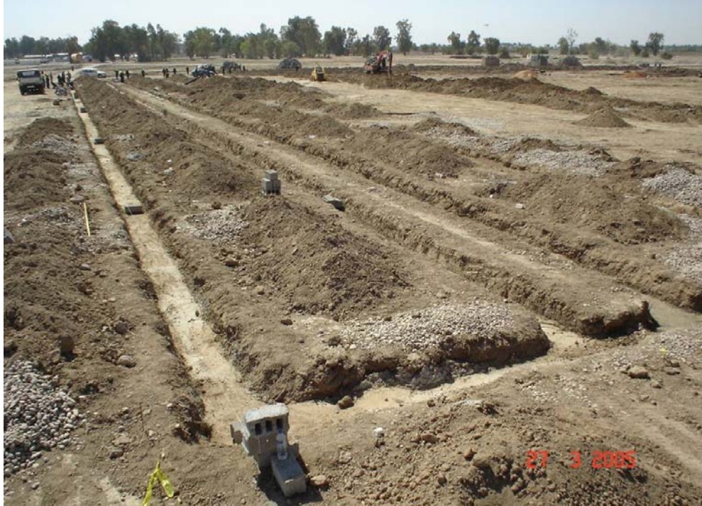
USACE Construction Progress Photo 1. Before construction, the level and accessible site was cleared.
