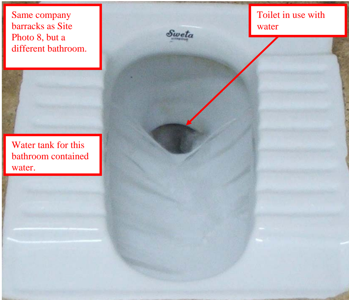
Site Photo 9. Toilet in use with water in the company barracks.
