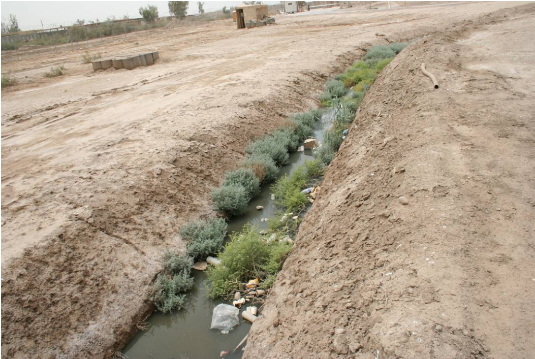
Site Photo 15. Raw sewage is pumped from sewage holding tanks into storm water runoff ditch
