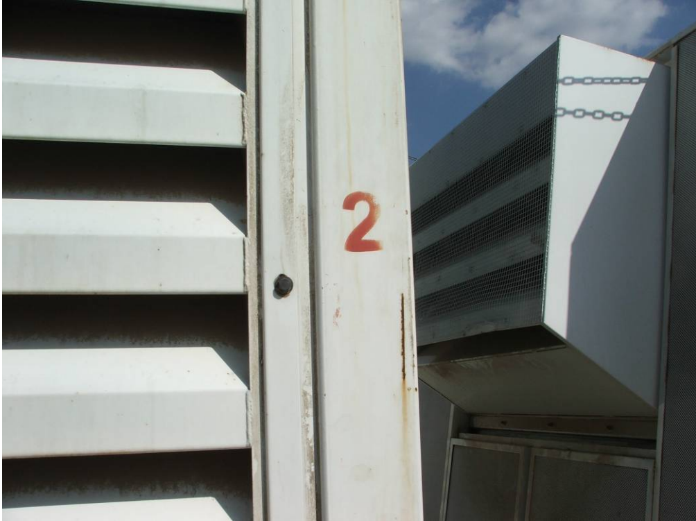
Site Photo 20. Cummins generator set 2
