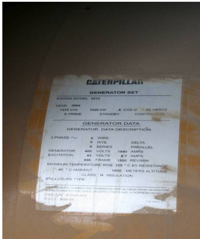
Site Photo 39. Caterpillar generator set 3 ID plate
