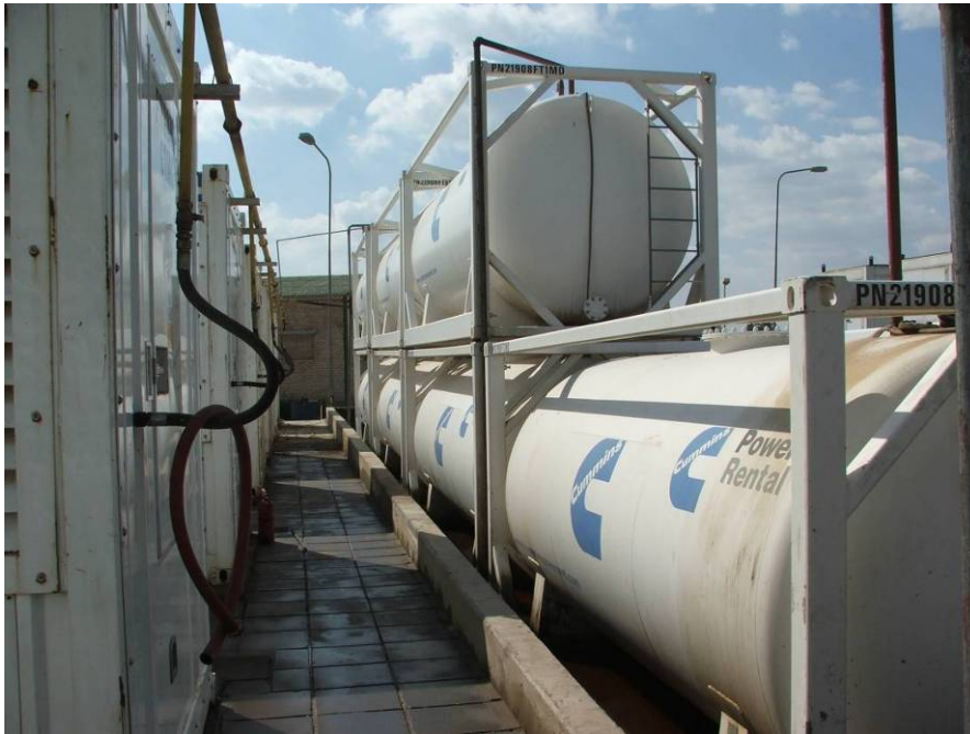
Site Photo 32. Cummins generator sets' fuel tanks
