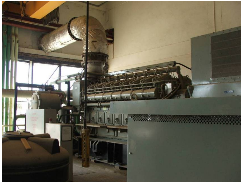
Site Photo 11. General Electric generator
