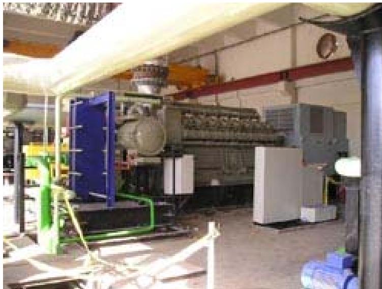
Site Photo 3. GE generator (Photo provided by USAID)
