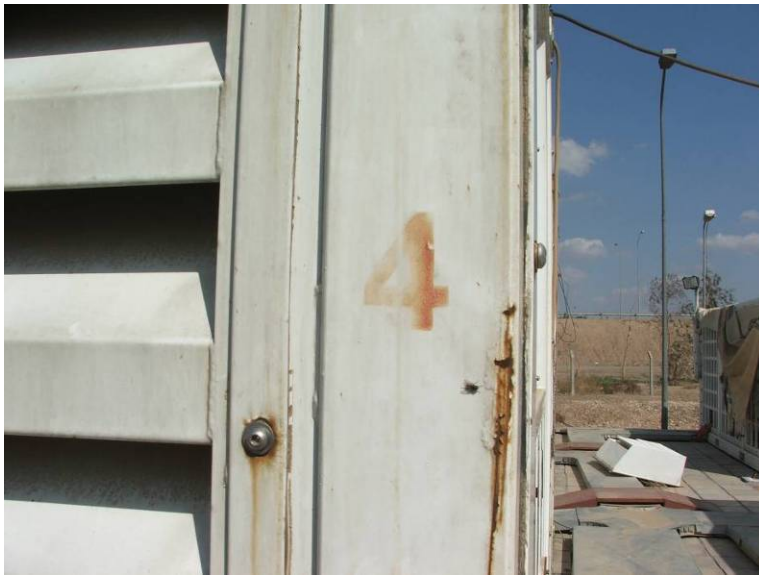
Site Photo 24. Cummins generator set 4
