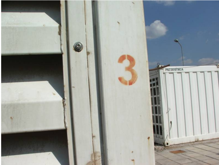
Site Photo 22. Cummins generator set 3
