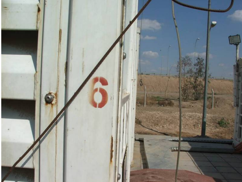
Site Photo 28. Cummins generator set 6
