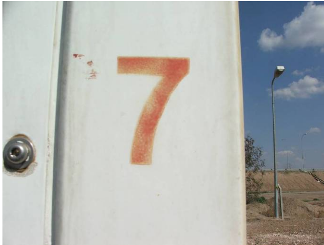
Site Photo 30. Cummins generator set 7
