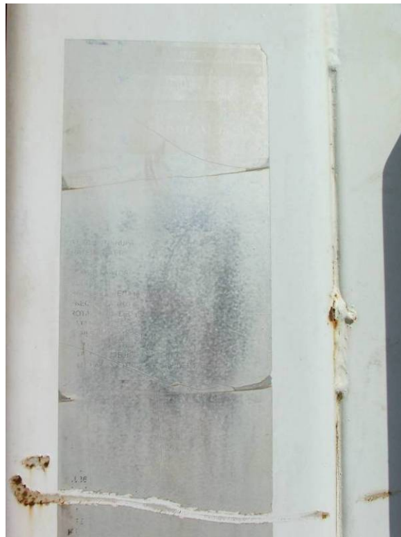
Site Photo 19. Cummins generator set 1 ID plate faded from direct sunlight
