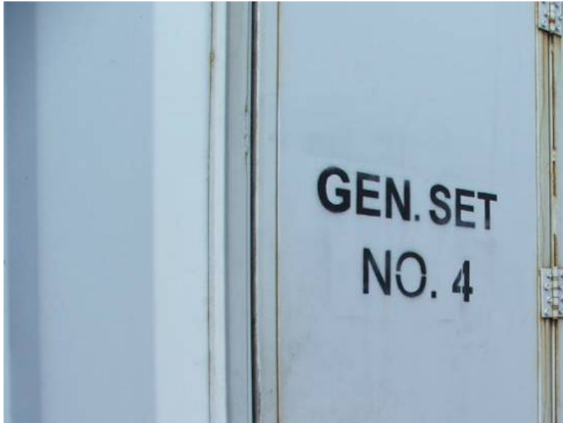
Site Photo 40. Caterpillar generator set 4
