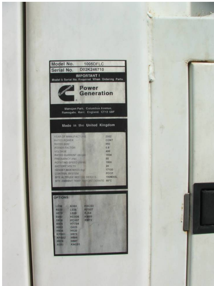
Site Photo 29. Cummins generator set 6 ID plate
