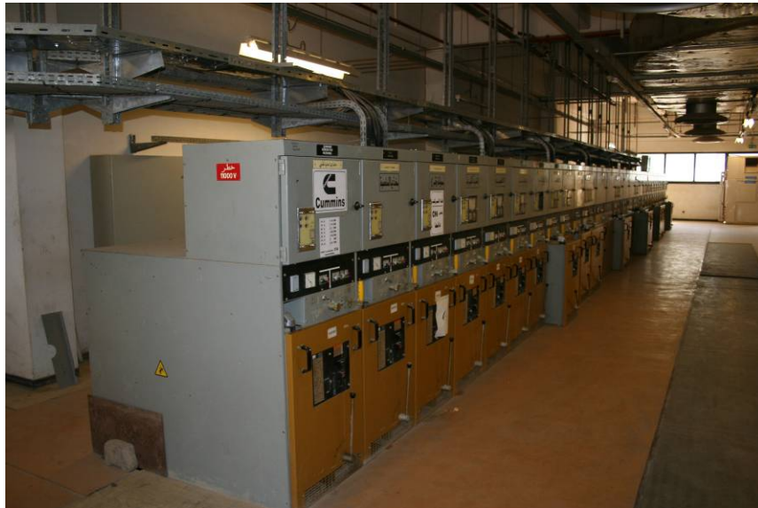
Site Photo 48. System for Cummins generator sets
