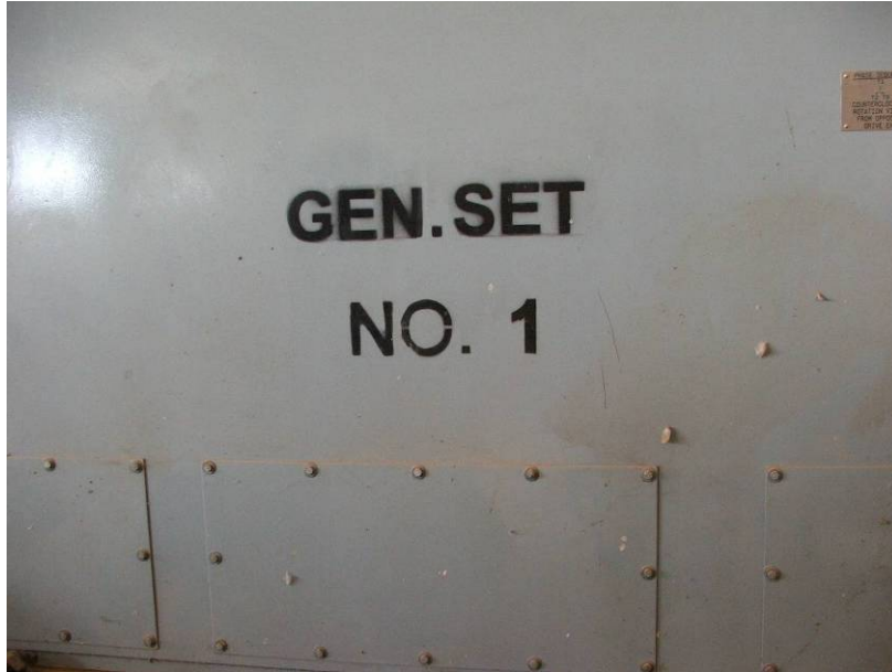
Site Photo 12. General Electric generator set 1
