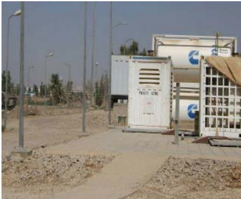
Site Photo 5. Cummins generator sets (Photo provided by USAID)
