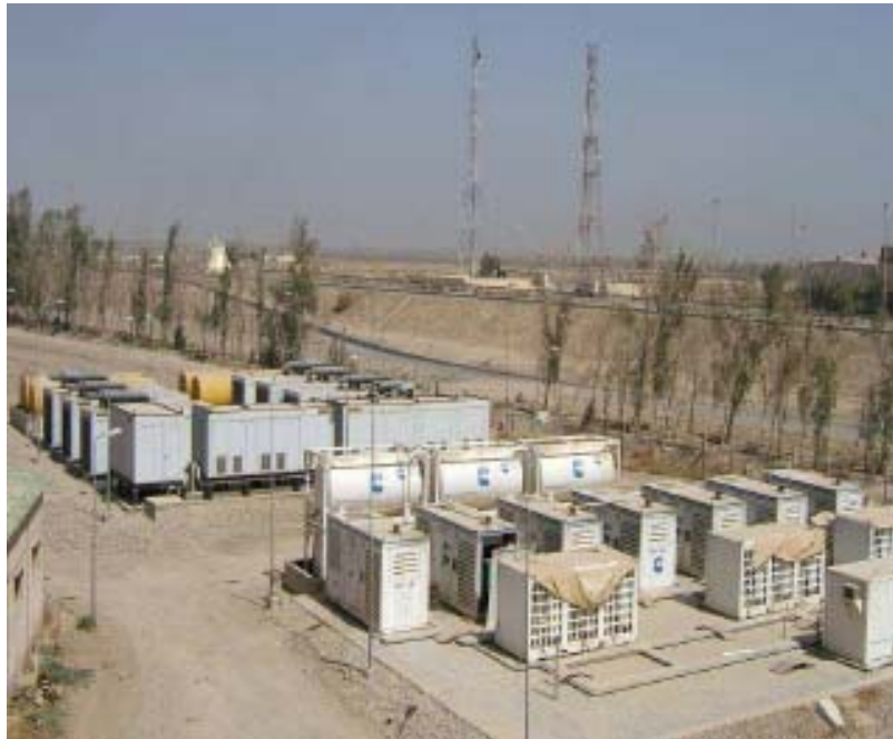
Site Photo 4. Seven Cummins generators (Photo provided by USAID)
