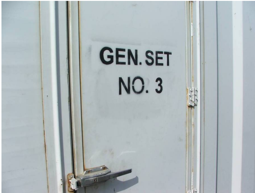
Site Photo 38. Caterpillar generator set 3
