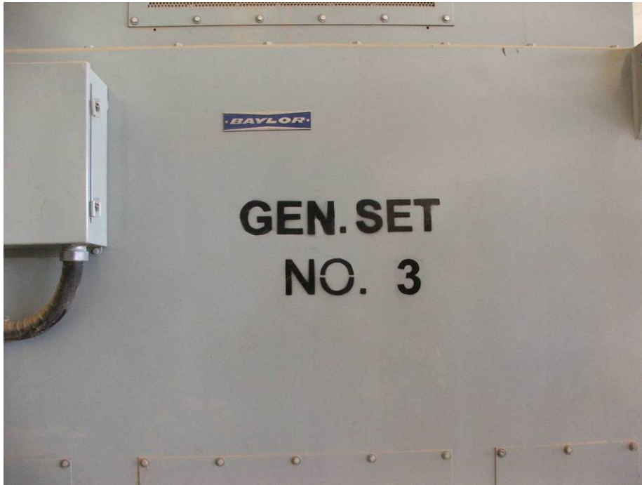
Site Photo 16. GE generator set 3
