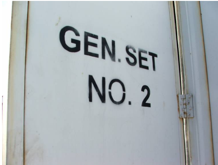
Site Photo 36. Caterpillar generator set 2
