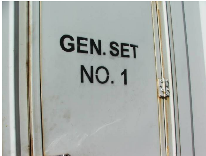
Site Photo 34. Caterpillar generator set 1
