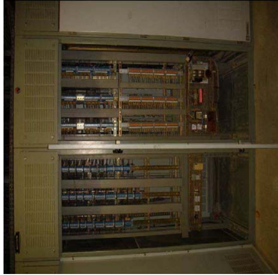
Site Photo 9. Programmable Logic Controller system (Photo provided by USAID)
