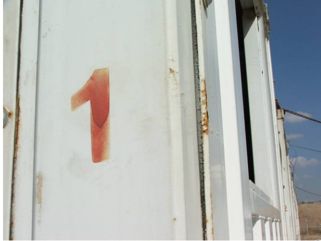
Site Photo 18. Cummins generator set 1
