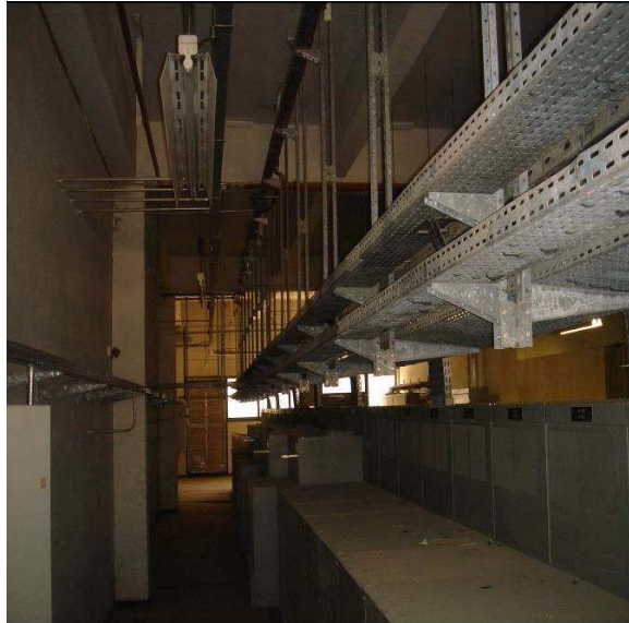
Site Photo 7. 11 kilovolt system (Photo provided by USAID)
