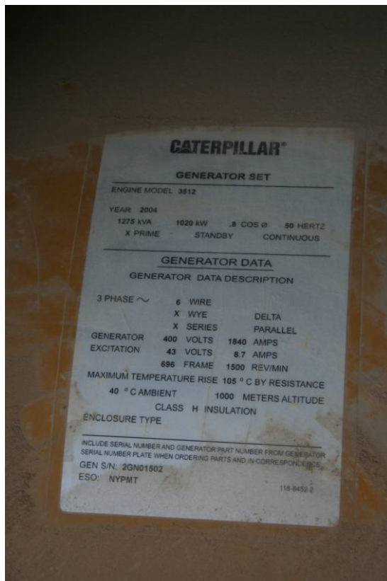
Site Photo 47. Caterpillar generator set 7 ID plate
