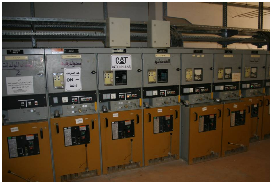
Site Photo 49. System for Caterpillar generator sets
