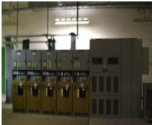
Site Photo 8. 11 kilovolt system (Photo provided by USAID)
