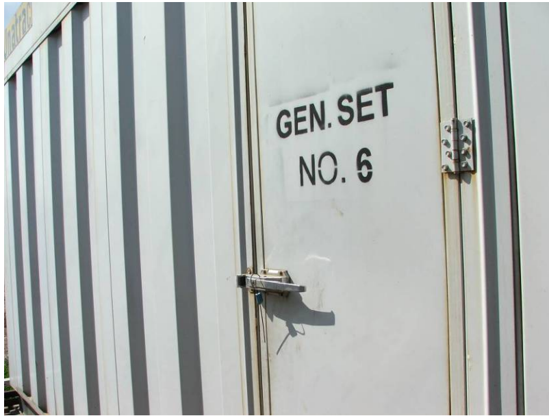
Site Photo 44. Caterpillar generator set 6
