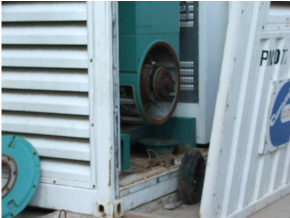
Site Photo 33. Cummins generator set 2 disassembled & unprotected from weather
