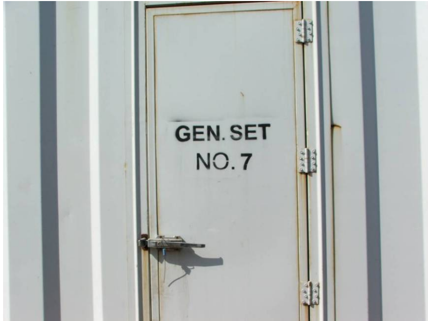
Site Photo 46. Caterpillar generator set 7
