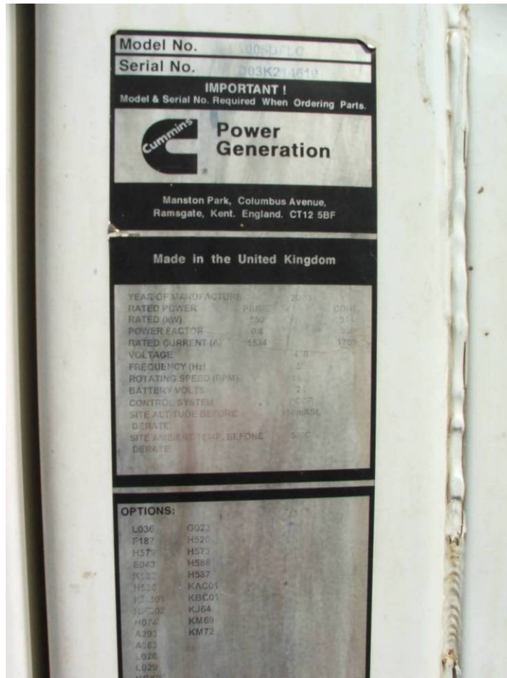
Site Photo 31. Cummins generator set 7 ID plate
