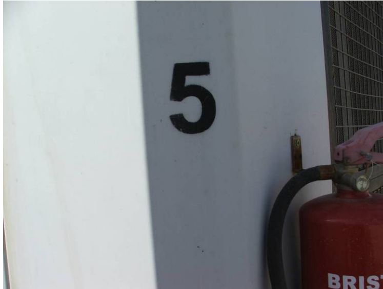
Site Photo 42. Caterpillar generator set 5
