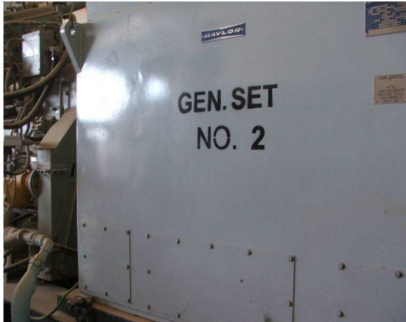
Site Photo 14. GE generator set 2
