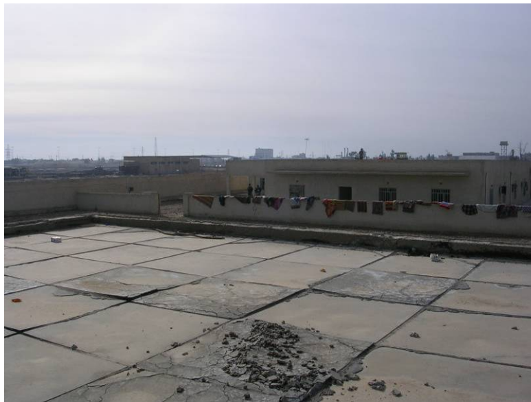
Site Photo 7. Deteriorated roof tiles on the guard house
