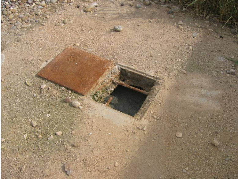
Site Photo 10. Sewage holding tank filled to capacity and draining to the adjacent lot
