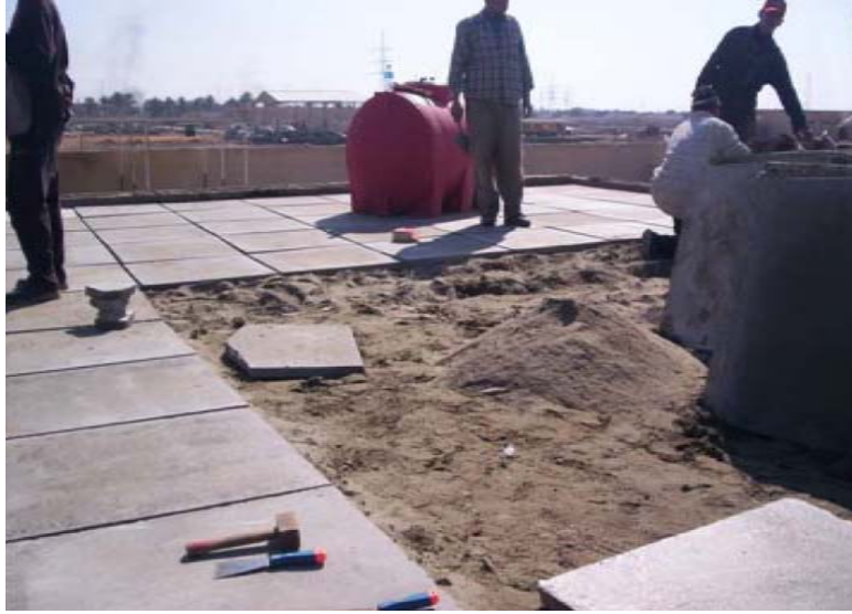
Site Photo 8. Contractor repairing the guard house roof after being notified by SIGIR (From Weston photo log)
