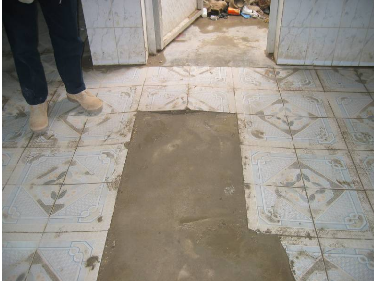
Site Photo 1. Bathroom floor tile damage caused by buckling from ground swelling
