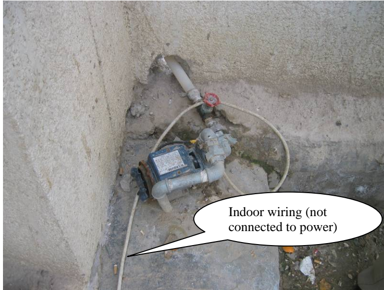
Site Photo 6. Exposed water pump connected to the main water supply line using indoor wiring. (Wiring is not connected to electrical power.)
