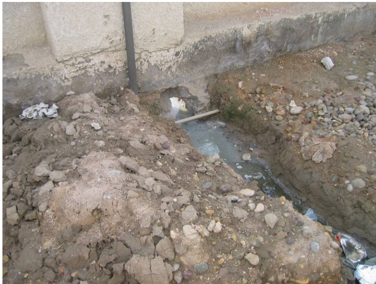
Site Photo 2. Raw sewage draining from the holding tank to the adjacent property.
