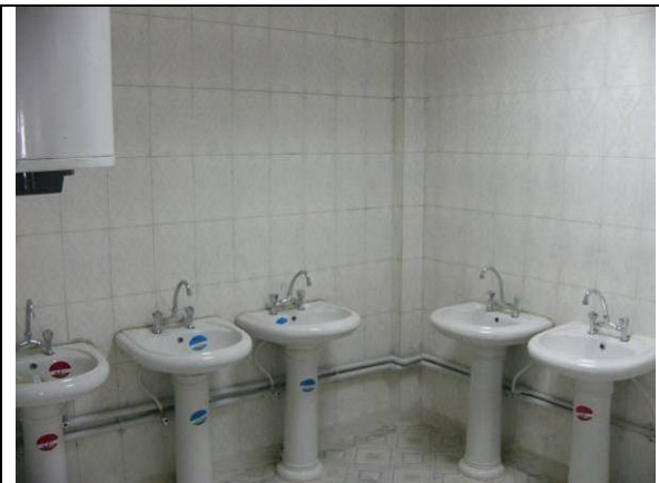
Site Photo 1. Example of bathroom sinks immediately after construction (From Weston photo log)
