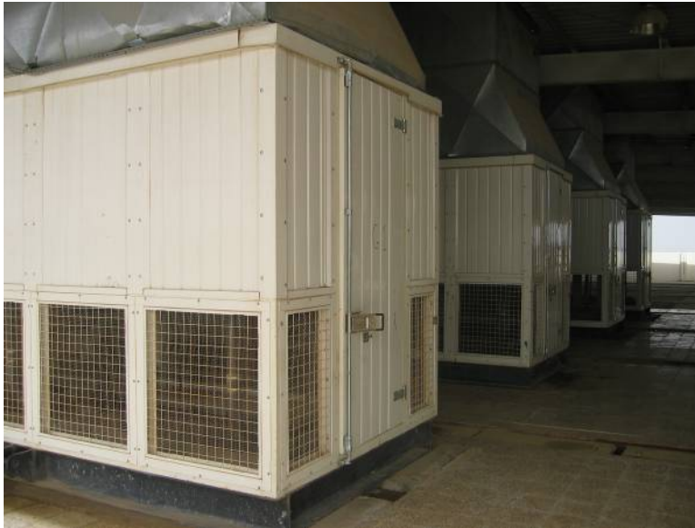
Site Photo 8. Remaining base plant generators.
