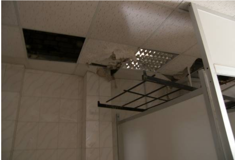
Site Photo 5. Ground floor ceiling water damage caused by leak and excess water from the bathroom above. The bed frame was apparently used to protect the person below in case the ceiling collapsed.
