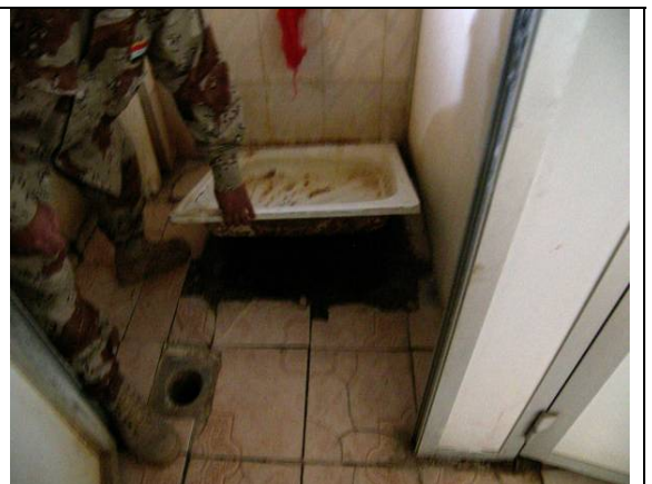
Site Photo 4. Dislodged shower floor pan at inspection
