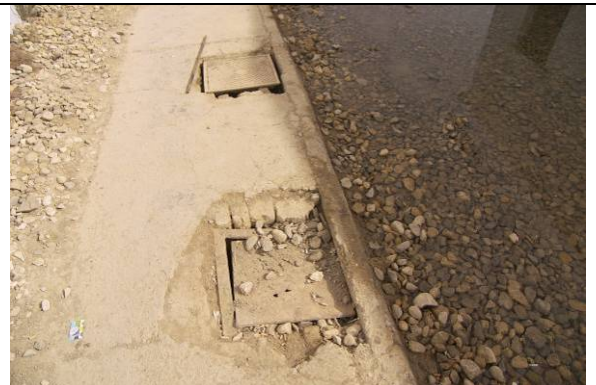
Site Photo 10. Drainage cleanout holes and standing water that should drain into the system
