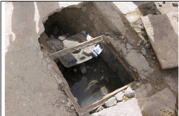
Site Photo 9. Broken drain cleanout hole
