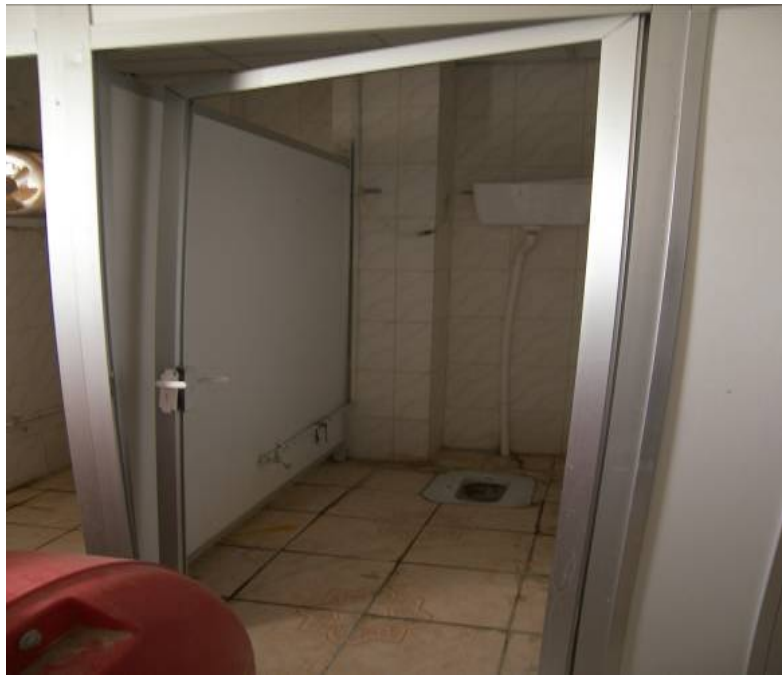
Site Photo 6. Closed toilet door frame with missing center panel
