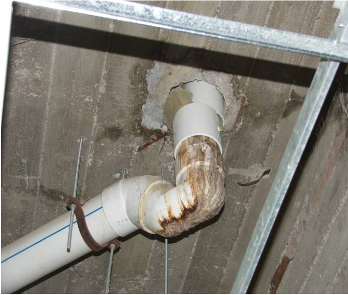
Site Photo 12. View of wastewater leaking from pipe
