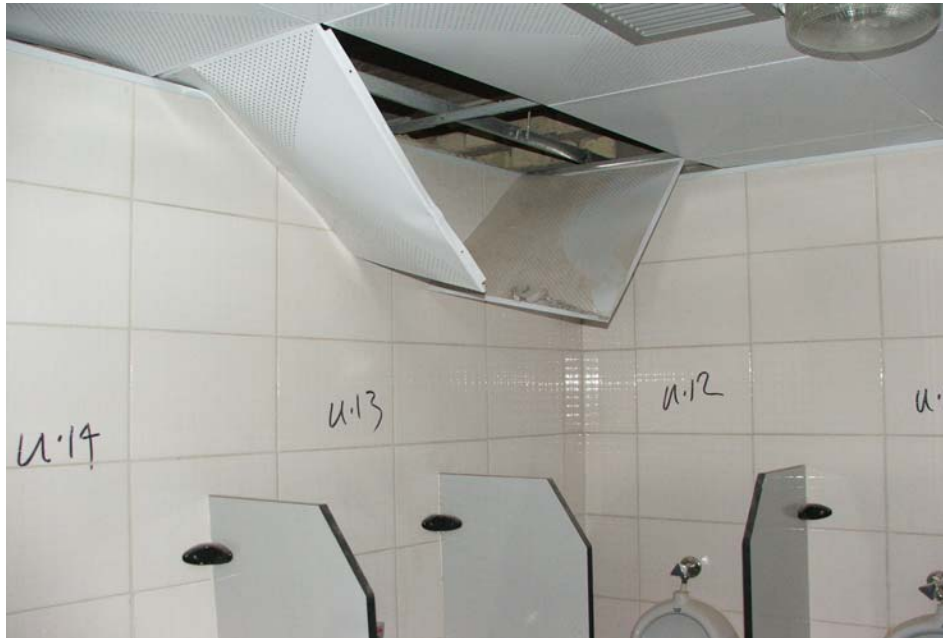
Site Photo 6. Water damage to second floor bathroom ceiling
