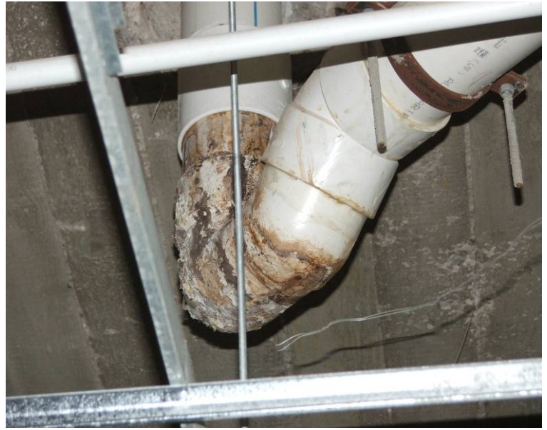
Site Photo 13. View of another pipe leaking wastewater
