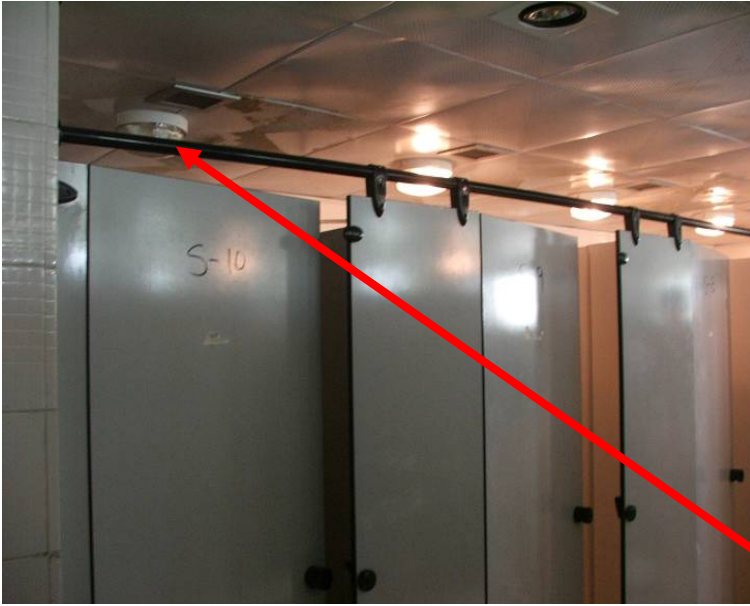
Site Photo 16. Bathroom lights on second floor
