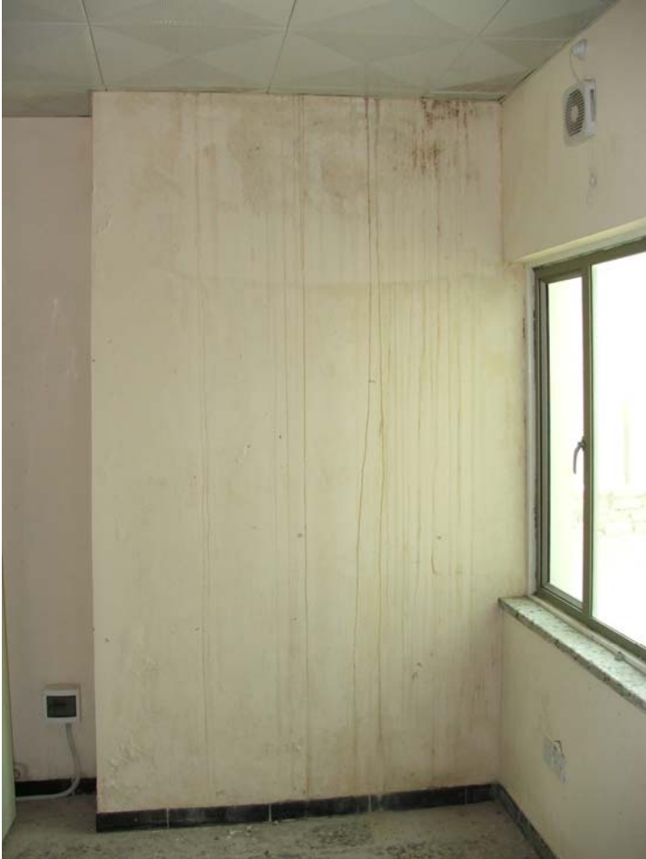
Site Photo 4. Water damage to wall
