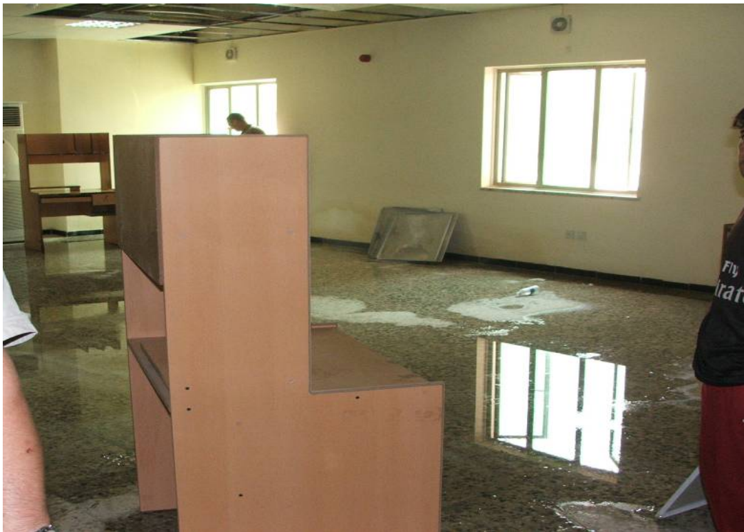
Site Photo 10. Water damage from leaking ceiling
