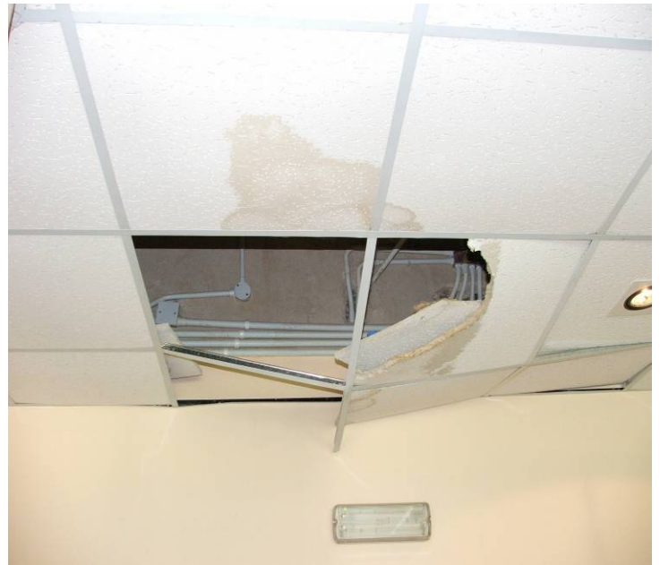
Site Photo 5. Water damage to ceiling
