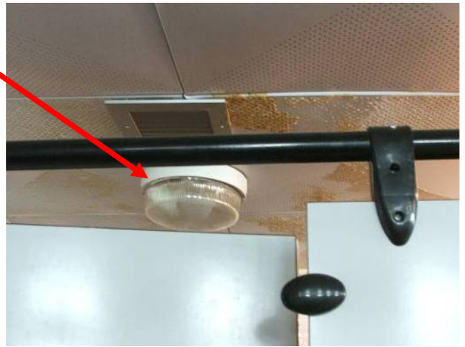
Site Photo 17. Close-up view of far left bathroom light not operating because it is full of diluted urine and fecal matter
