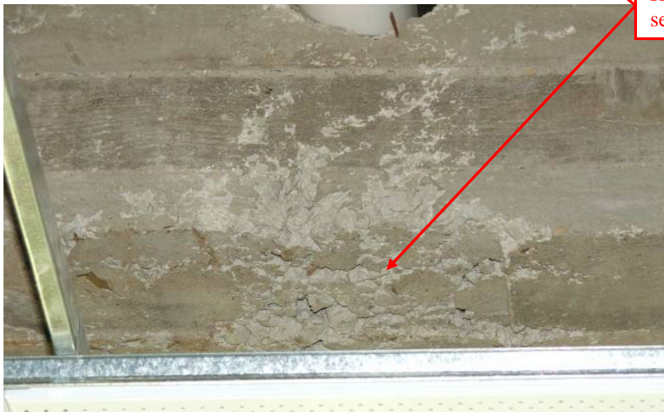
Site Photo 7. Concrete segregation and honeycombing
