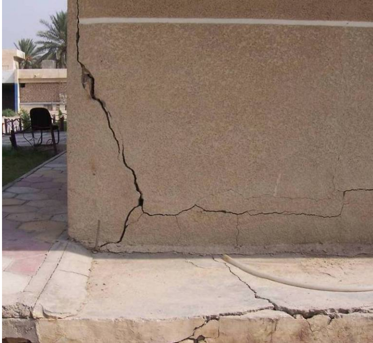
Site Photo 89. Substantial cracks in the exterior of the building and side walk
