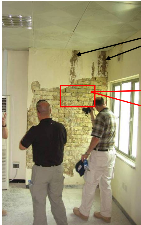
Site Photo 109. Water damage to cadet barracks ground floor common area
