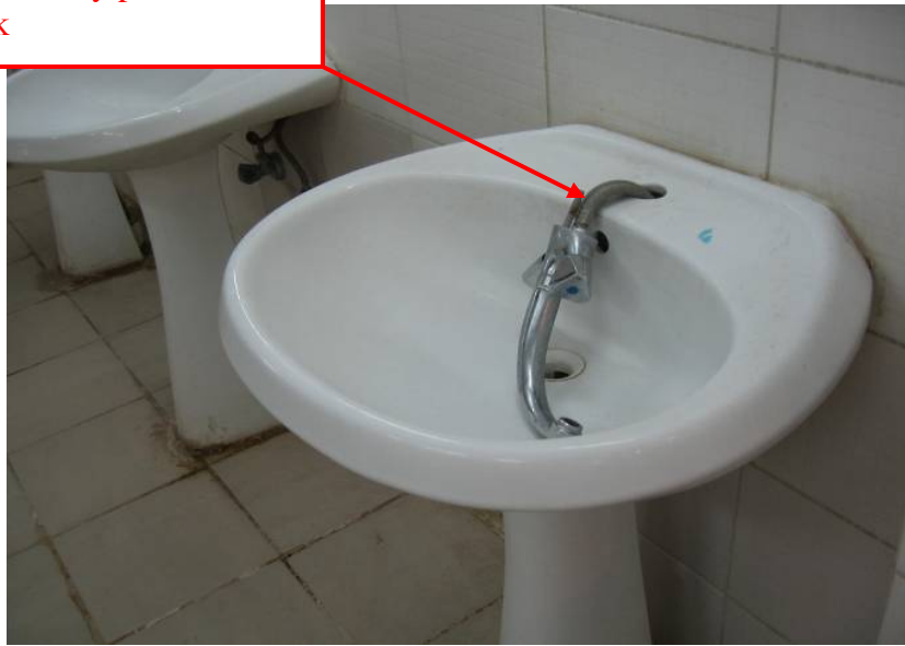
Site Photo 33. Bathroom sink in cadet barracks
