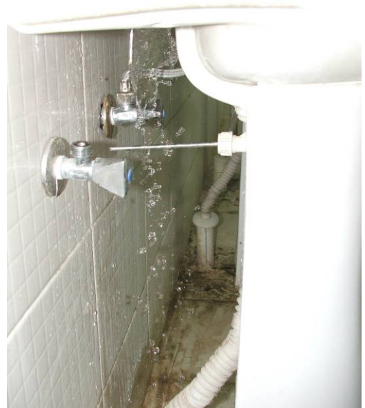
Site Photo 118. Leaking water
