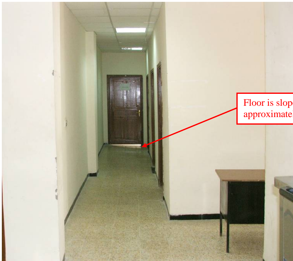
Site Photo 143. Poor construction of the first floor in Classroom E
