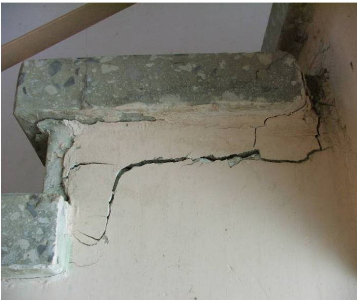
Site Photo 120. De-lamination of staircase step
