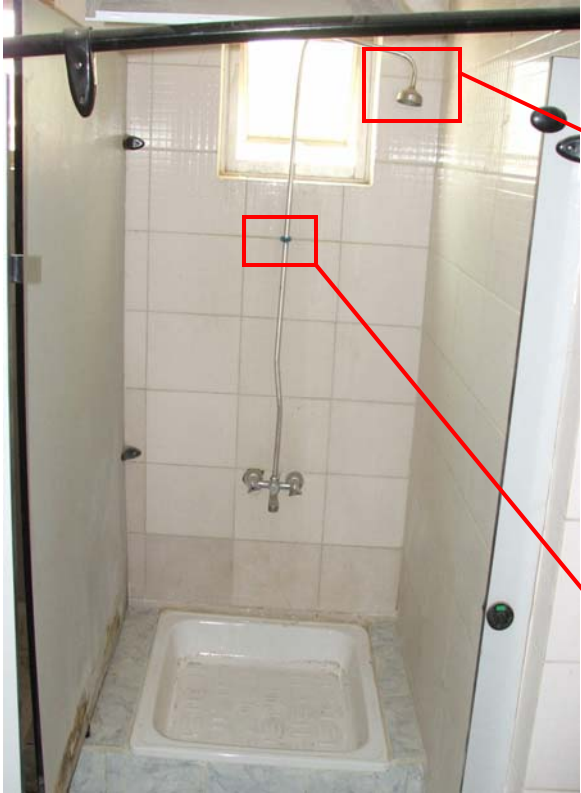
Site Photo 30. Shower fixture in cadet barracks
