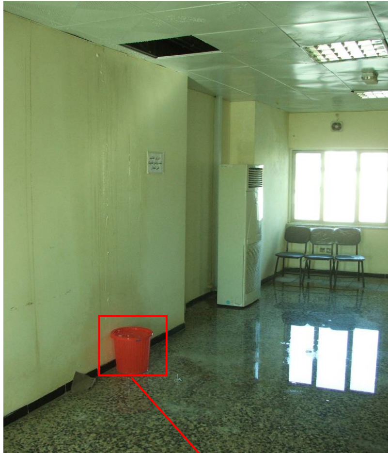
Site Photo 210. Total accumulation of leaking water in cadet barracks
