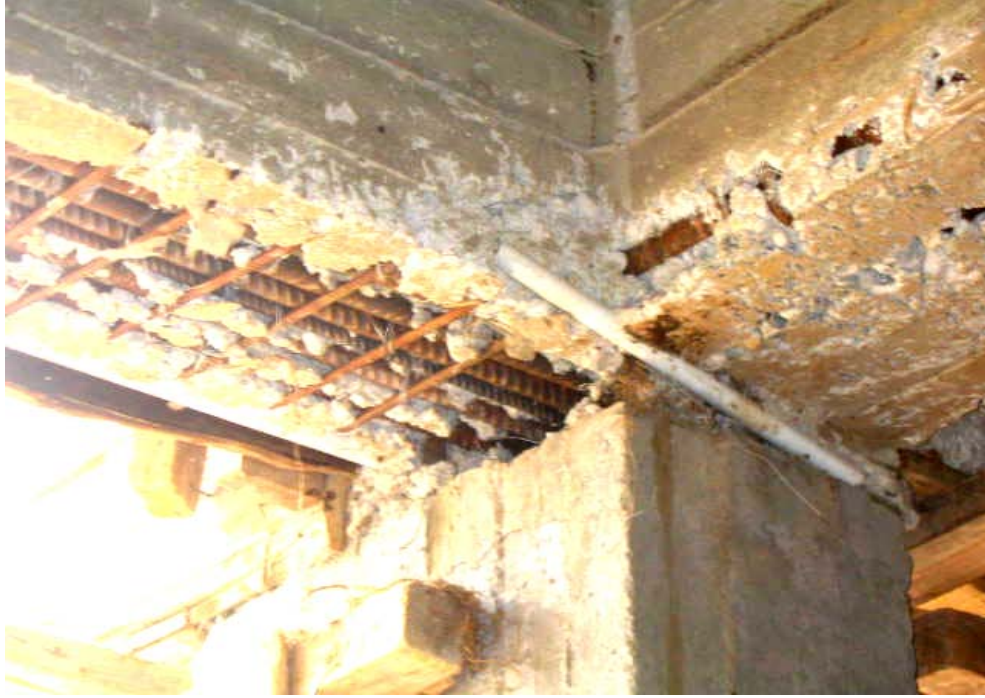
Site Photo 50. Concrete segregation, reinforcement bar and electrical conduit exposure (Photo courtesy of the USACE)
