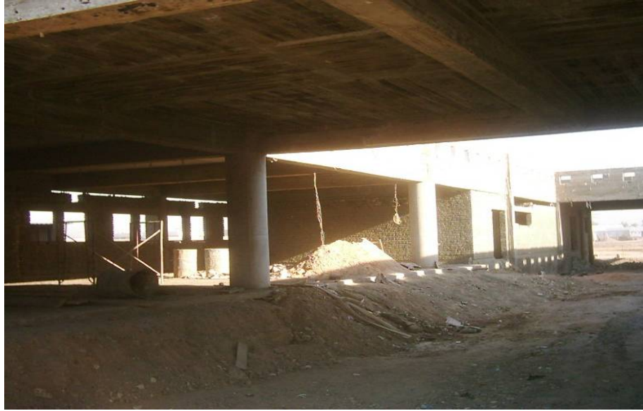
Site Photo 52. QAR daily report photo of interior of central laundry facility (Photo courtesy of the USACE)
