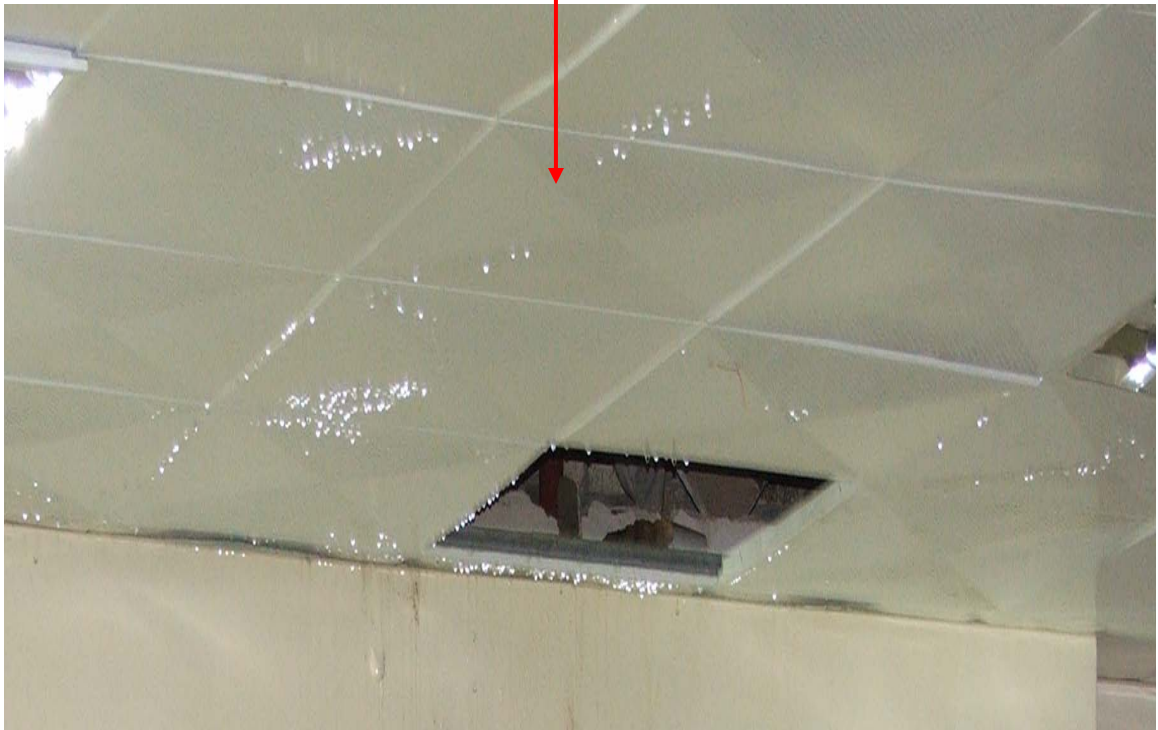
Site Photo 207. Close-up view of the water leaking from the ceiling of Site Photo 206
