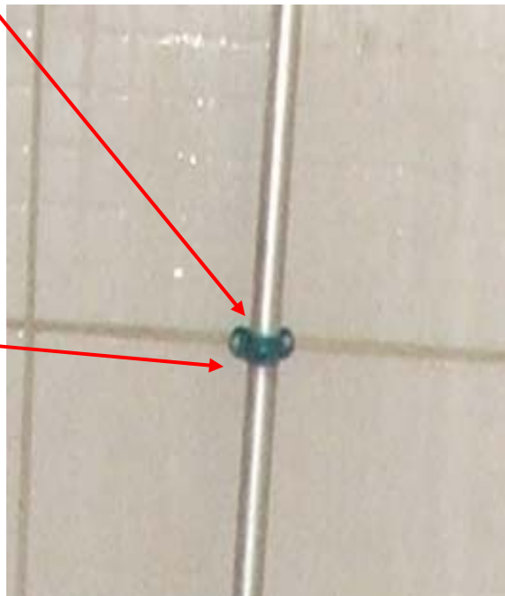
Site Photo 32. Close-up view of clamp
