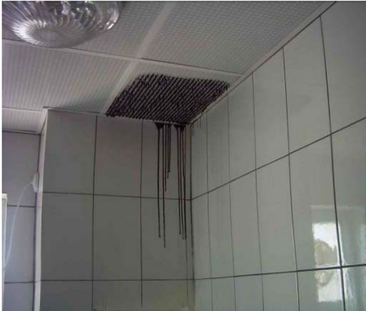
Site Photo 203. Interior damage caused by leaking tar
