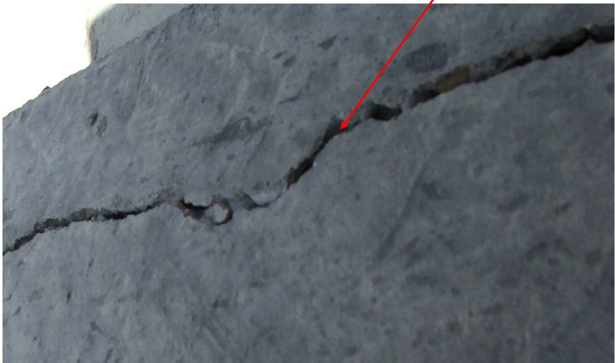
Site Photo 135. Enlarged view of expansion crack from Site Photo 103
