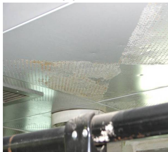
Site Photo 215. Crystallized urine stains on ceiling panels
