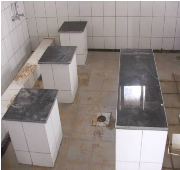
Site Photo 147. Interior of ablution unit
