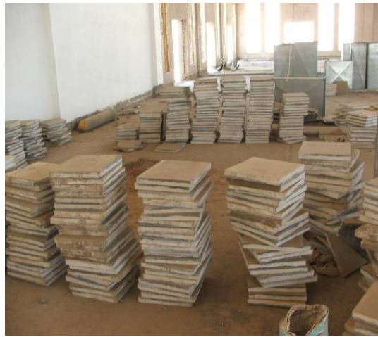
Site Photo 192. Materials left by Parsons
