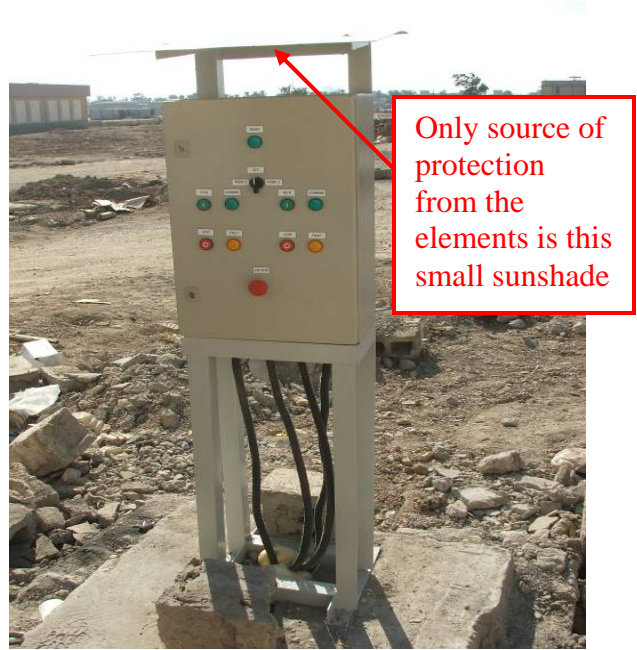
Site Photo 162. Dual pump station control panel
