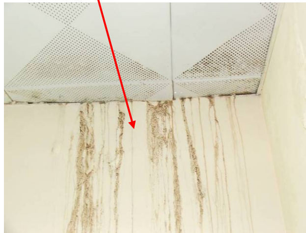
Site Photo 12. Water damage on ground floor from leak on 2 nd floor
