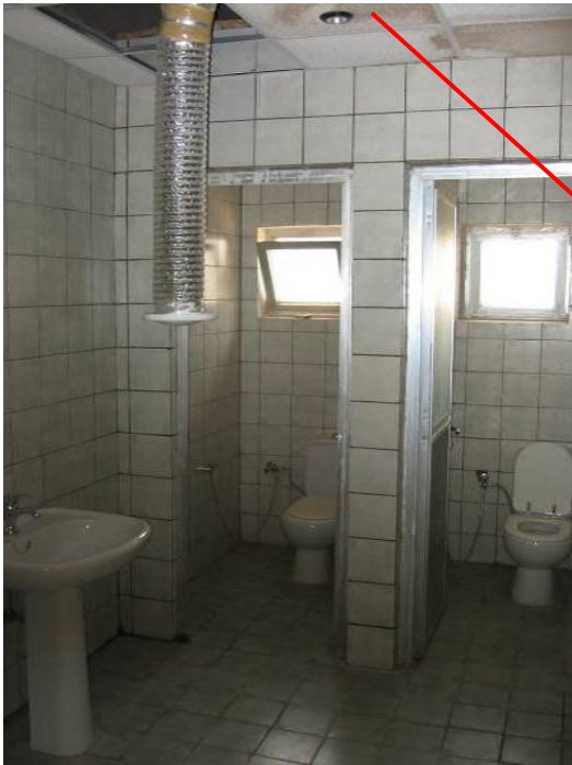
Site Photo 150. Water damage on ceiling panel
