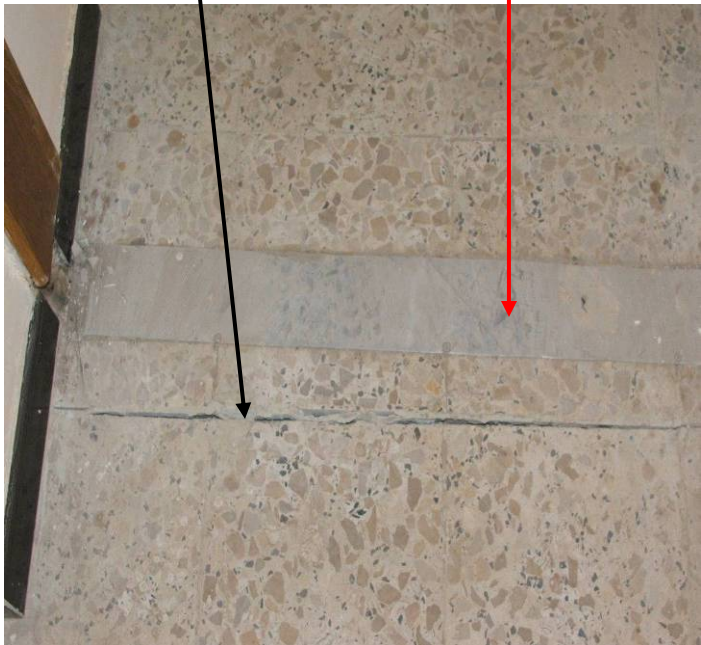
Site Photo 132. Interior expansion crack
