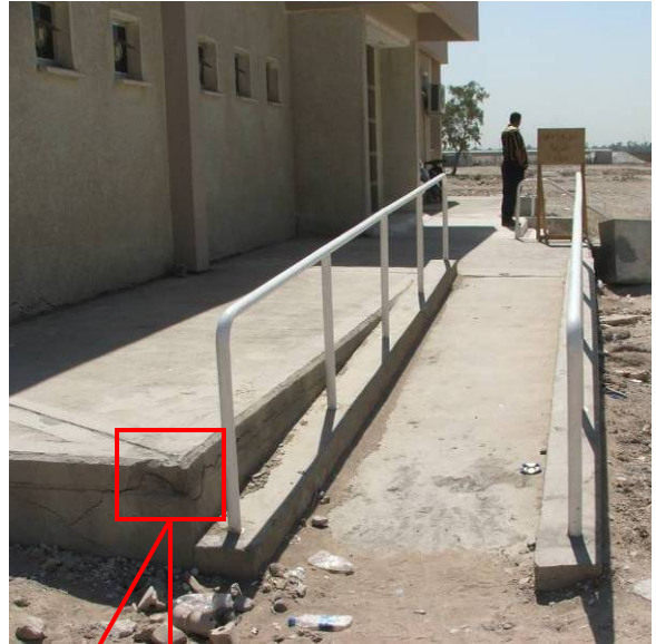
Site Photo 153. Defective concrete work
