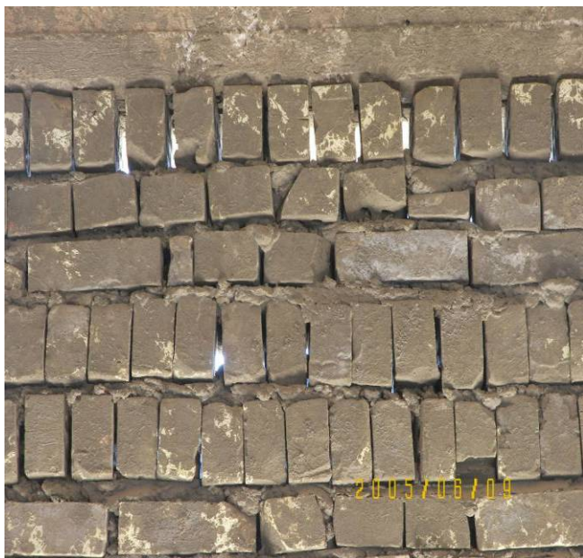
Site Photo 186. Example of poor brick workmanship
