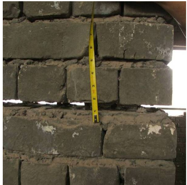
Site Photo 185. One inch gap between bricks
