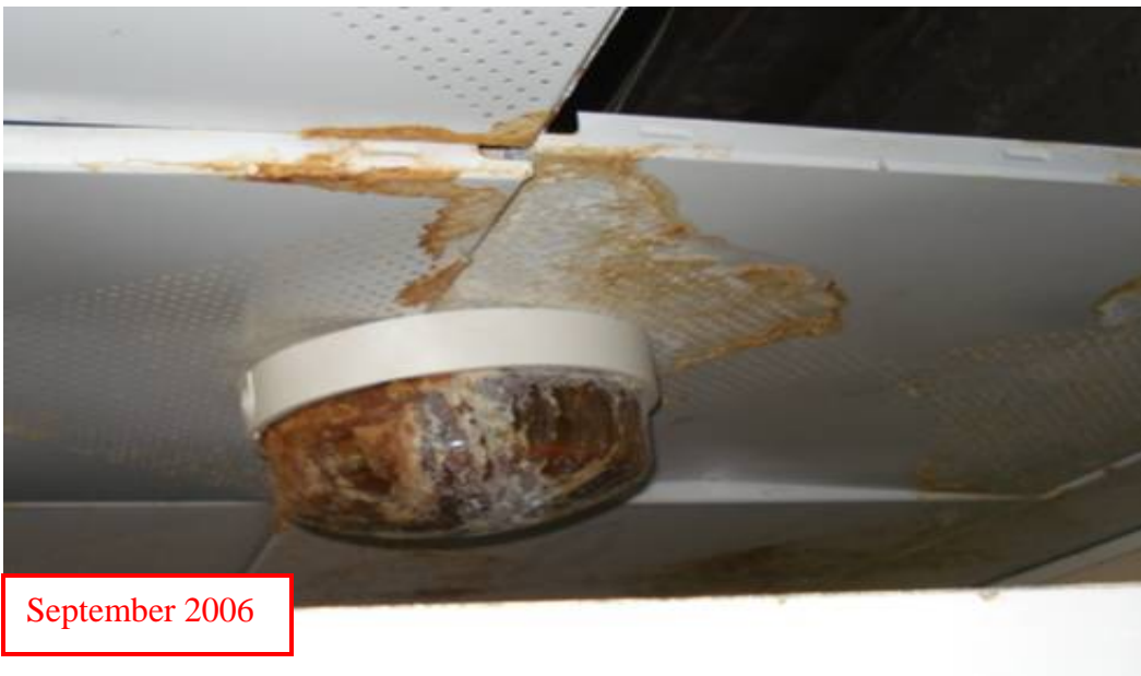
Site Photo 98. Urine-filled light fixture in cadet barracks bathroom from original construction
