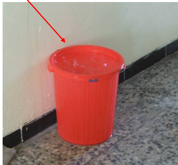
Site Photo 211. Close-up of bucket full of leaking water
