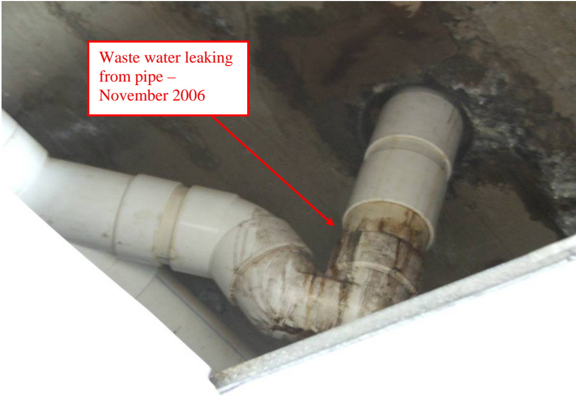
Site Photo 208. Effect of leaking waste water on plumbing pipes
