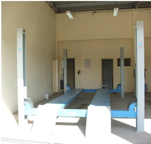
Site Photo 168. Car lift within the motor pool
