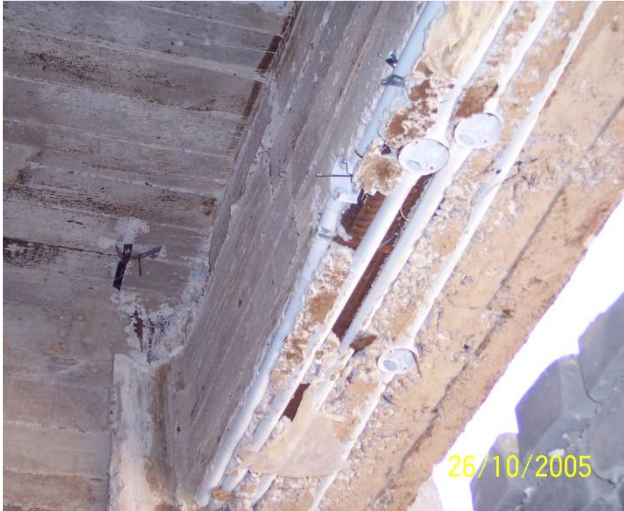
Site Photo 48. Electrical conduit exposure and reinforcement bar rust (Photo courtesy of the USACE)
