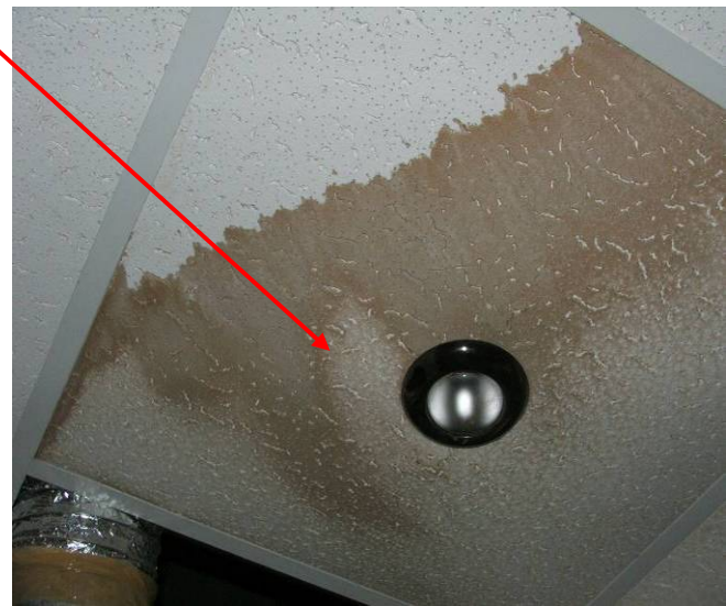
Site Photo 151. Close-up view of water damage
