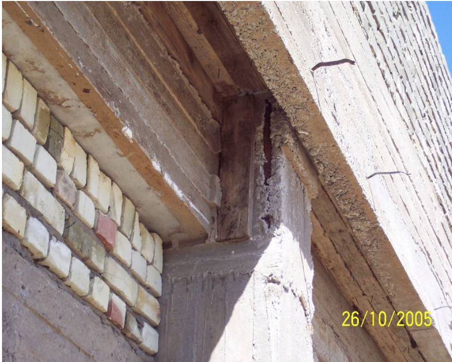
Site Photo 46. Concrete segregation and exposed reinforcement bar (Photo courtesy of the USACE)
