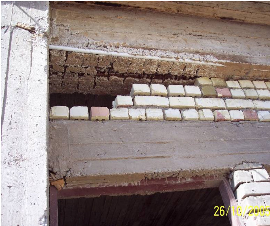
Site Photo 49. Concrete segregation and electrical conduit exposure (Photo courtesy of the USACE)
