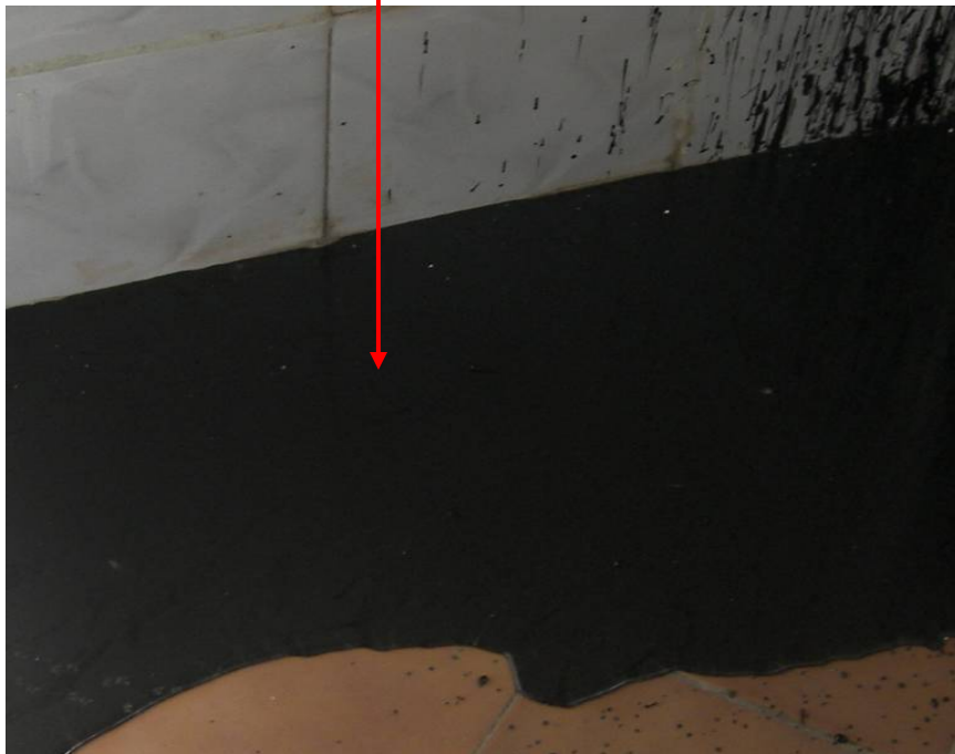
Site Photo 128. Close-up view of tar damage from Site Photo 127
