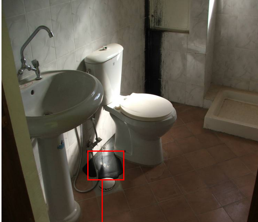
Site Photo 127. Tar damage on wall and floor of an instructors' barracks bathroom
