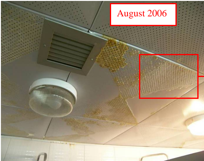
Site Photo 100. Urine stain on second floor ceiling
