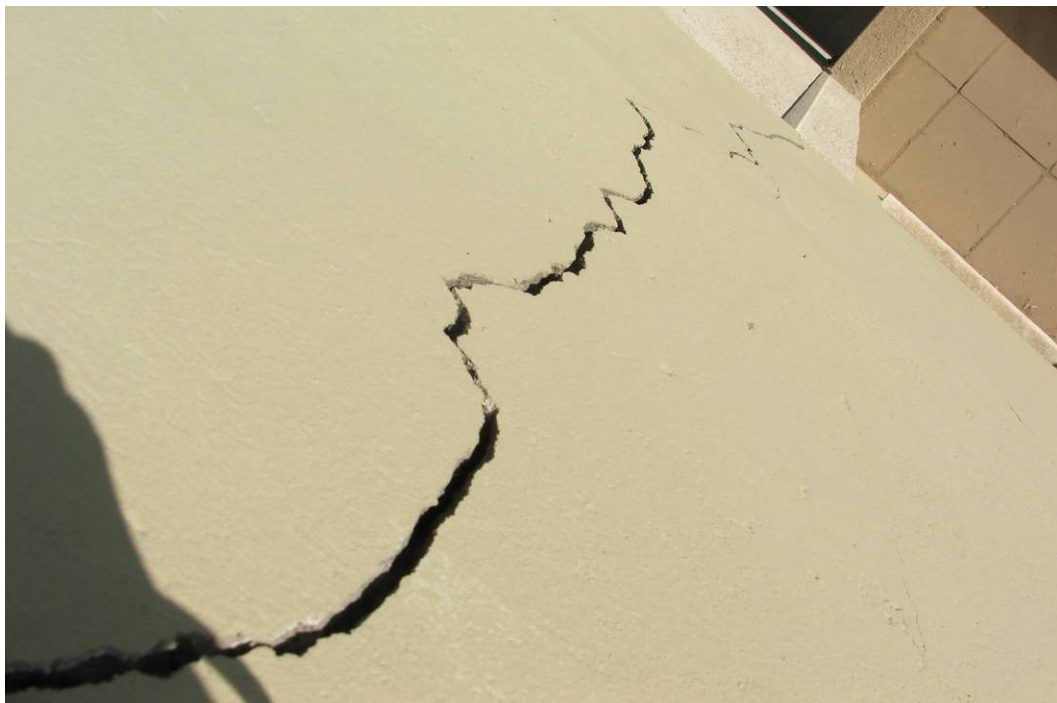
Site Photo 83. Substantial exterior expansion crack
