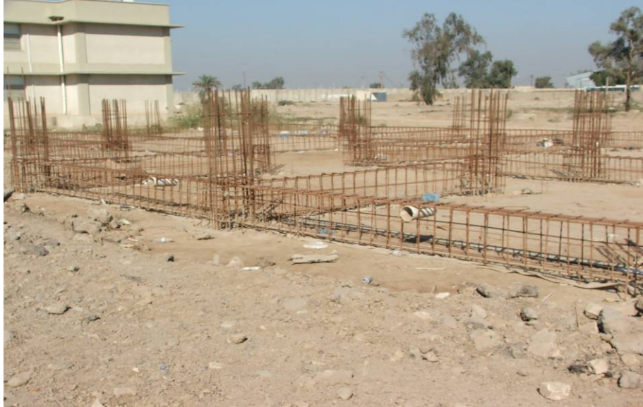
Site Photo 199. Partially completed weight training room, with reinforcement bar exposure
