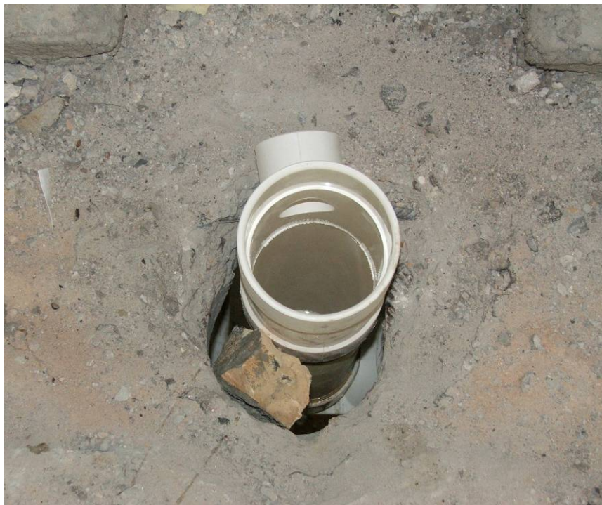
Site Photo 79. Example of poor sealing technique used by the contractor during rework construction
