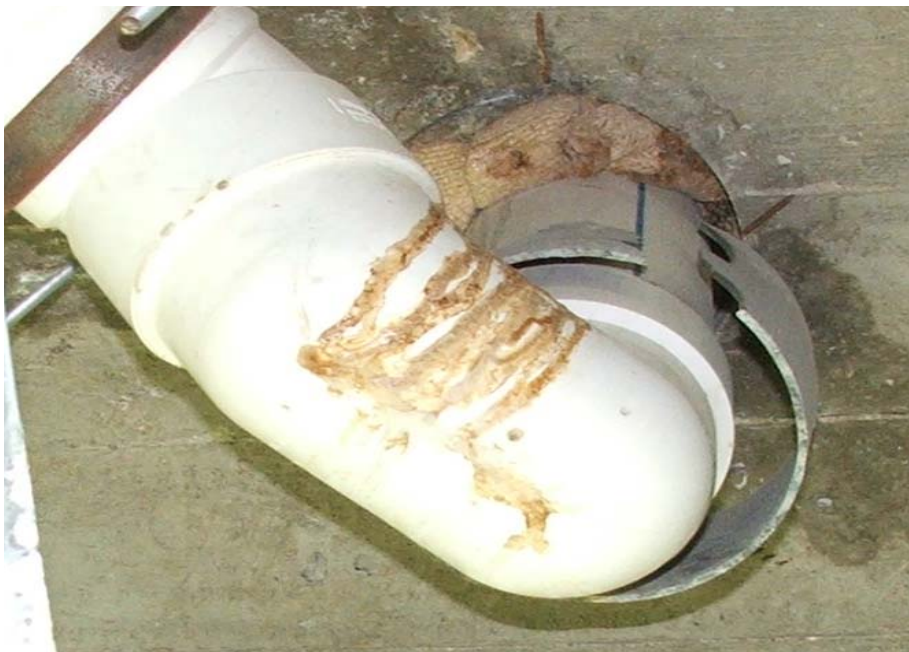
Site Photo 63. Example of poor sealing technique used by the contractor
