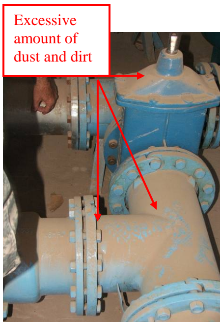
Site Photo 175. Dirt within the pump room
