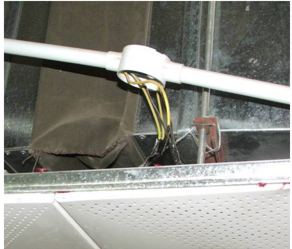
Site Photo 217. Wires taped together
