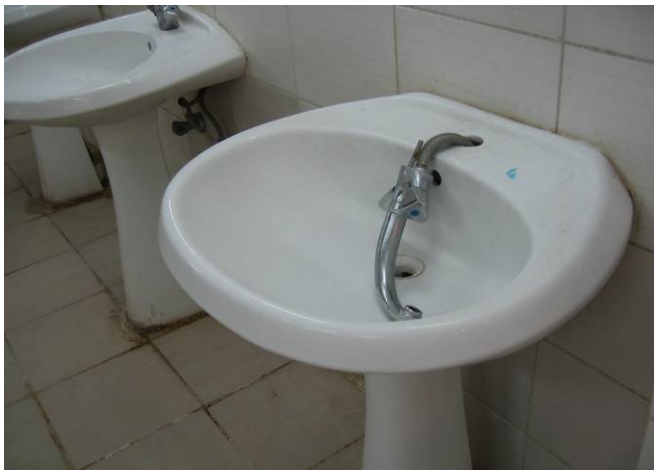
Site Photo 117. Broken sink fixture
