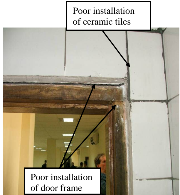
Site Photo 142. Example of poor installation
