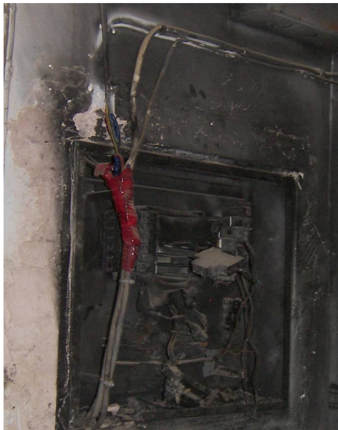
Site Photo 36. Electrical panel for the dog kennel
