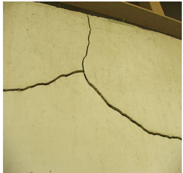
Site Photo 121. Staircase crack
