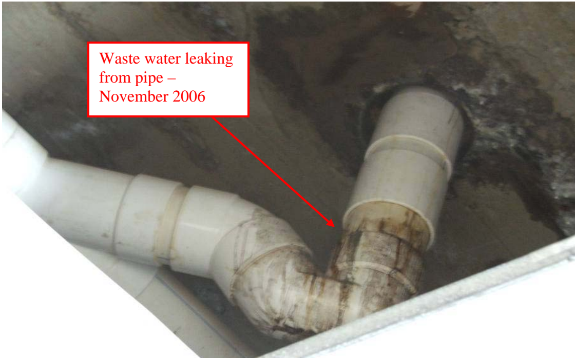
Site Photo 95. Effect of leaking waste water on plumbing pipes
