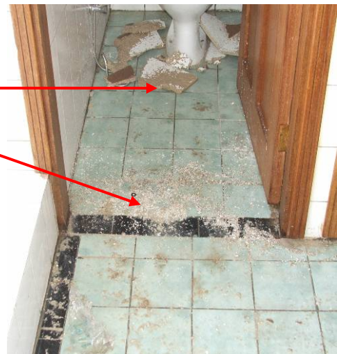
Site Photo 224. Close-up of Site Photo 223
