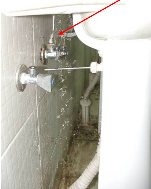
Site Photo 34. Water leak
