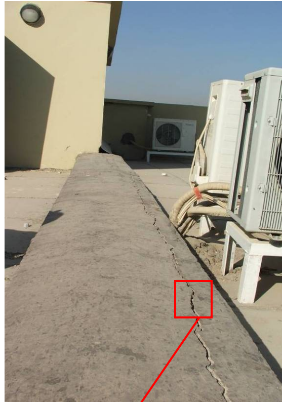
Site Photo 67. Exterior expansion crack
