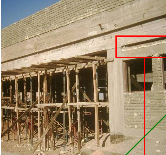
Site Photo 56. QAR provided photograph of poor construction (Photo courtesy of the USACE)
