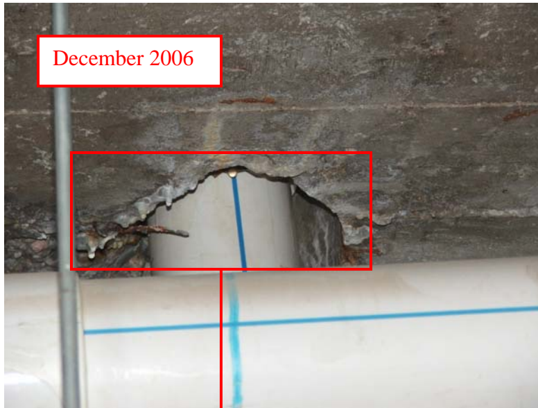
Site Photo 41. Water leaking from poorly installed drain in cadet barracks
