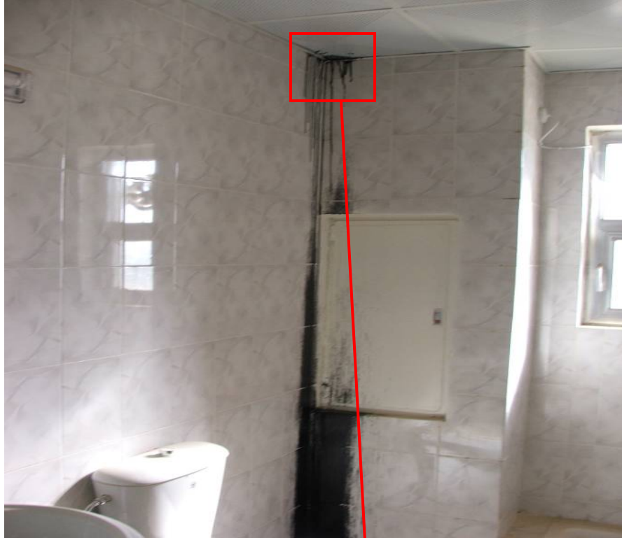
Site Photo 129. Ceiling and wall damage in bathroom
