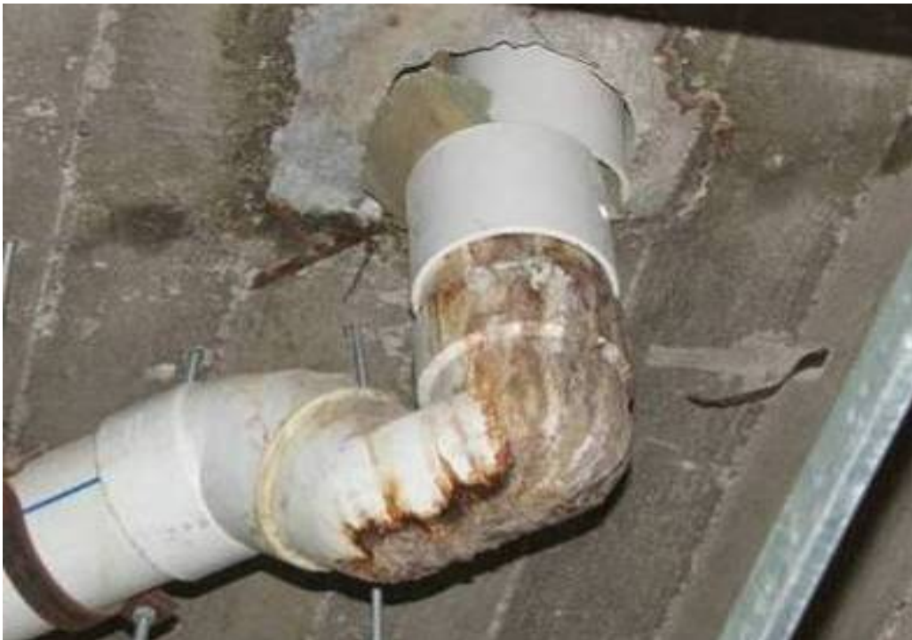
Site Photo 74. Significant plumbing leaks resulting from poorly sealed pipes
