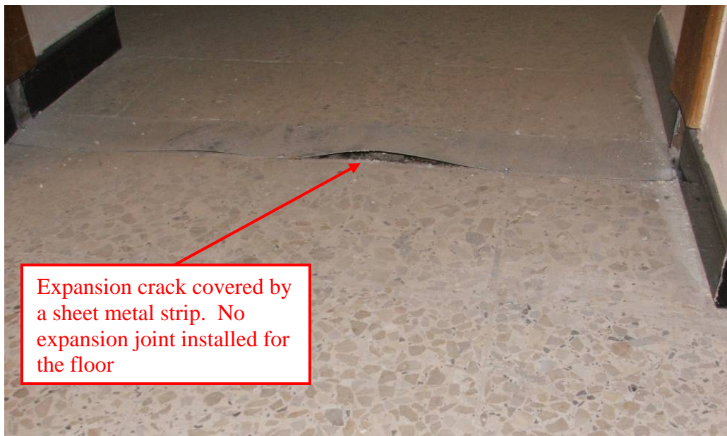
Site Photo 66. Interior expansion crack in instructors' barracks
