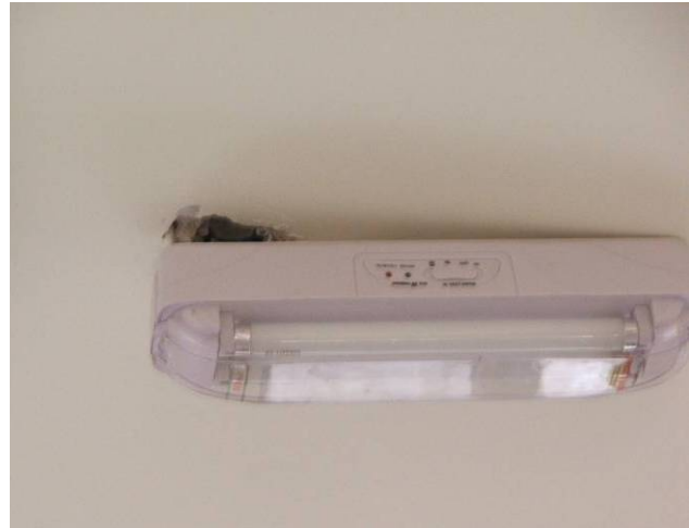
Site Photo 159. Poor installation of light fixture
