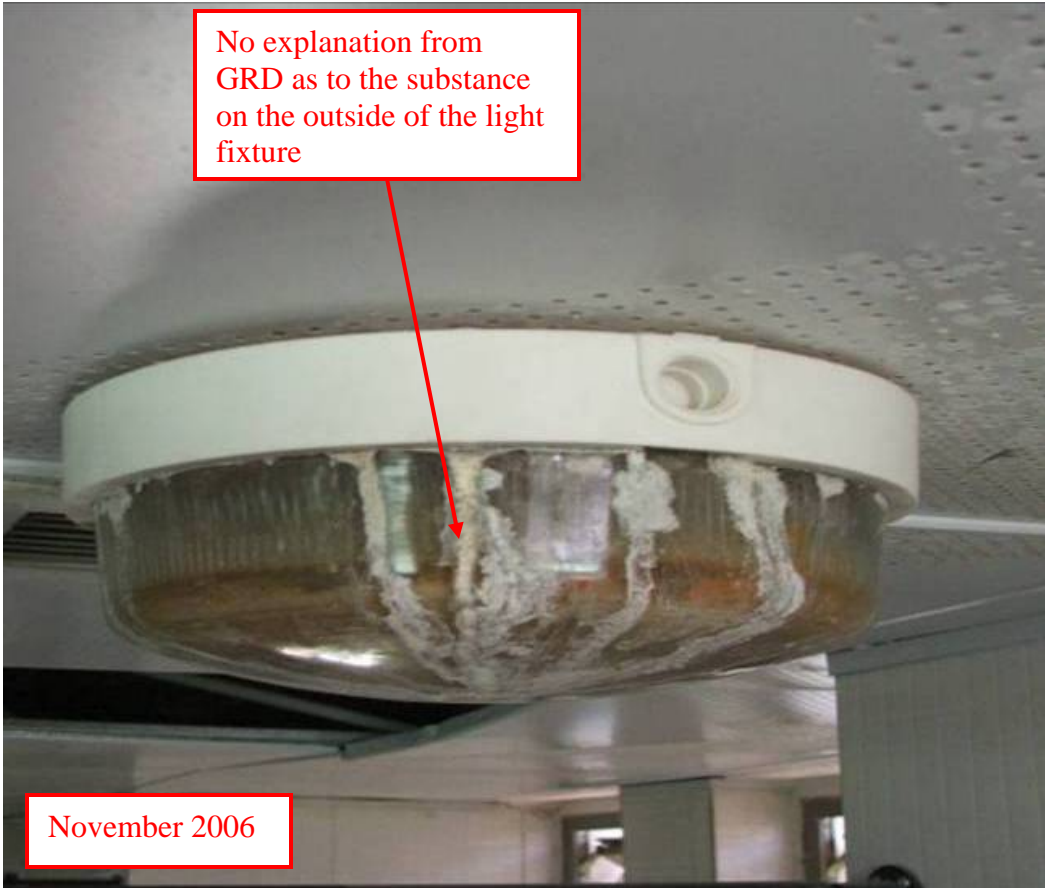
Site Photo 97. Urine-filled light fixture in cadet barracks bathroom after rework
