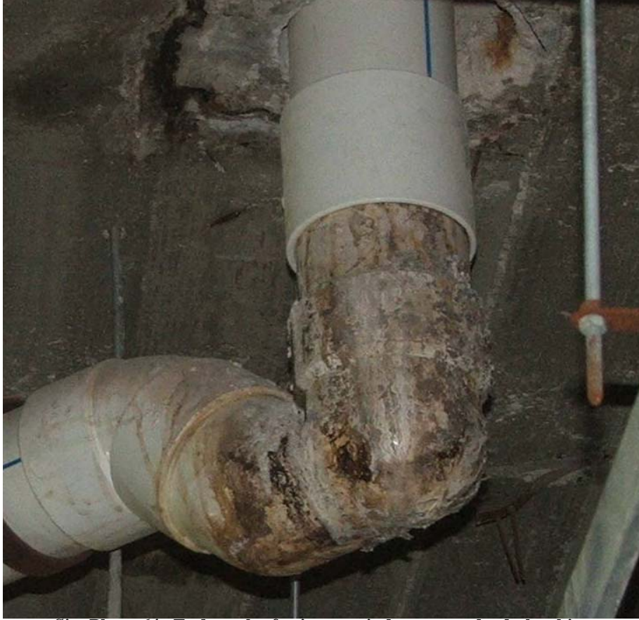
Site Photo 64. End result of using non-industry standard plumbing fixtures and not sealing pipes correctly
