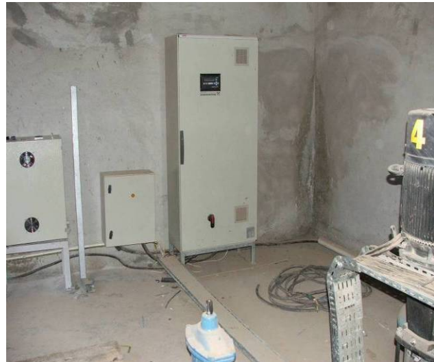
Site Photo 172. Electronic control panel in pump room
