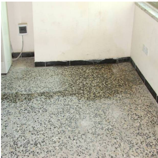
Site Photo 218. Water damage on the floor of the cadet barracks
