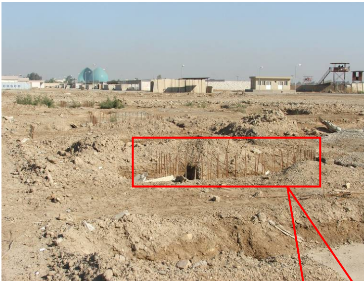
Site Photo 197. Foundation for PT field with exposed reinforcement bars extending beyond the ground
