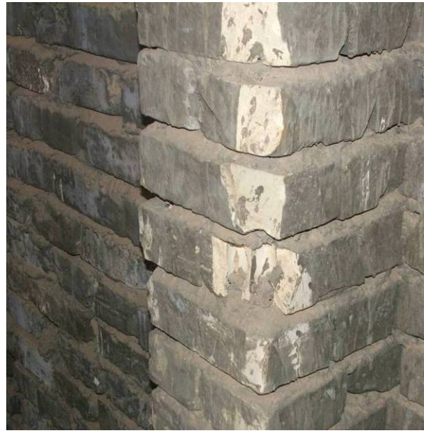
Site Photo 187. Example of poor brick workmanship
