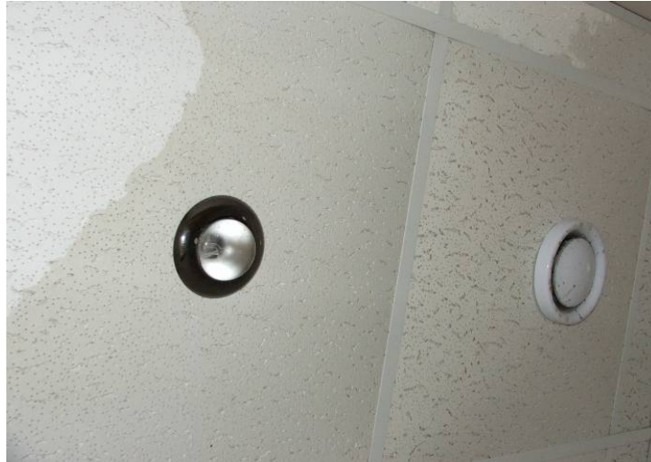
Site Photo 222. Water damage on ceiling panels
