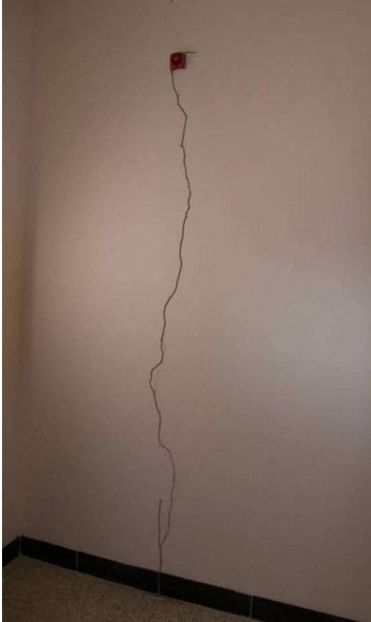
Site Photo 157. Example of termite damage to interior wall
