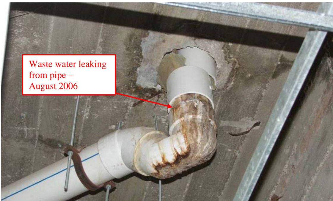
Site Photo 96. Effect of leaking waste water on plumbing pipes
