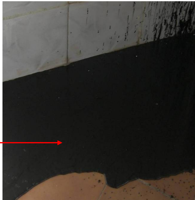
Site Photo 15. Close-up view of tar damage
