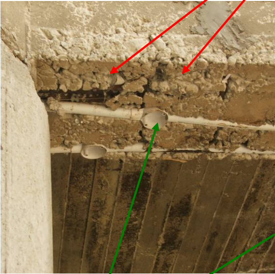
Site Photo 24. Concrete segregation and electrical conduit exposure
