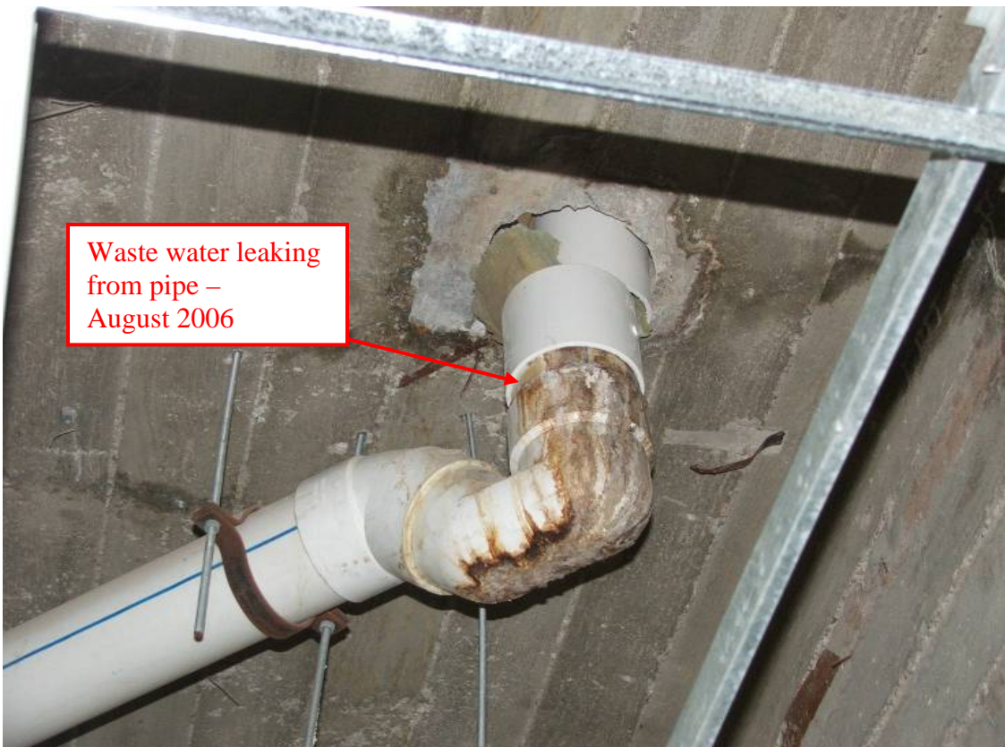
Site Photo 209. Effect of leaking waste water on plumbing pipes
