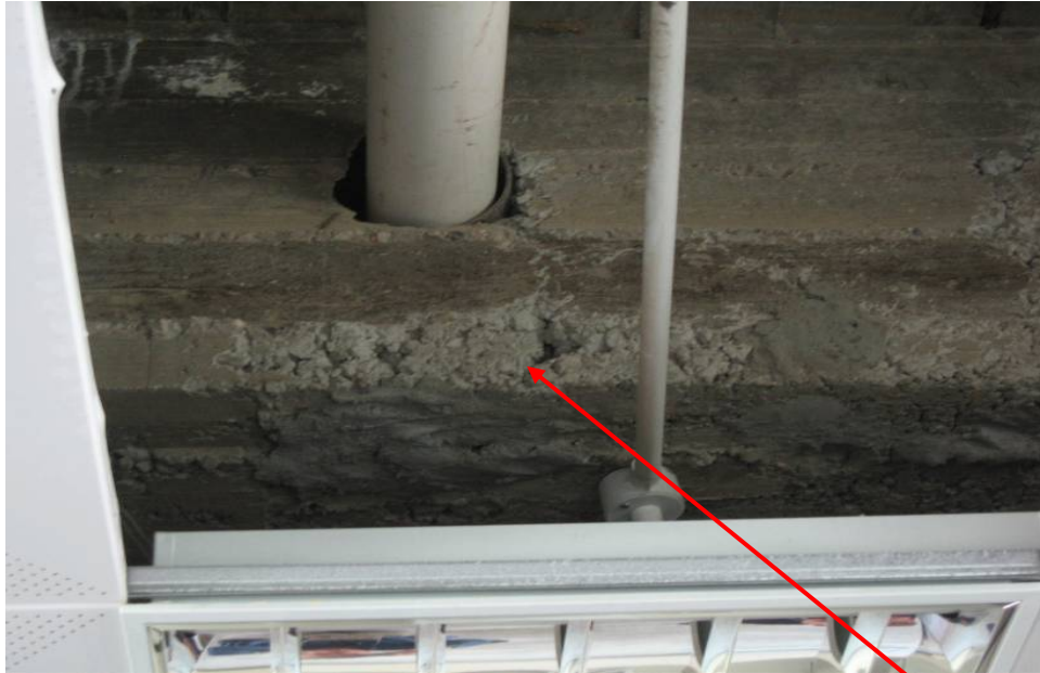
Site Photo 6. Concrete segregation and honeycombing in cadet barracks
