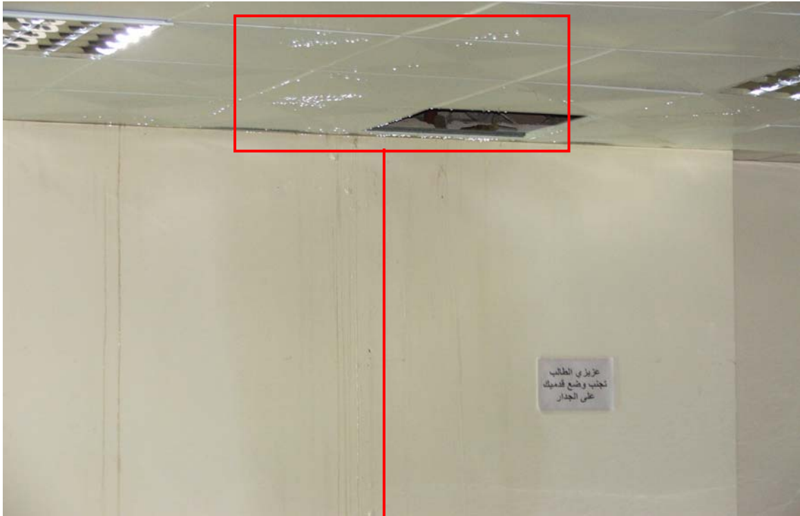
Site Photo 206. Water leaking from ceiling of cadet barracks
