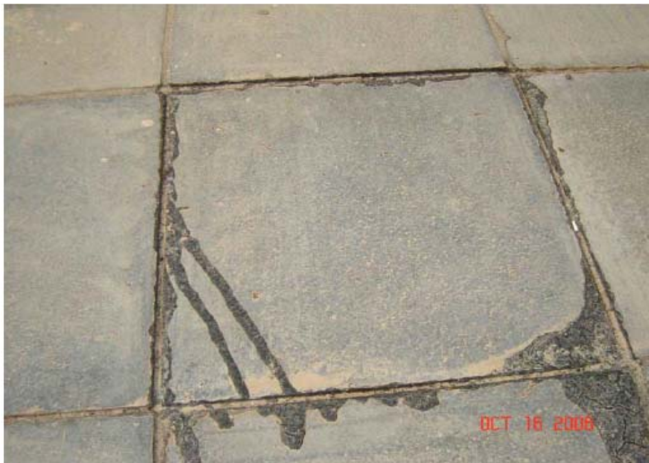
Site Photo 202. Example of poor mastic work on the roof
