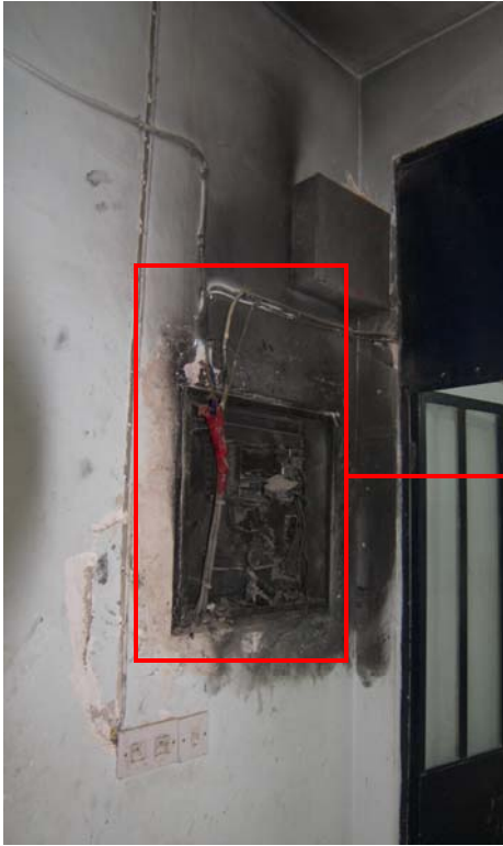
Site Photo 200. “Emergency” electrical work performed by Parsons
