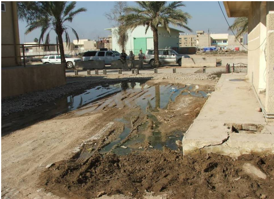
Site Photo 90. Significant standing sewer water outside the BPC security office
