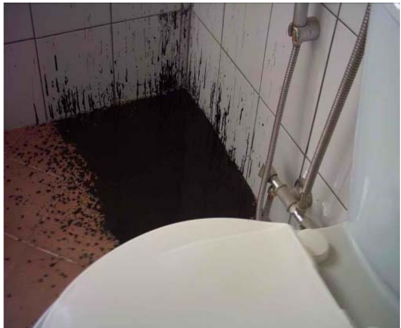
Site Photo 204. Interior damage caused by leaking tar
