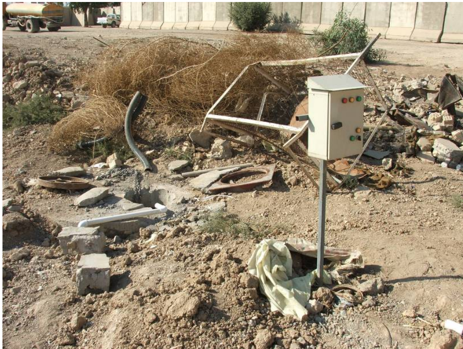
Site Photo 160. Original single pump station installed by Parsons but never connected to power
