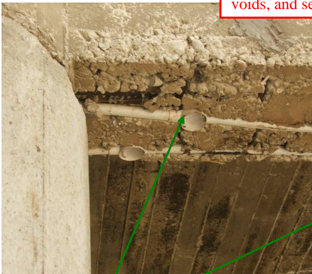
Site Photo 92. Concrete segregation and electrical conduit exposure
