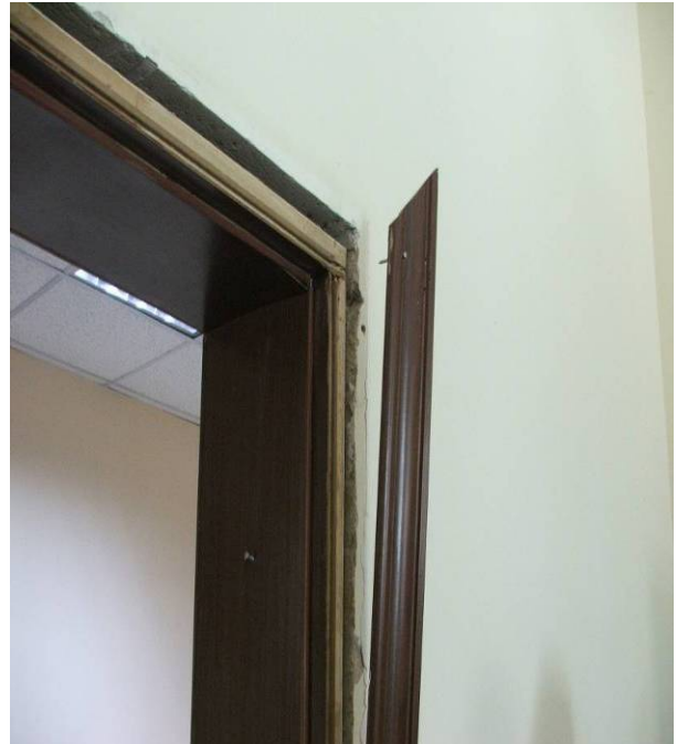
Site Photo 112. Poor door frame installation
