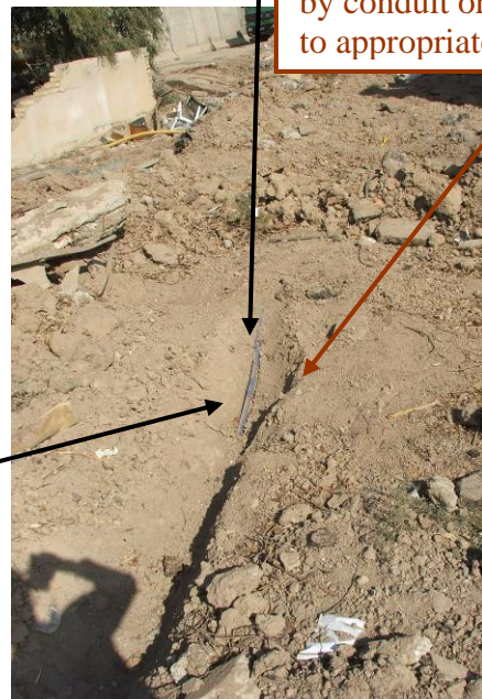
Site Photo 165. Exposed electrical power lines to pump station
