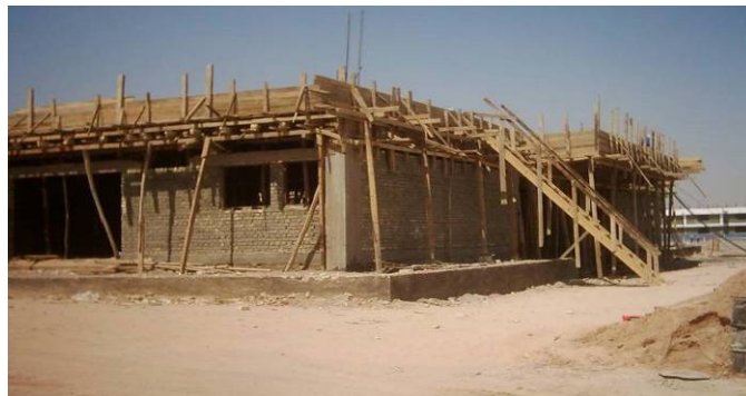
Site Photo 54. Exterior view of the central laundry facility (Photo courtesy of the USACE QAR daily report)
