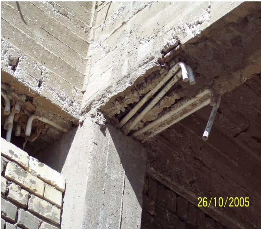
Site Photo 47. Electrical conduit exposure (Photo courtesy of the USACE)
