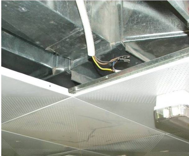
Site Photo 216. Wires taped together
