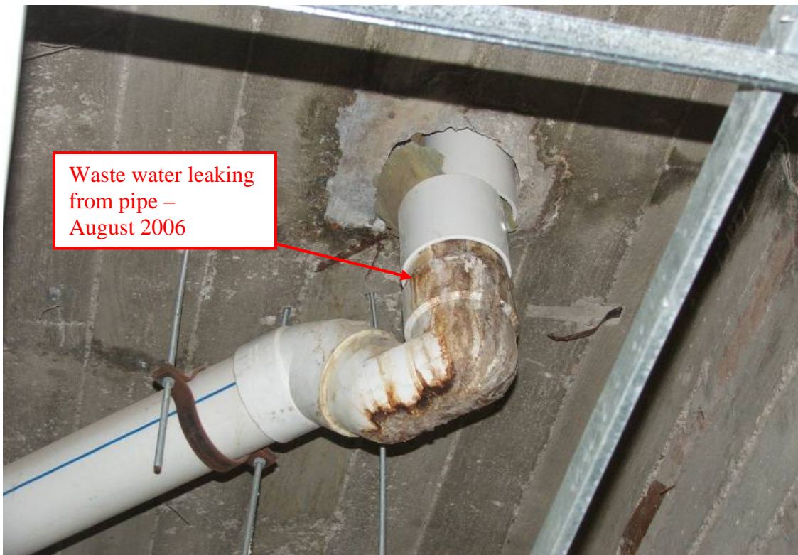
Site Photo 76. Effect of leaking waste water on plumbing pipes
