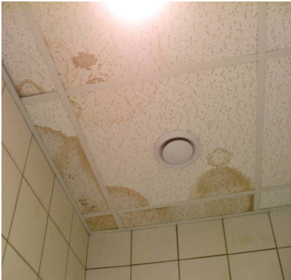
Site Photo 141. Example of water damage
