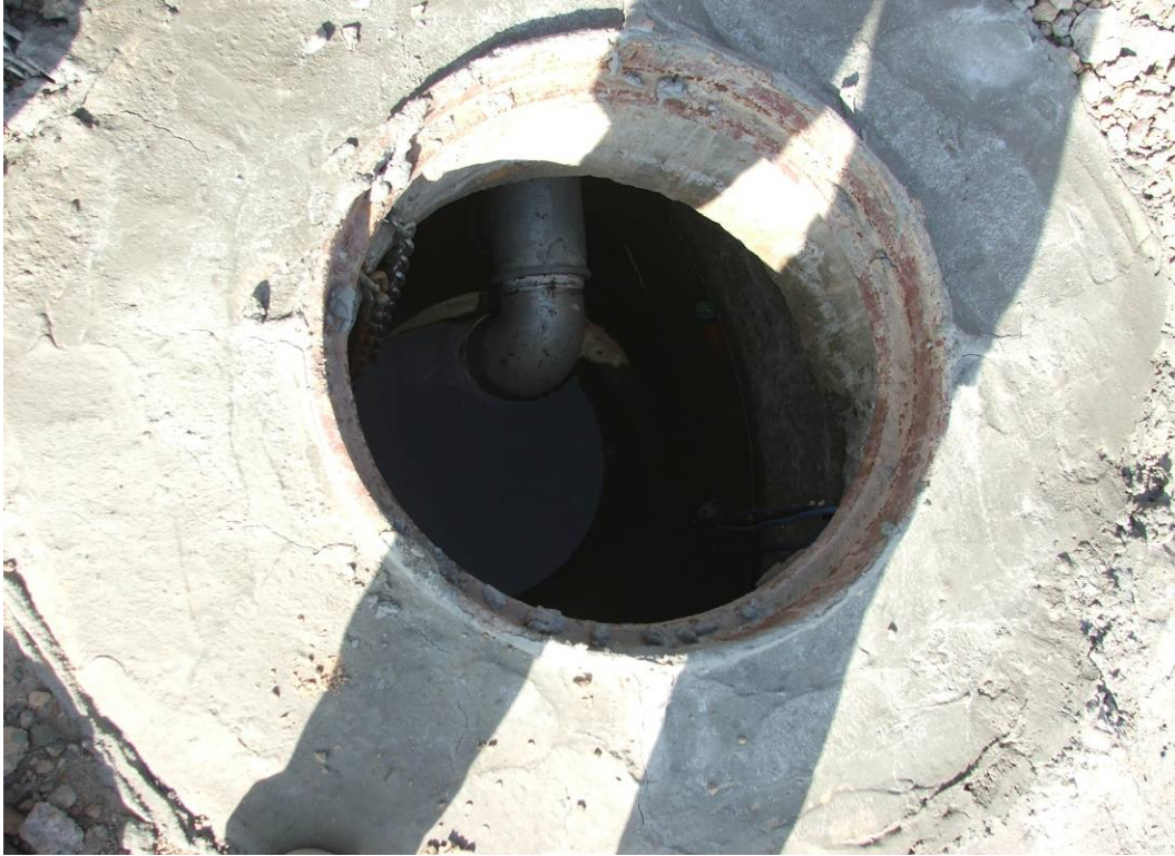
Site Photo 166. New constructed dual pump station, which is not operational due to the installation of the incorrect type of pump
