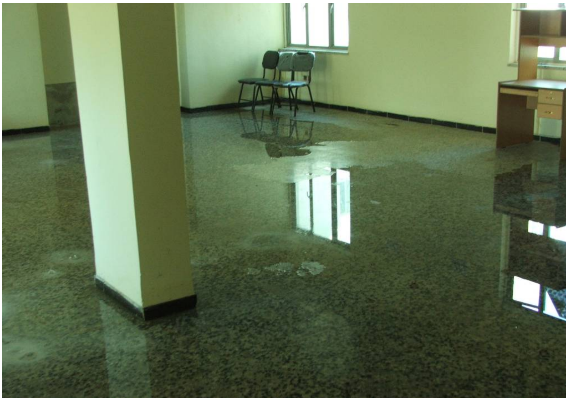
Site Photo 205. Leaking water on floor of the cadet barracks common area room
