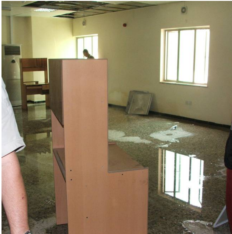
Site Photo 119. Cadet barracks common area used for storage of miscellaneous items due to continuous water leakage
