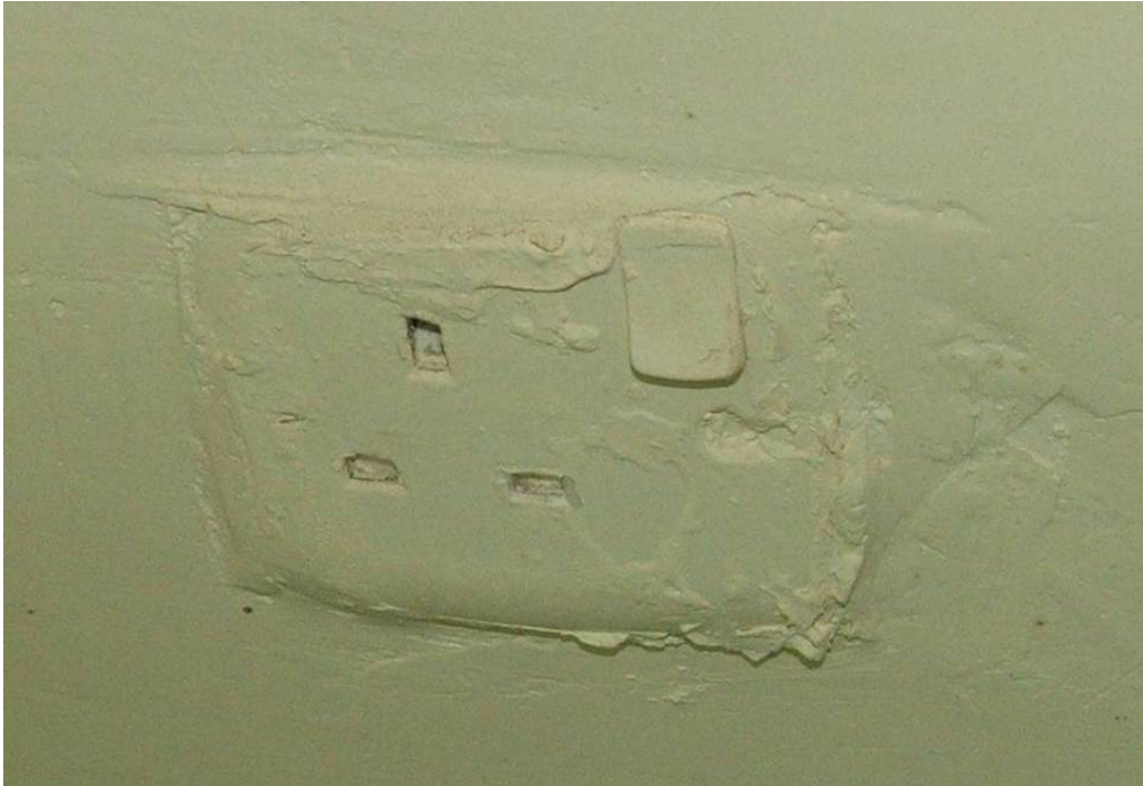
Site Photo 131. Electrical outlet covered with mortar and paint
