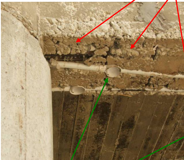
Site Photo 181. Concrete segregation and electrical conduit exposure
