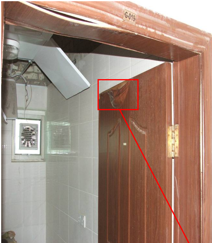
Site Photo 220. Door frame and door damage resulting from water leaks in cadet barracks
