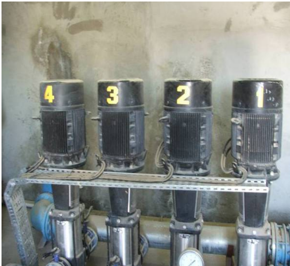
Site Photo 171. Four booster pumps in pump room
