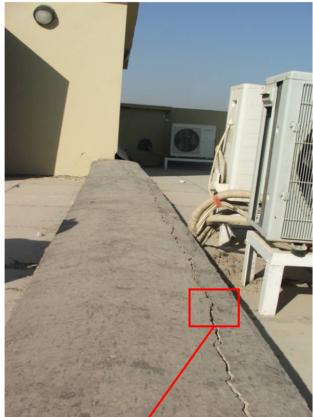
Site Photo 134. Expansion crack on roof
