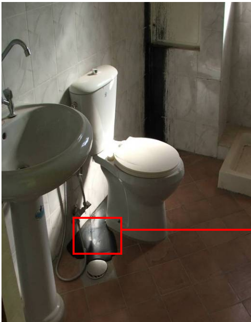
Site Photo 14. Tar leaking from roof to ground bathroom.
