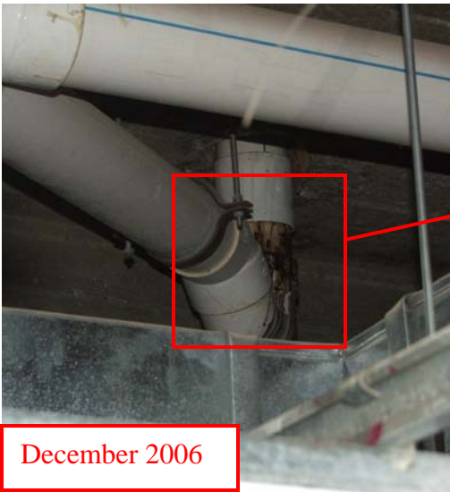
Site Photo 80. Leaking waste water from poorly sealed pipes
