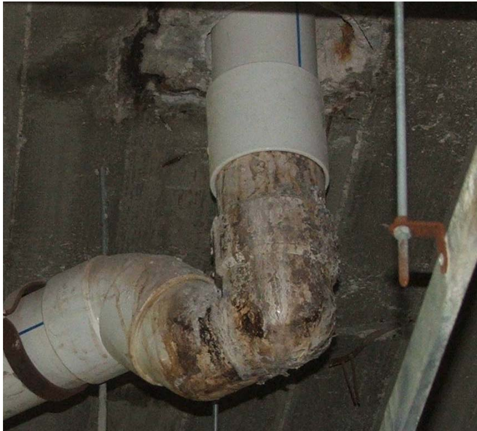
Site Photo 73. Significant plumbing leaks resulting from poorly sealed pipes
