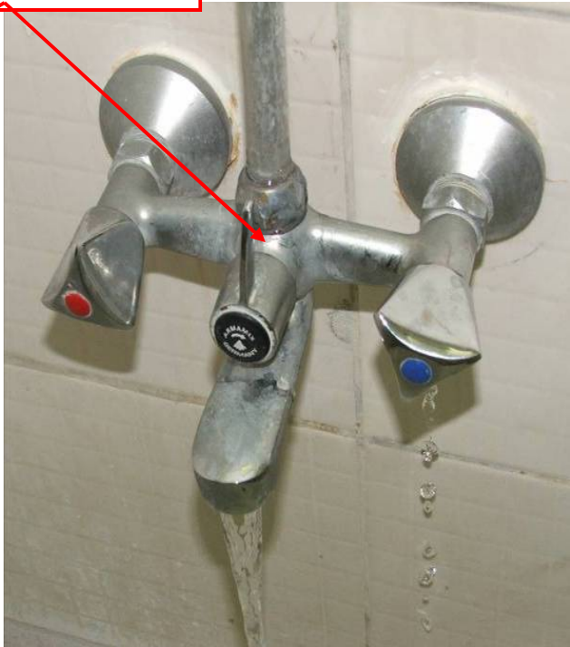
Site Photo 35. Leaking shower faucet in cadet barracks
