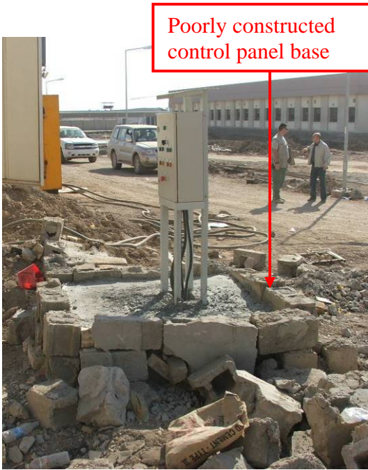
Site Photo 161. Dual pump station control panel base
