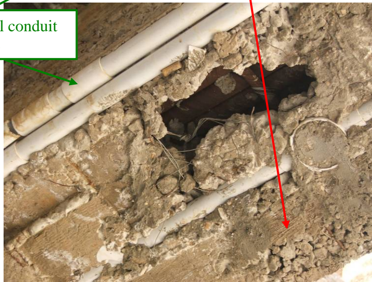
Site Photo 183. Concrete voids and electrical conduit exposure
