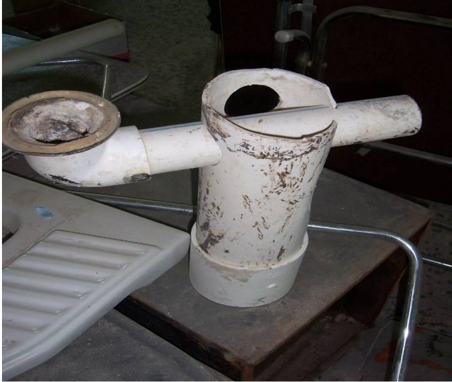
Site Photo 62. Non-industry standard plumbing fixtures
