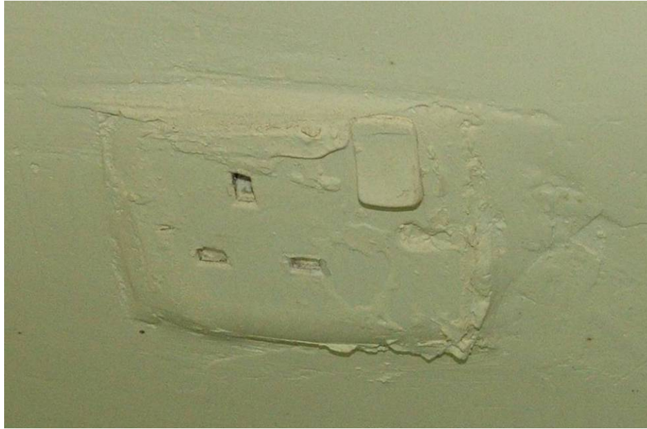
Site Photo 16. Unusable electrical outlet - mortar and paint inside the outlet
