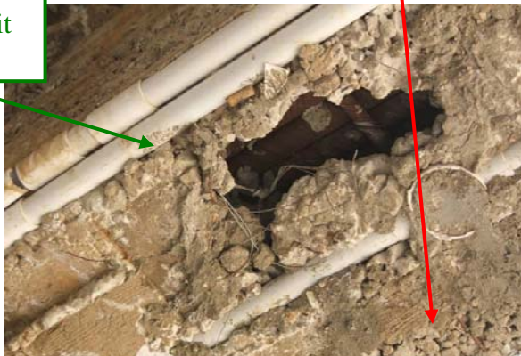
Site Photo 94. Concrete voids and electrical conduit exposure
