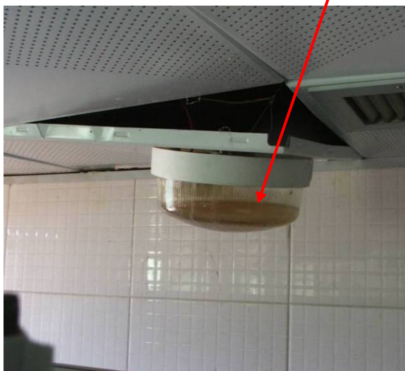
Site Photo 214. Urine-filled ceiling light
