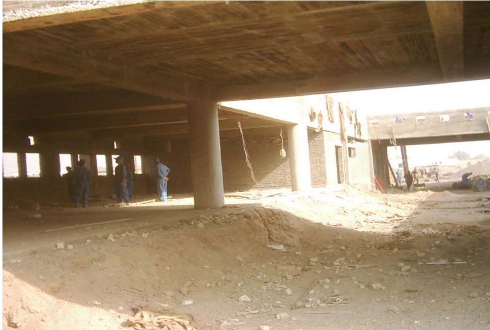
Site Photo 51. QAR daily report photo of interior of central laundry facility from the 26 November 2005 daily QA report (Photo courtesy of the USACE)
