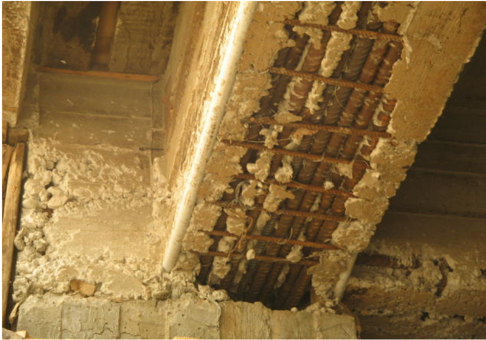
Site Photo 45. Improperly placed and exposed reinforcement bar, PVC conduit, and rust
