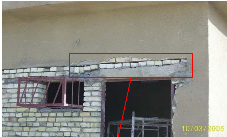
Site Photo 59. QAR provided photograph with caption “Armory warehouse bad lintel” (Photo courtesy of the USACE)
