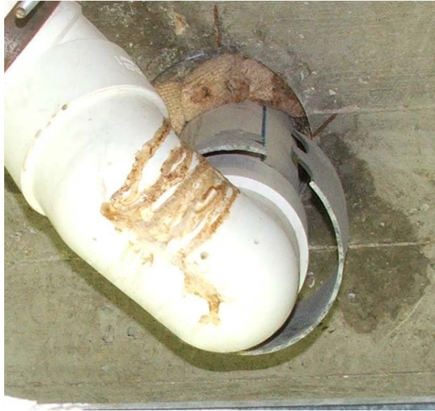
Site Photo 78. Example of poor sealing technique used by the contractor during initial construction
