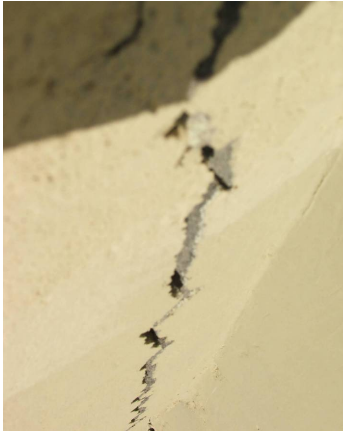
Site Photo 82. Exterior expansion crack
