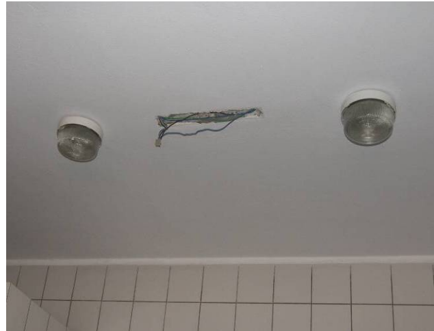
Site Photo 158. Poor installation of light fixture
