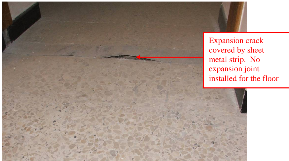
Site Photo 20. Interior expansion crack inside the instructors' barracks
