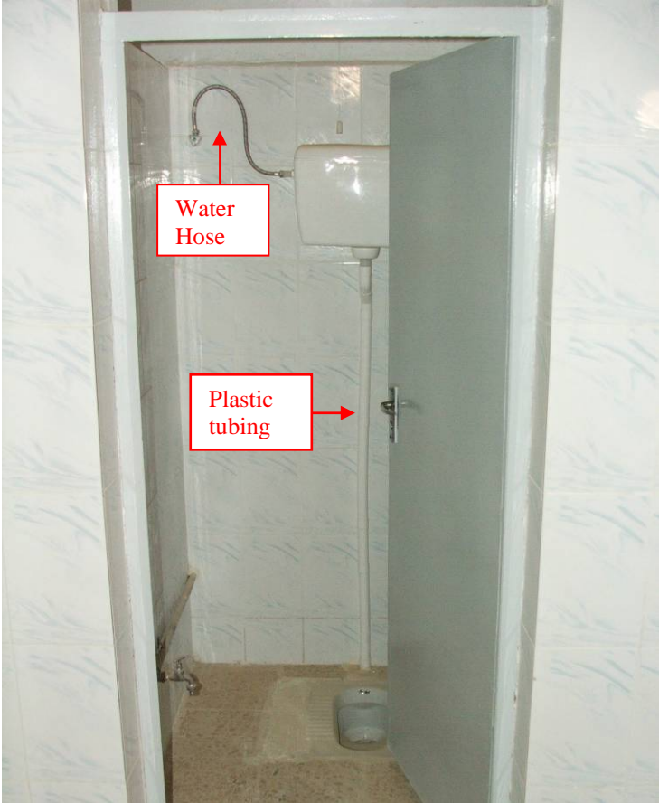
Site Photo 11. Water closet in ablution building
