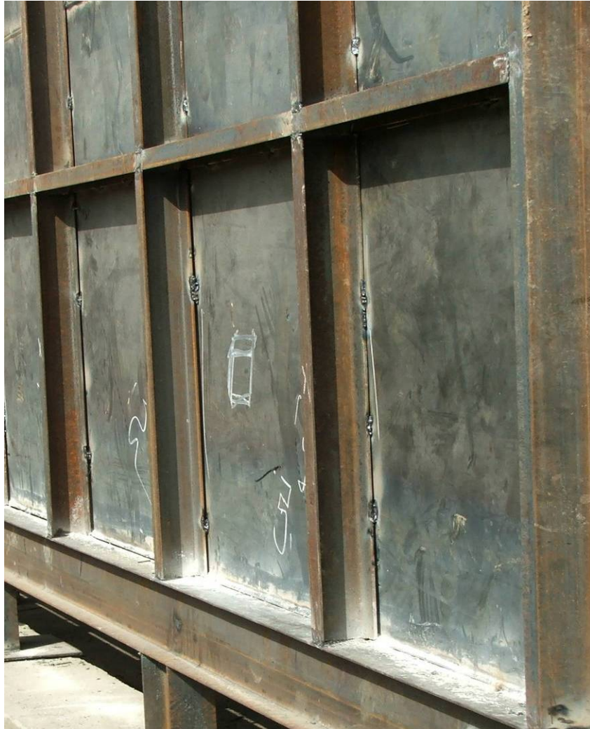
Site Photo 15. One of the tank's sidewalls showing steel plates spot welded to frame
