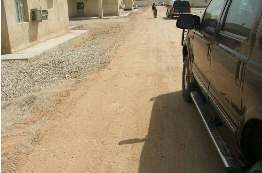
Site Photo 16. Compacted subbase material for one of the new roads under construction
