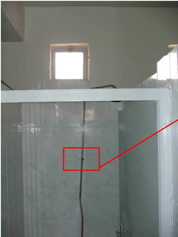
Site Photo 17. Shower fixture in the ablution building
