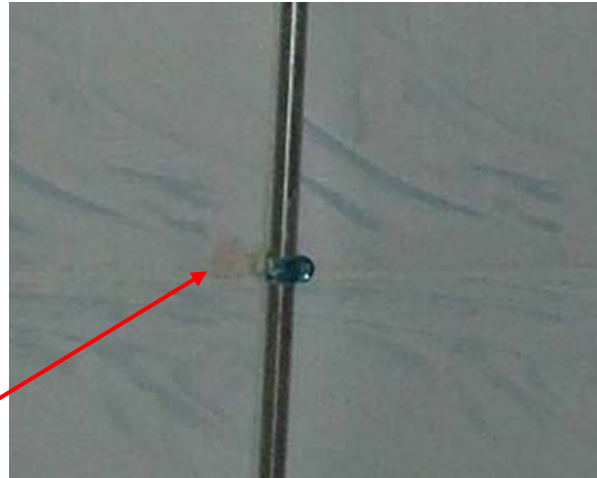
Site Photo 18. Close up view of clamp
