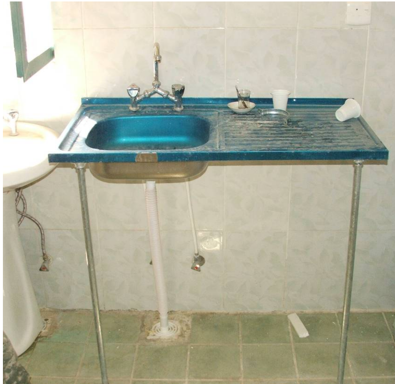
Site Photo 9. Medical clinic exterior sink
