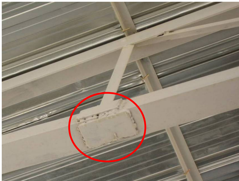
Site Photo 24. Spliced bottom chord on motor pool roof
