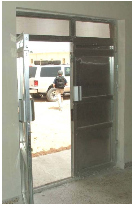
Site Photo 5. Aluminum doors at front entrance to the barracks sleeping quarters
