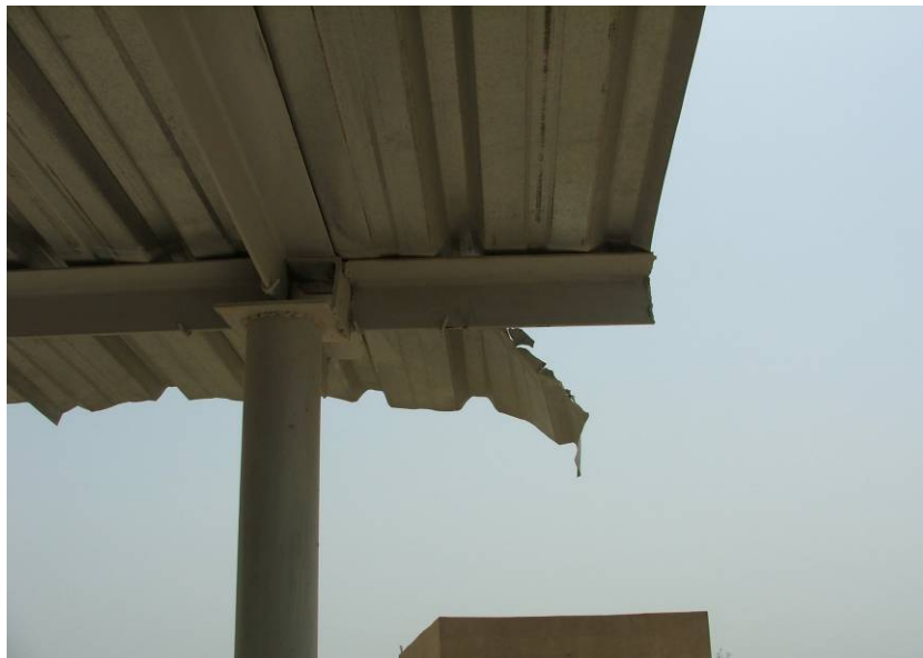
Site Photo 15. Torn sheeting at one end of the parking sunshade
