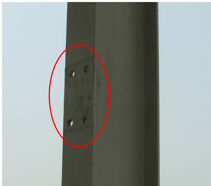
Site Photo 22. Bolt holes in flange of a steel H-column at the motor pool
