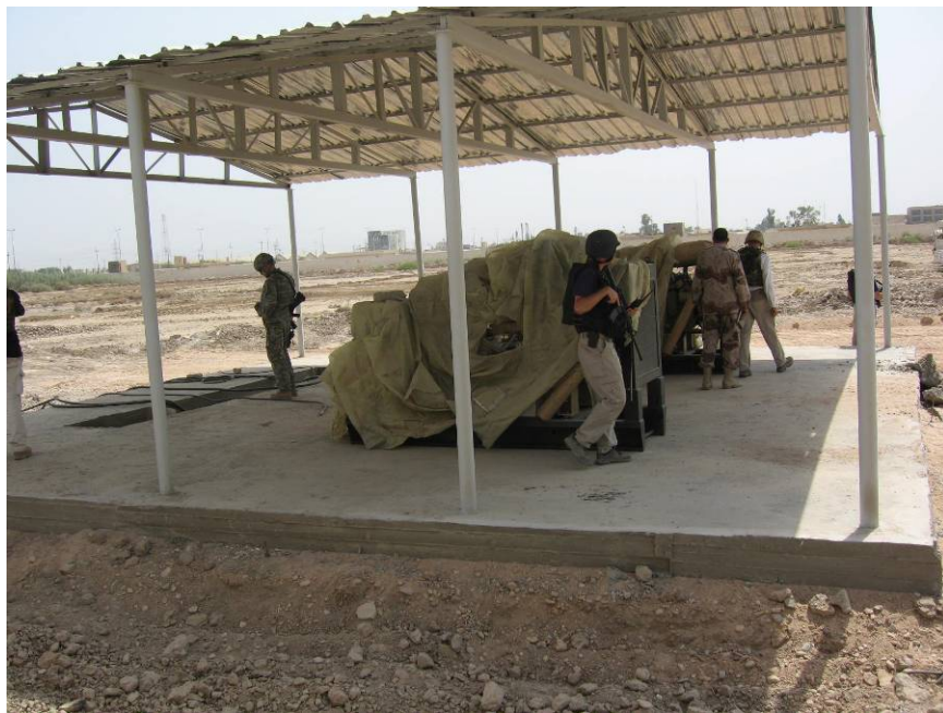
Site Photo 25. Generator shed and two generators (covered with tarps)
