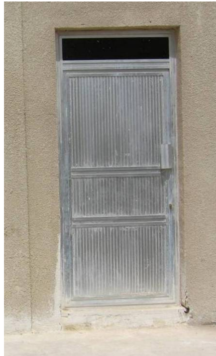
Site Photo 6. Aluminum door at rear entrance to the barracks sleeping quarters
