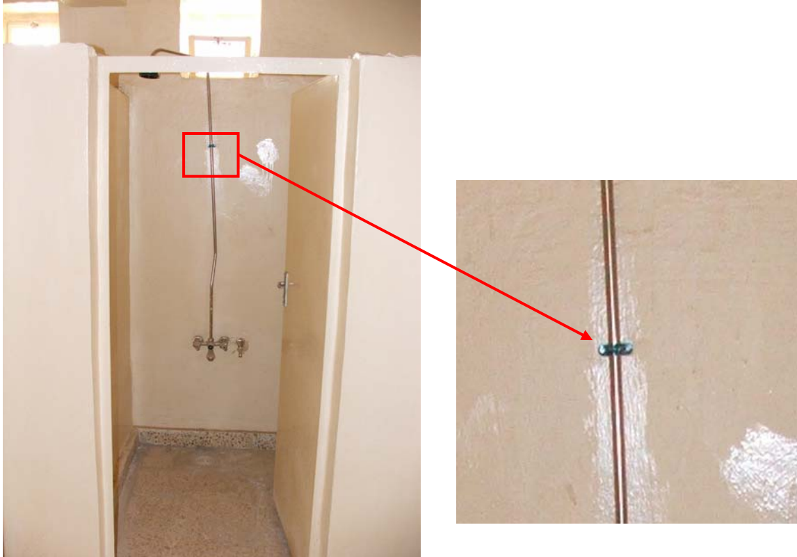
Site Photos 26 and 27. Single screw clamp holding the thin metal water pipe to the wall.
