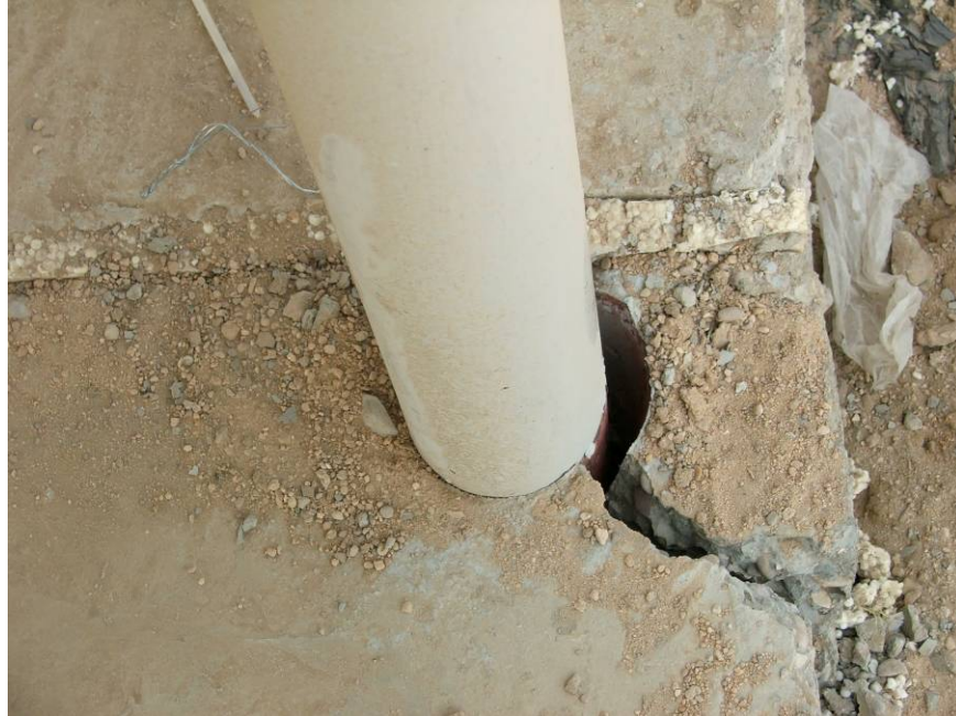
Site Photo 16. Broken concrete at column base in the parking sunshade
