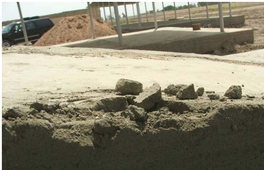
Site Photo 20. Crumbling mortar at the surface of the vehicle ramp
