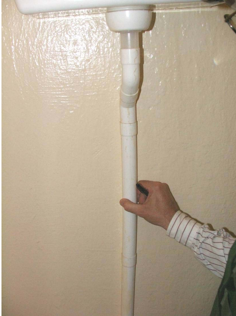
Site Photo 12. Close-up of plastic tubing used in ablution building water closets
