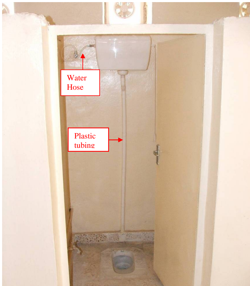
Site Photo 11. Water closet in ablution building
