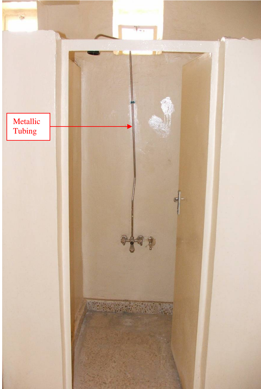
Site Photo 9. Shower in ablution buildings
