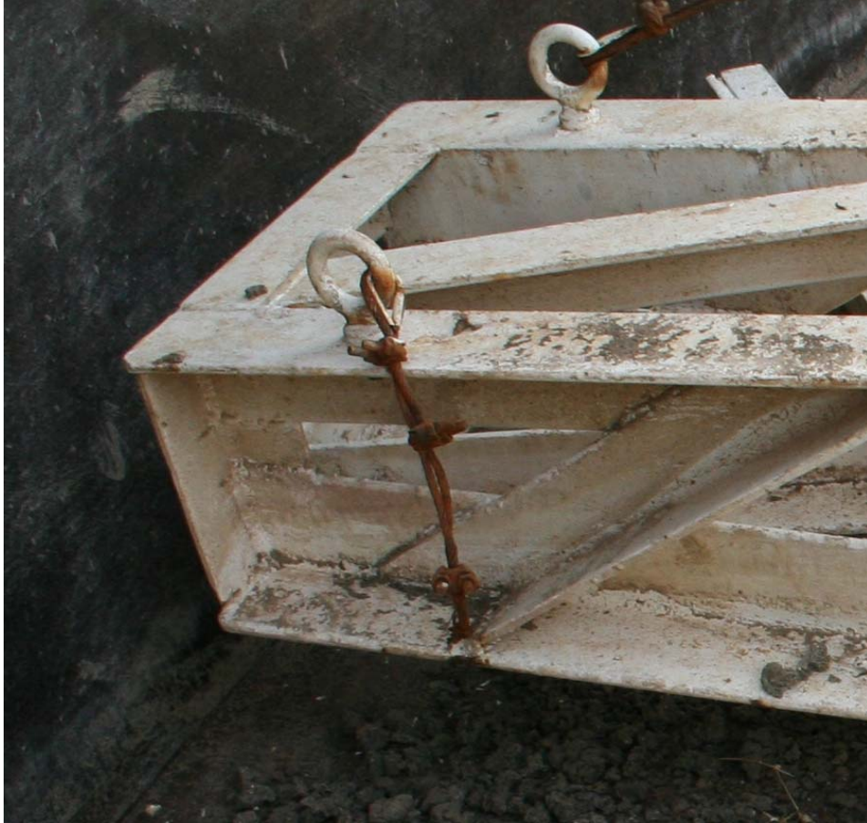
Site Photo 1. Cable failure caused the clarifier arm assembly to drop to the bottom of the tank.
