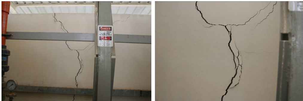
Site Photos 11 and 12. Vertical cracks were present in the inner rear wall of the pump station.
