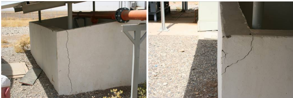
Site Photos 17 and 18. Vertical cracks wound their way to the outer corners of the rear wall.
