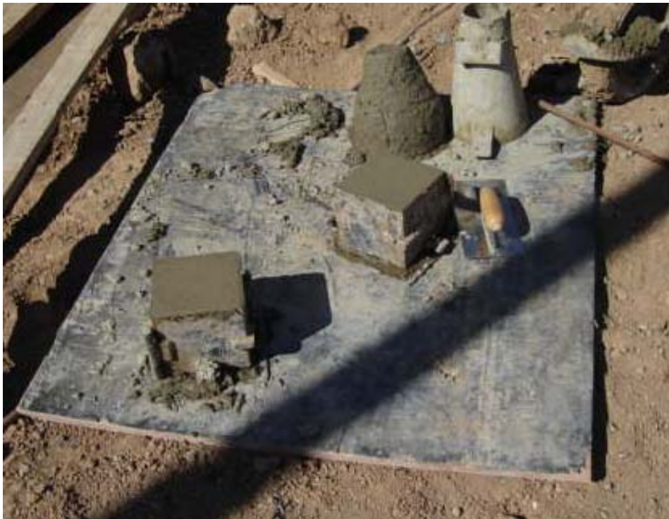
QA Photo 4. Slump test and 2 cube samples taken for laboratory concrete strength testing (from QA report 26 Oct 2005).
