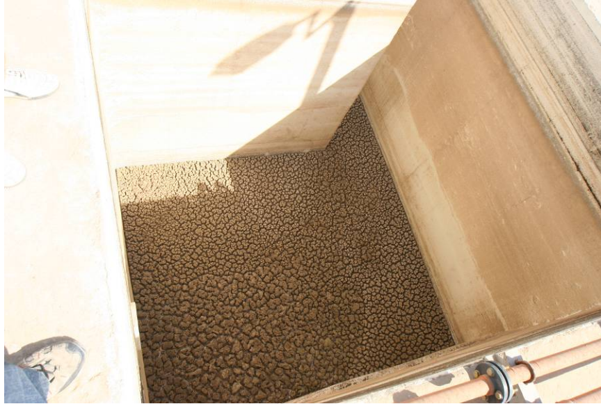
Site Photos 20. Prefilter chlorination tank floor was covered with solids.
