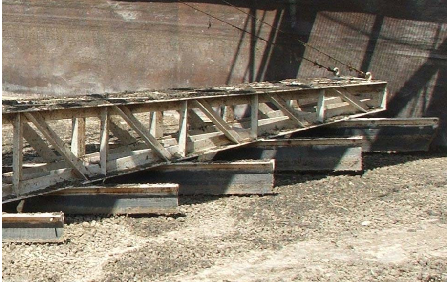
Site Photo 9. The rubber scrapers hang freely on the side that did not experience cable failure.
