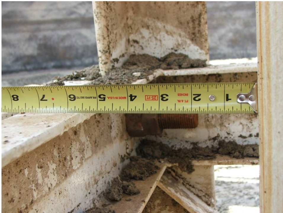
Site Photo 5. Main shaft was positioned approximately 5 5/8 inches from the static frame.
