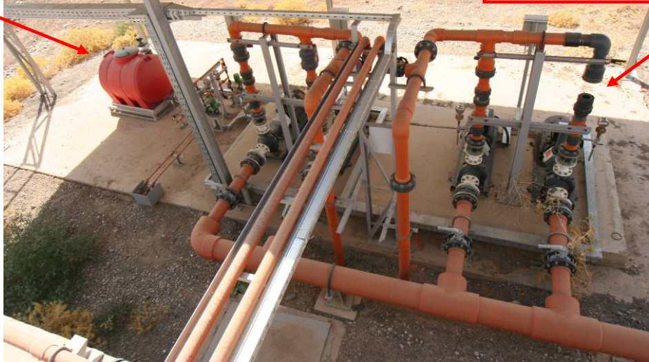
Site Photo 21. Effluent supply and back flush inlet piping systems.
