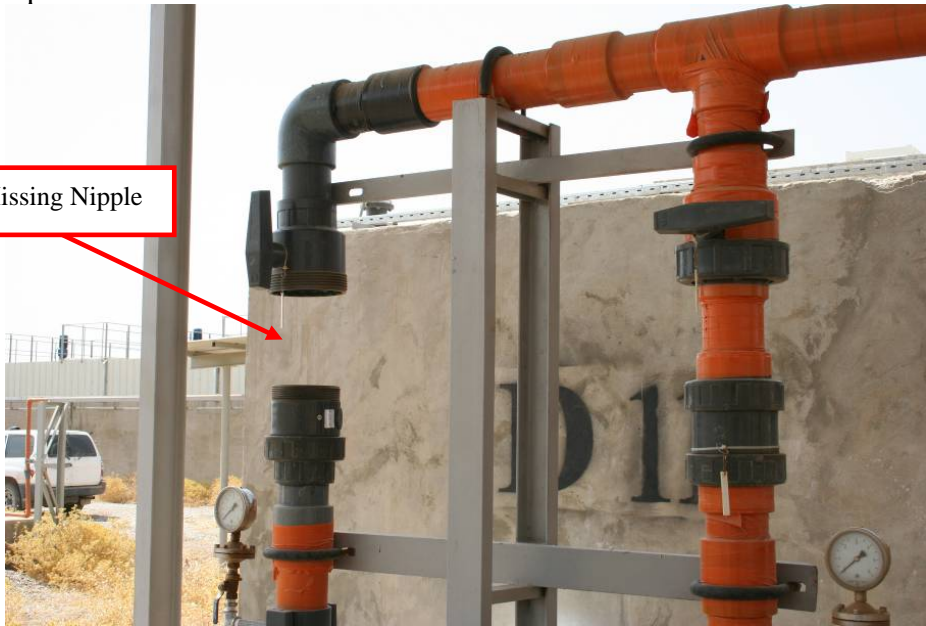
Site Photo 22. Missing nipple meant that back flushing could not be performed.
