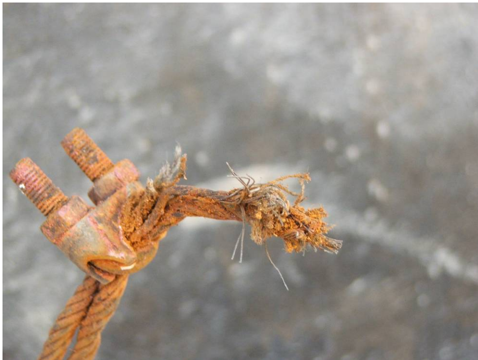
Site Photo 2. Support cable was frayed and corroded.
