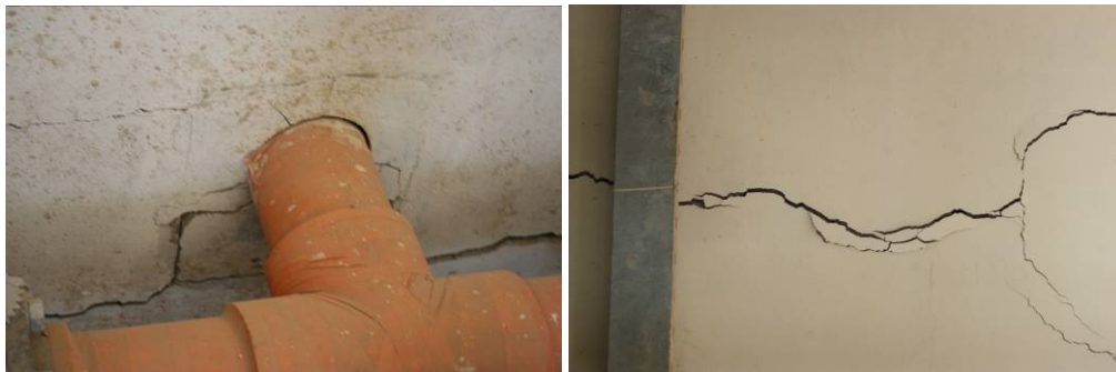
Site Photos 13 and 14. Horizontal wall cracks along floor and middle of the wall.
