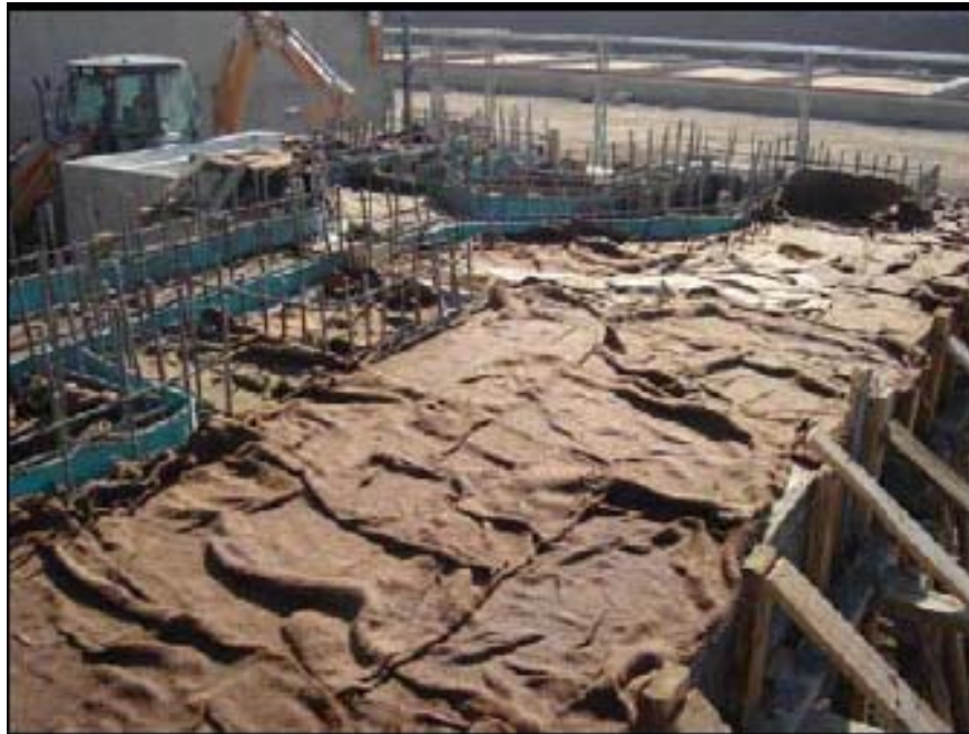
QA Photo 8. Concrete covered with burlap to prevent too rapid drying and decreased strength (from QA Report 3 Oct 2005).
