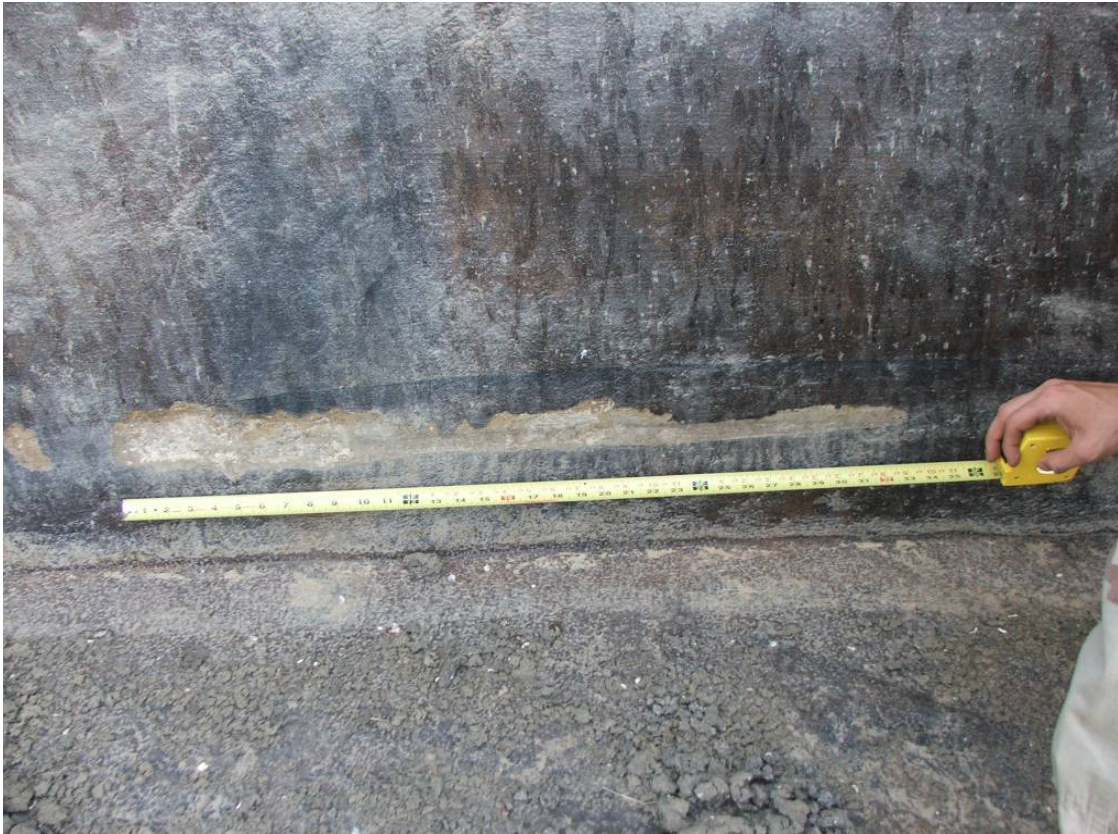
Site Photo 3. Gouge mark approximately 33 inches long.
