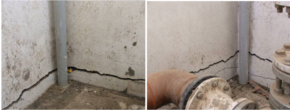
Site Photos 15 and 16. Horizontal cracks near the floor at opposite corners of the G-03 building.
