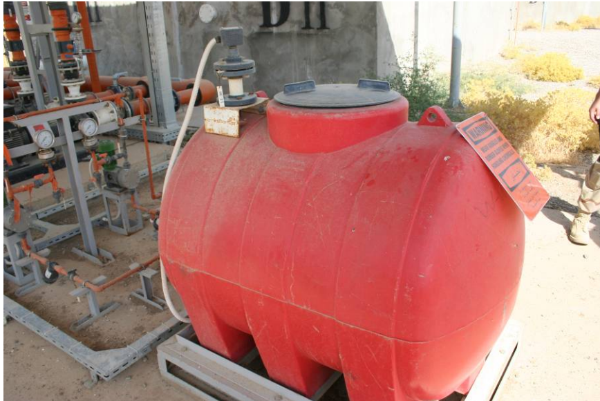
Site Photos 19. Chlorination system included a holding tank for Sodium Hypochlorite (NaOCL).
