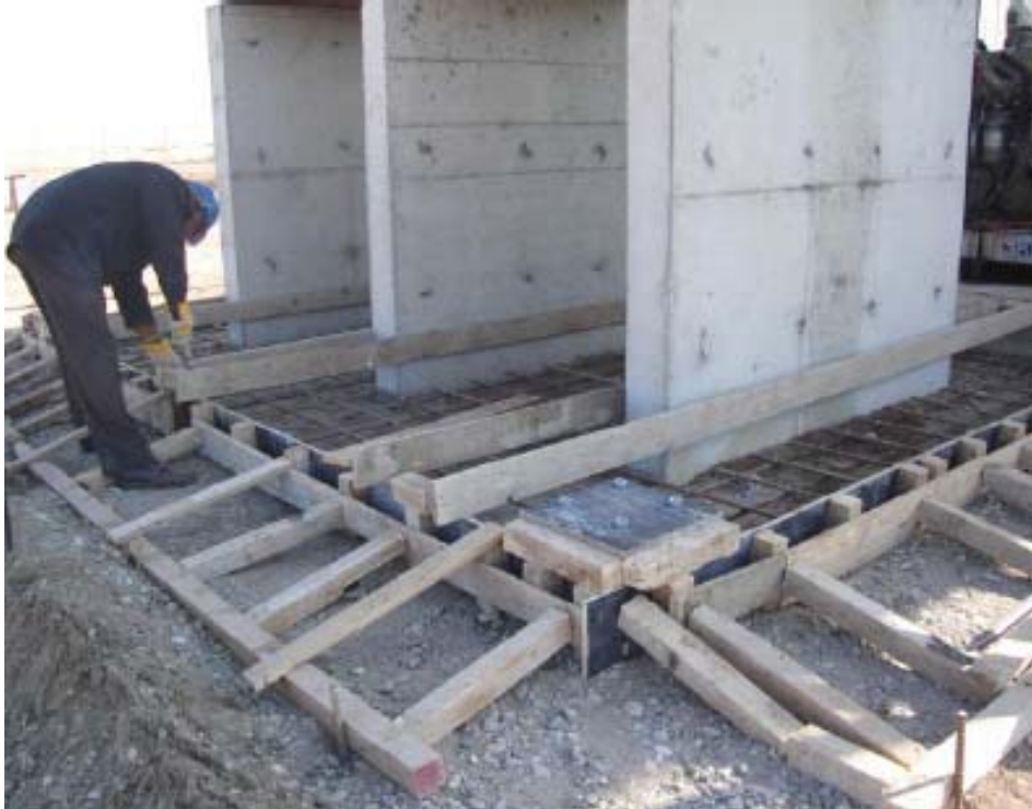
QA Photo 5. Flatwork form with clear / sufficiently sized lumber and proper brace placement (from QA Report 14 Dec 2005).
