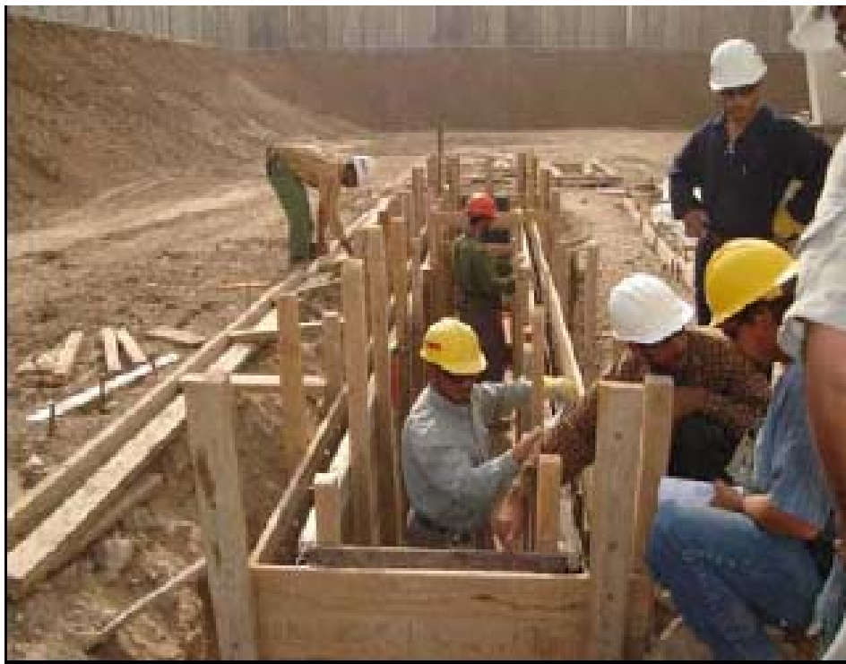
QA Photo 6. Good form techniques were used to build a sub-grade foundation with supervisors on site (from QA Report 11 Oct 2005).
