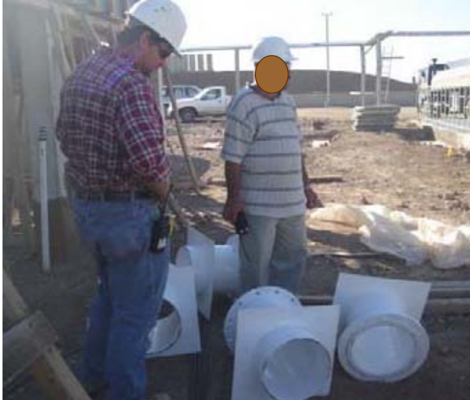
QA Photo 3. QC Manager inspected and rejected pipe flanges (from QA Report 11 Sep 2005).
