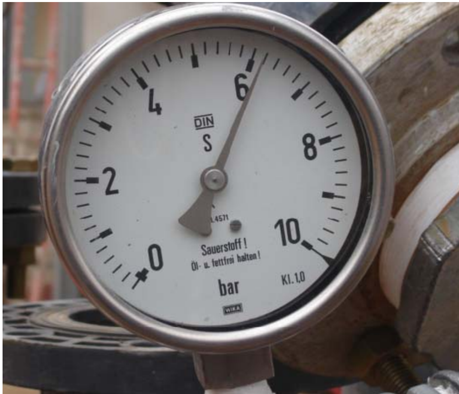
QA Photo 2. Hydro-testing a pipe line between tanks (from QA Report 23 Dec 2005).
