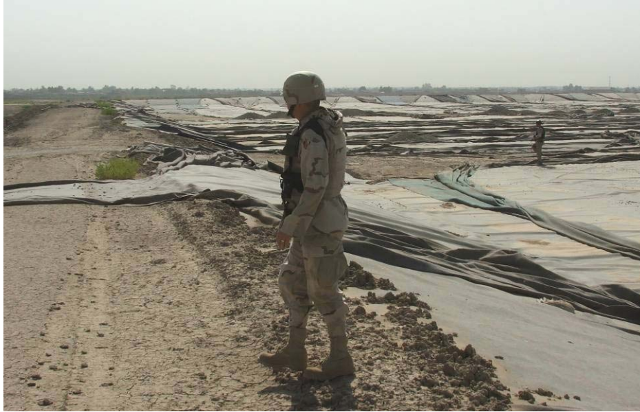
Site Photo 6. Section of the perimeter berm requiring remedial work to anchor the liner
