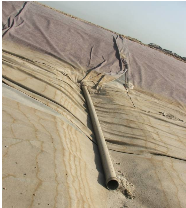
Site Photo 8. HDPE Leachate Collection Pipe
