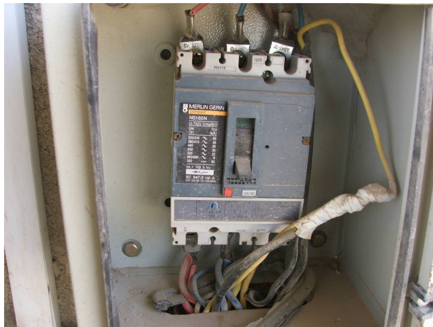
Site Photo 14: Wiring to one of the dedicated circuits
