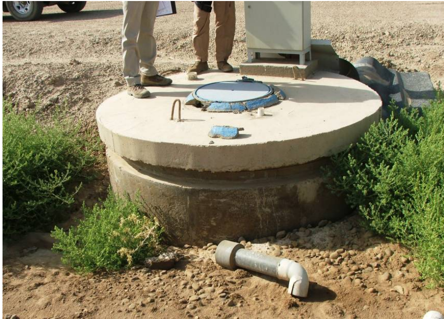
Site Photo 9. Pump enclosure with broken vent pipe and access cover ring
