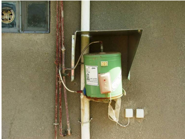
Site Photo 15. Water heater outside administration building
