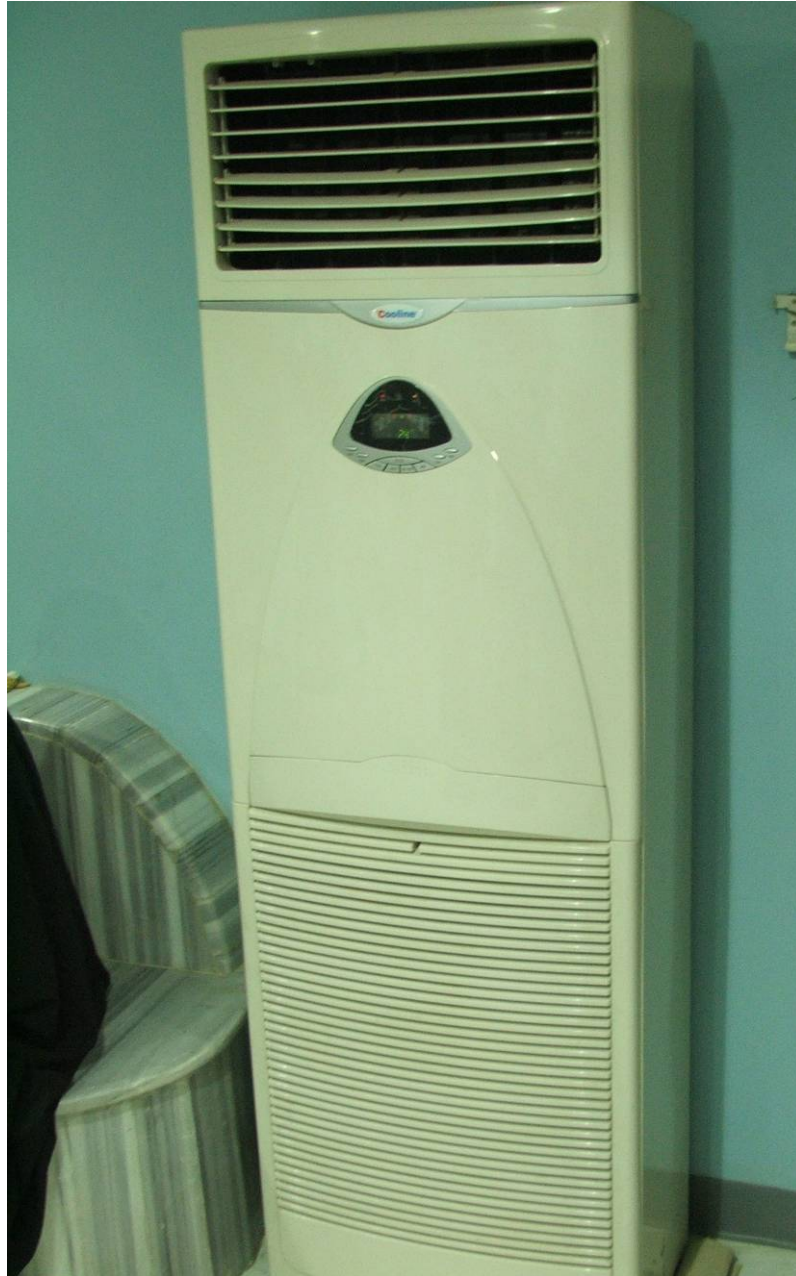
Site Photo 7. Stand alone HVAC unit in the clinic waiting area
