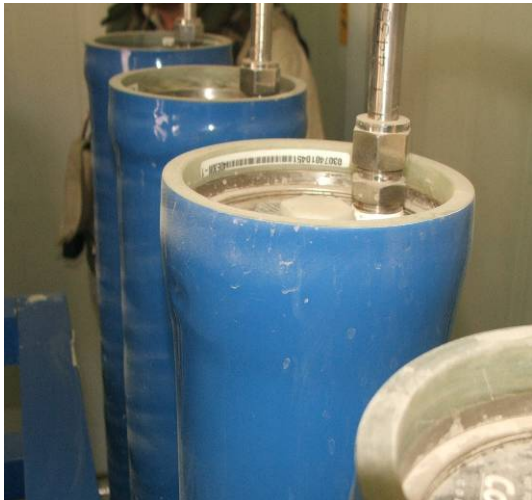
Site Photo 11. Pressure vessels containing RO membranes
