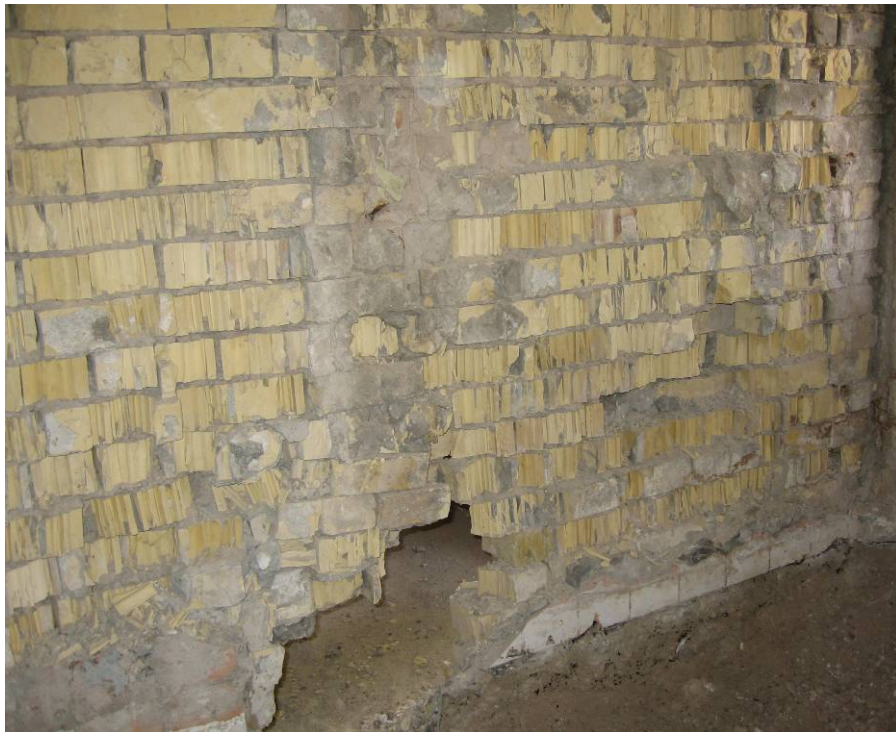
Site Photo 13. Existing brick walls in building B1 after demolition of interior finishes
