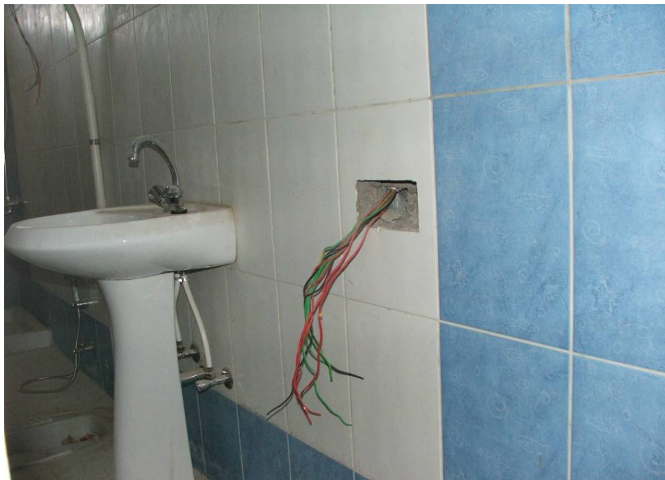
Site Photo 16. One of the bathrooms in building B1 rear section after ceramic tile placement.
