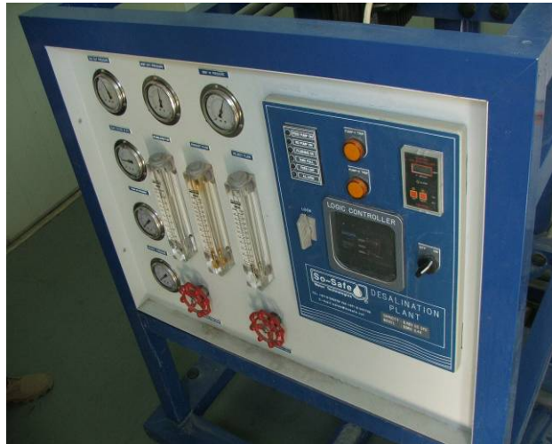
Site Photo 12. RO control panel
