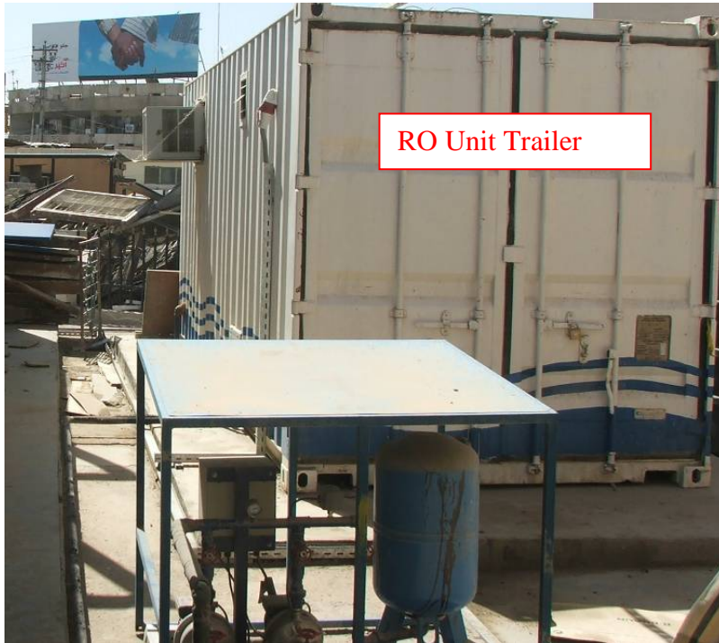
Site Photo10. Container housing the RO unit
