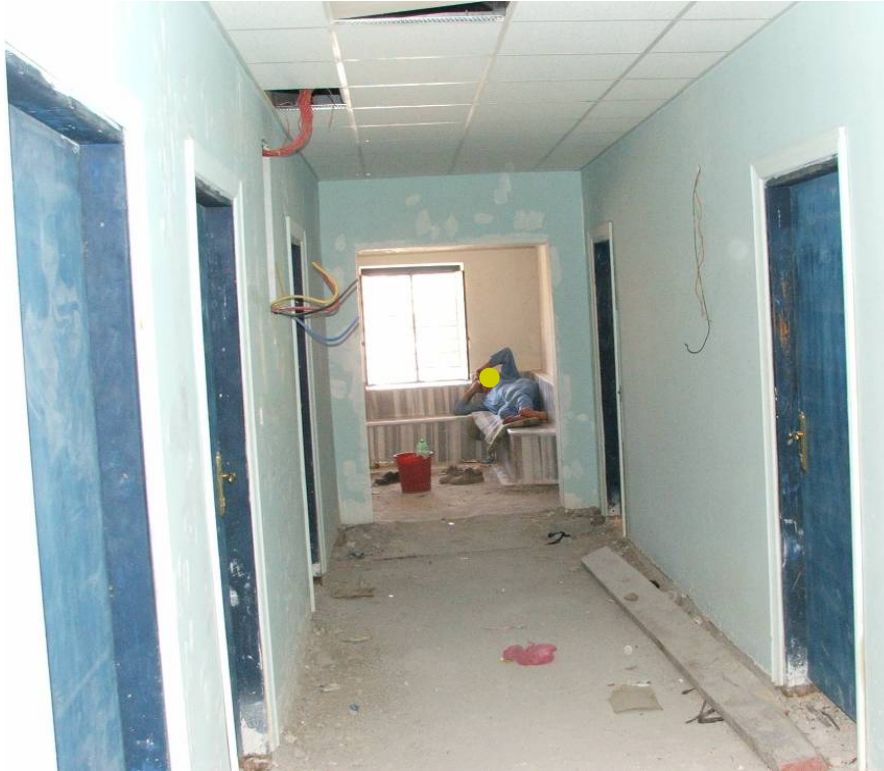
Site Photo 15. Plastered and painted walls in the rear section of building B1.
