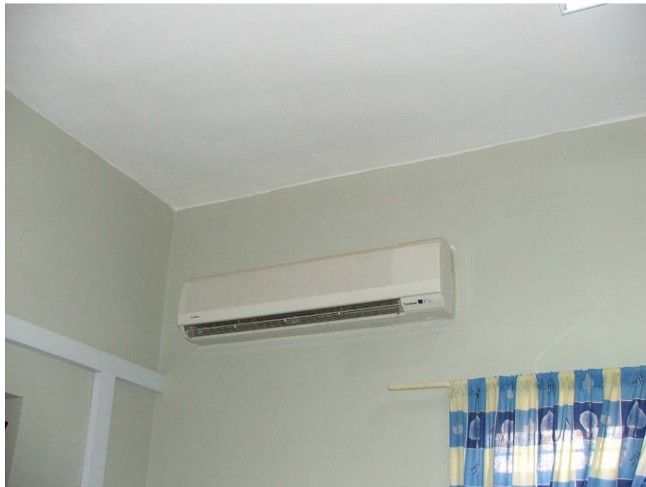
Site Photo 3. Split system HVAC evaporator unit in building B2
