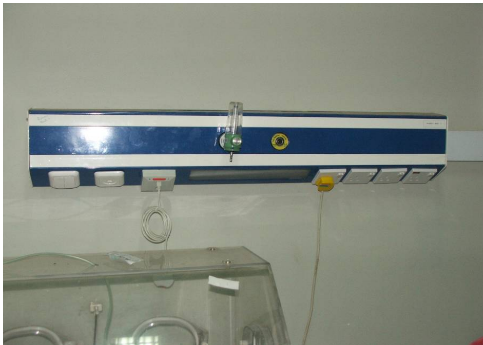
Site Photo 5. Electrical outlet box in patient ward in building B2
