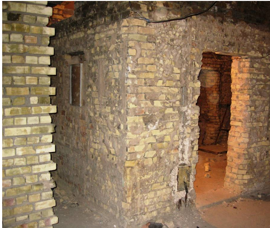
Site Photo 7. Existing brick walls in building B1 after demolition of interior finishes
