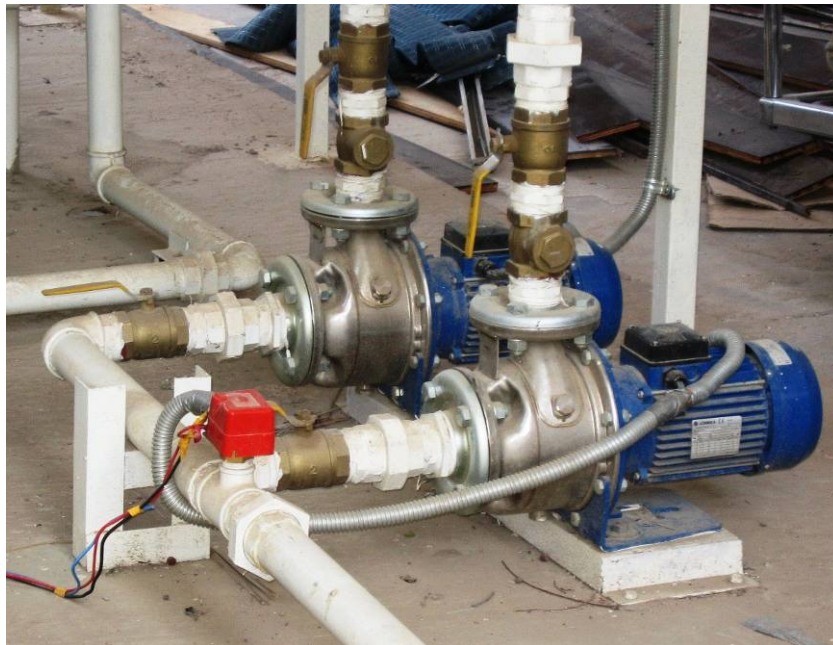
Site Photo 12. Circulation pumps
