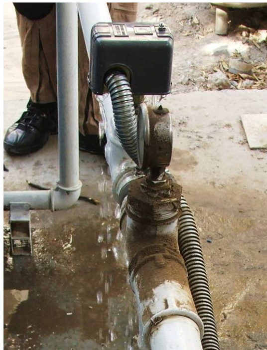
Site Photo 14. Leak at a solenoid valve
