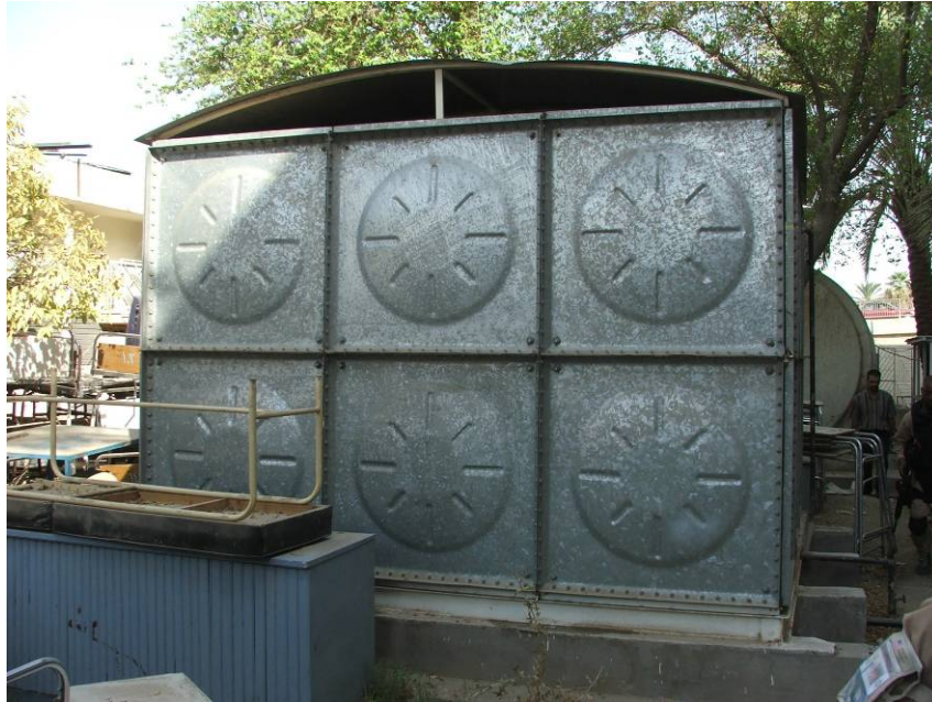
Site Photo 11. 40 m 3 galvanized steel water tank
