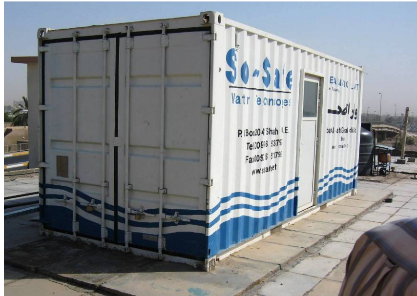
Site Photo 5. Container housing the RO unit
