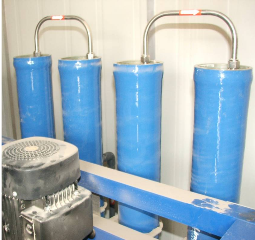
Site Photo 6. Pressure vessels containing RO membranes
