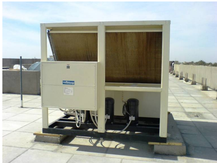
Site Photo 12. Roof top HVAC unit (Photo provided by USACE)
