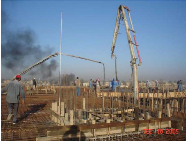
Site Photo 2. Pump truck booms delivering concrete for roof slab pour (Photo provided by USACE)
