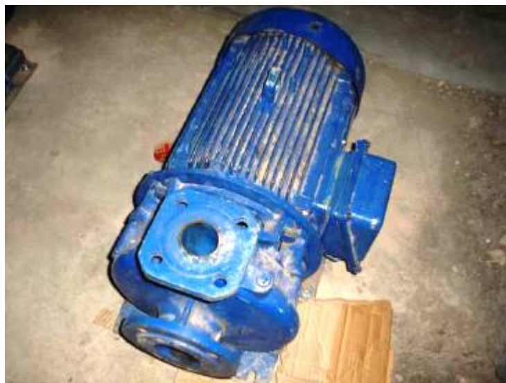
Site Photo 15. Domestic water circulation pump (Photo provided by USACE)
