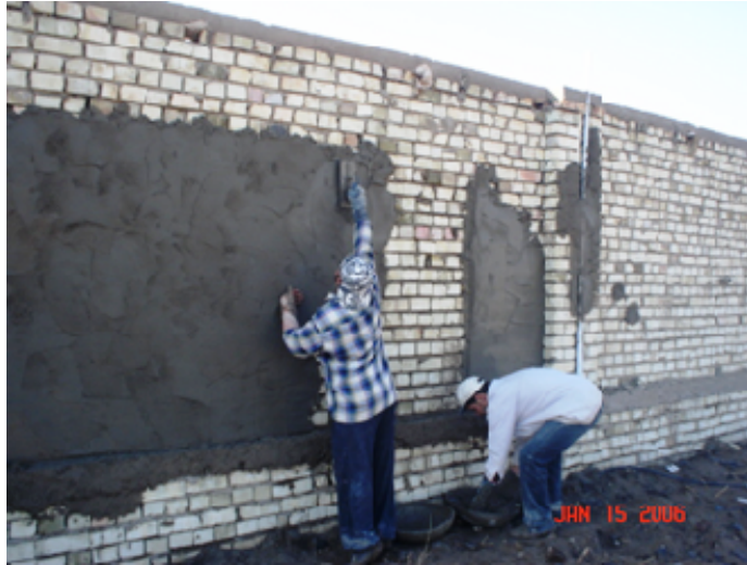
Site Photo 1. Rendering the Brick Perimeter Wall with a Cement Plaster (Photo provided by USACE)
