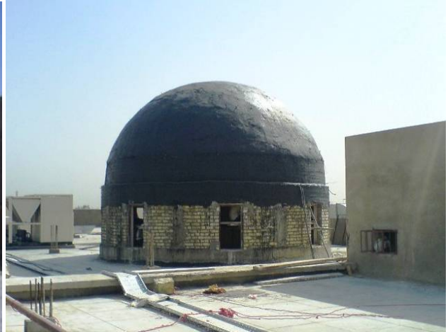
Site Photo 11. Dome after concrete placement and waterproofing (Photo provided by USACE)
