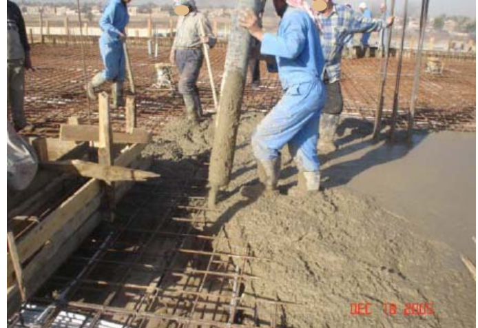
Site Photo 3. Concrete placement for roof slab pour (Photo provided by USACE)
