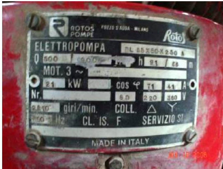
Site Photo 16. Factory plate for fire hydrant system pump (Photo provided by USACE)
