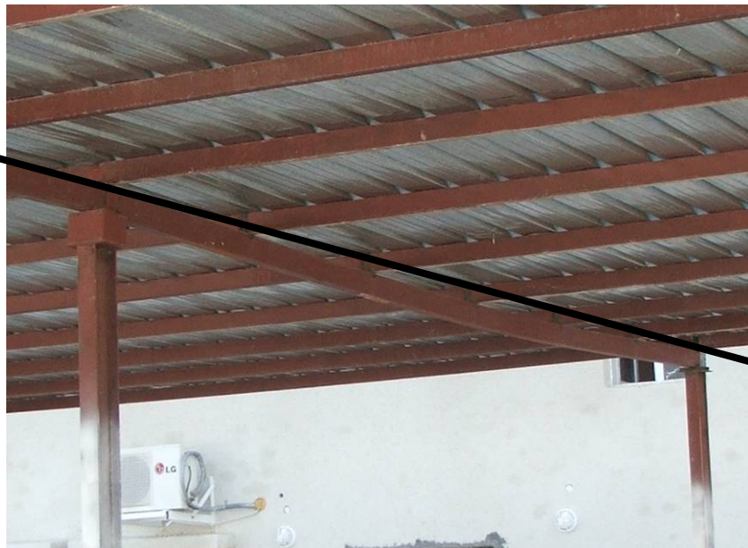
Site Photo 20: Deflection of the rectangular tubular steel cross member in contrast to a straight line between support points
