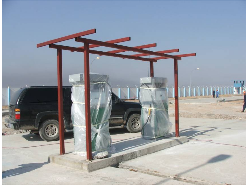
Site Photo 13: Fuel dispensing units
