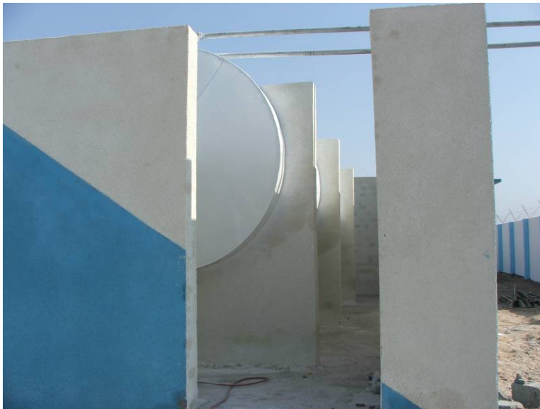
Site Photo 12: Fuel storage tank with wall enclosure
