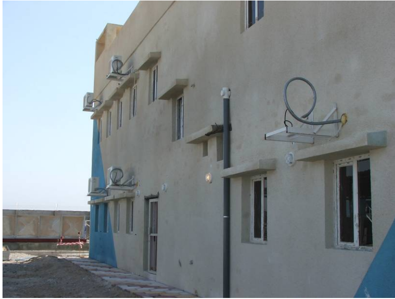
Site Photo 10: Exterior building light
