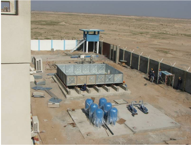
Site Photo 14: (6) hydrophumatic pressure vessels (left foreground), (2) water distribution pumps (right foreground), and single water storage tank
