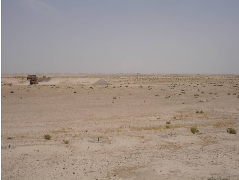
Site Photo 1: IHP Barracks project site during initial construction (Photo courtesy of the USACE)
