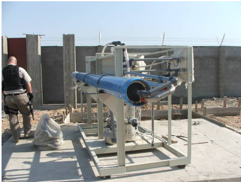
Site Photo 15: Reverse osmosis filtration unit
