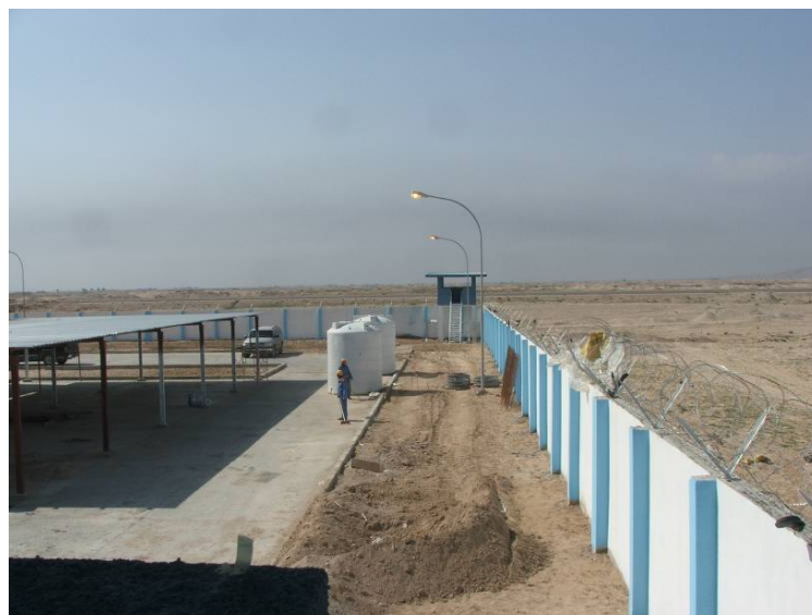
Site Photo 9: 8-meter light poles
