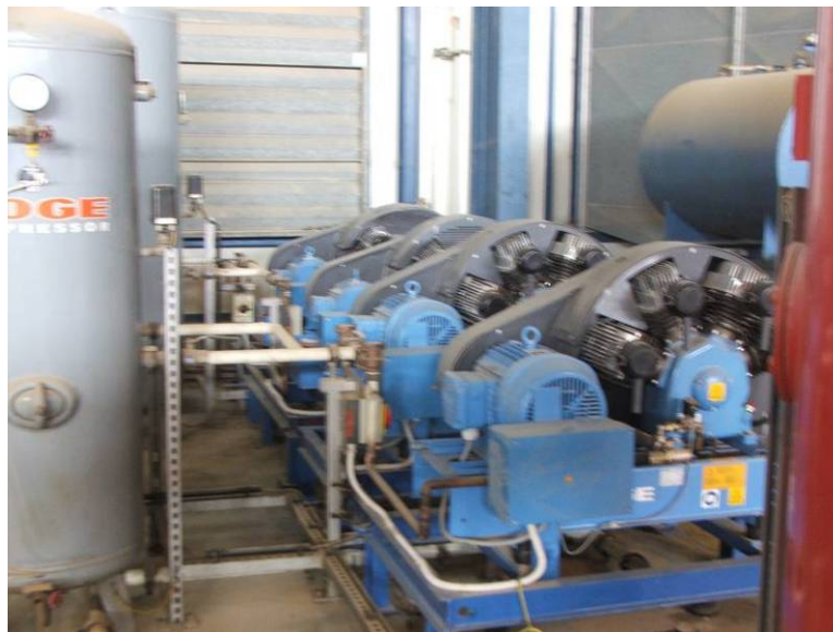
Site Photo 18. Air compressor units located at plant facility
