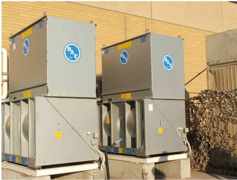
Site Photo 17. HVAC cooling towers located at fire station
