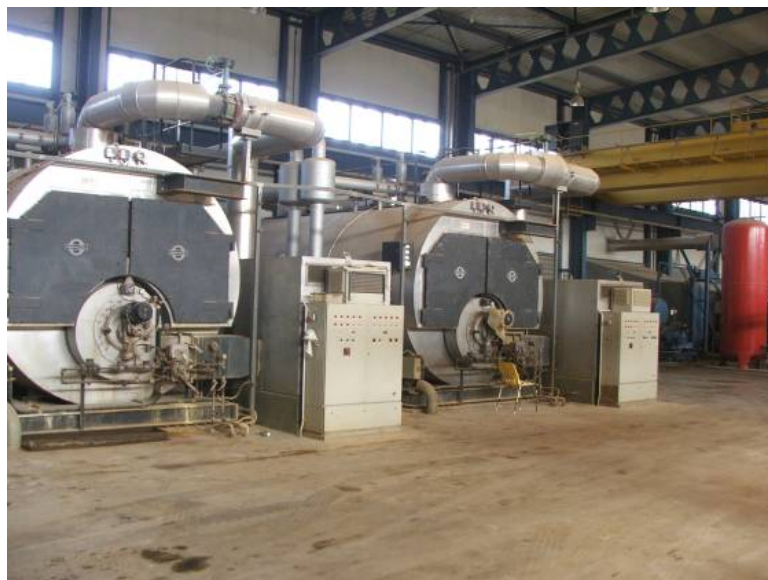
Site Photo 19. Boiler units located at plant facility
