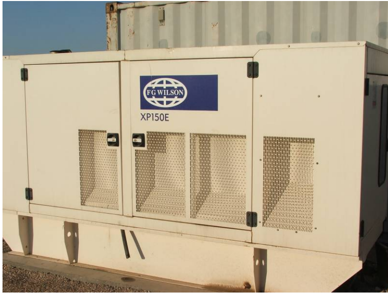
Site Photo 16. Generator set located at the fire station
