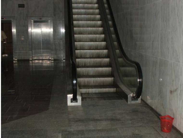
Site Photo 9. Escalator and two elevators (left) at passenger terminal
