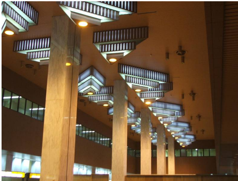
Site Photo 12. Operational lighting in ticket area of passenger terminal
