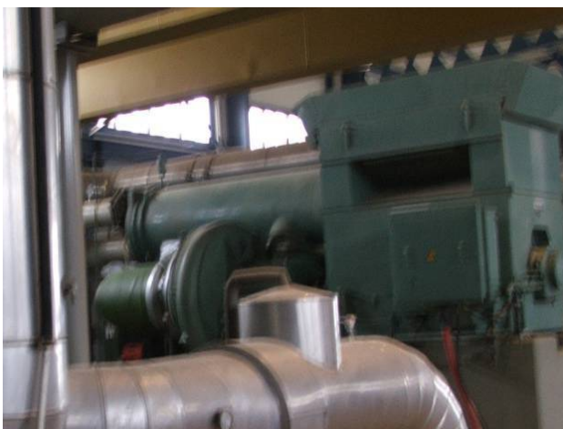
Site Photo 5. Chiller unit inside plant facility
