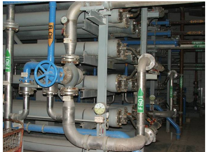
Site Photo 4. Reverse Osmosis filters
