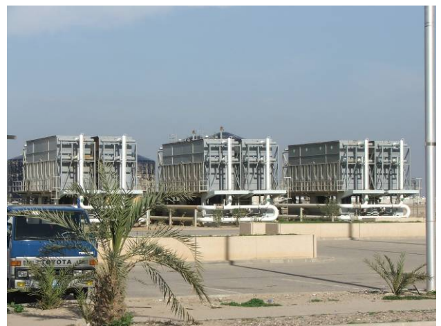
Site Photo 6. Three pairs of the cooling towers located adjacent to the plant facility
