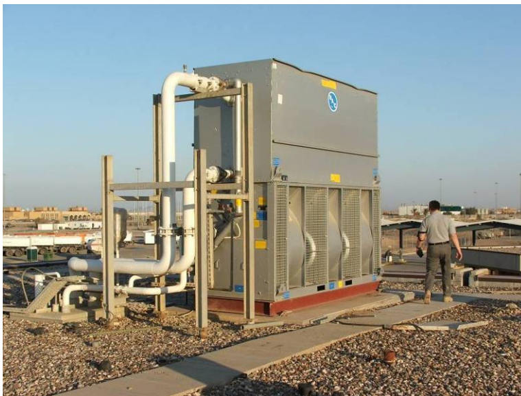
Site Photo 14. Roof mounted cooling tower located at ATC administration building
