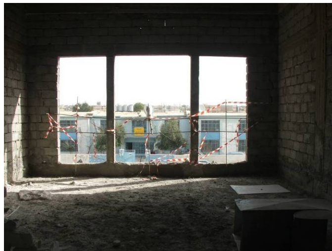
Site Photo 40. Example of windows without window frames
