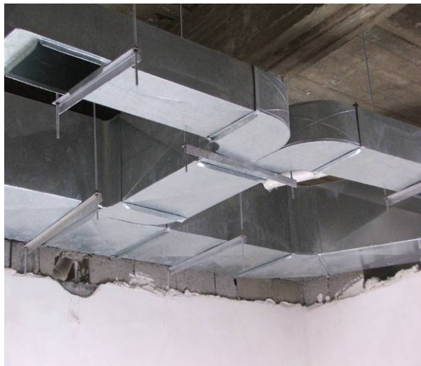
Site Photo 45. Ventilation ductwork
