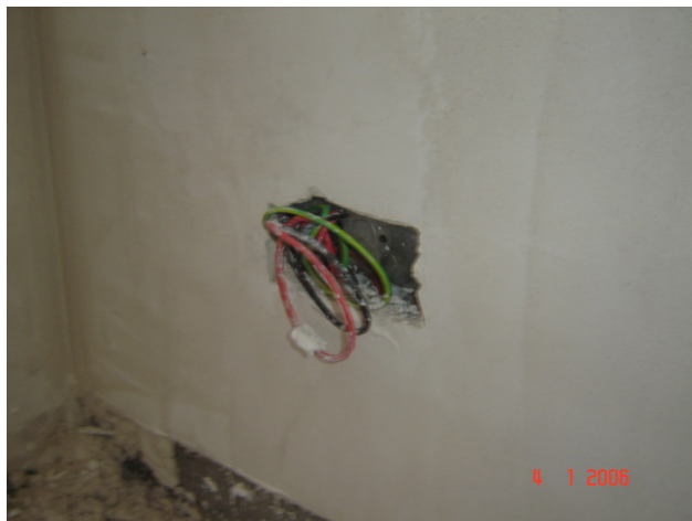
Site Photo 34. Electrical wiring (Photo courtesy of USACE)
