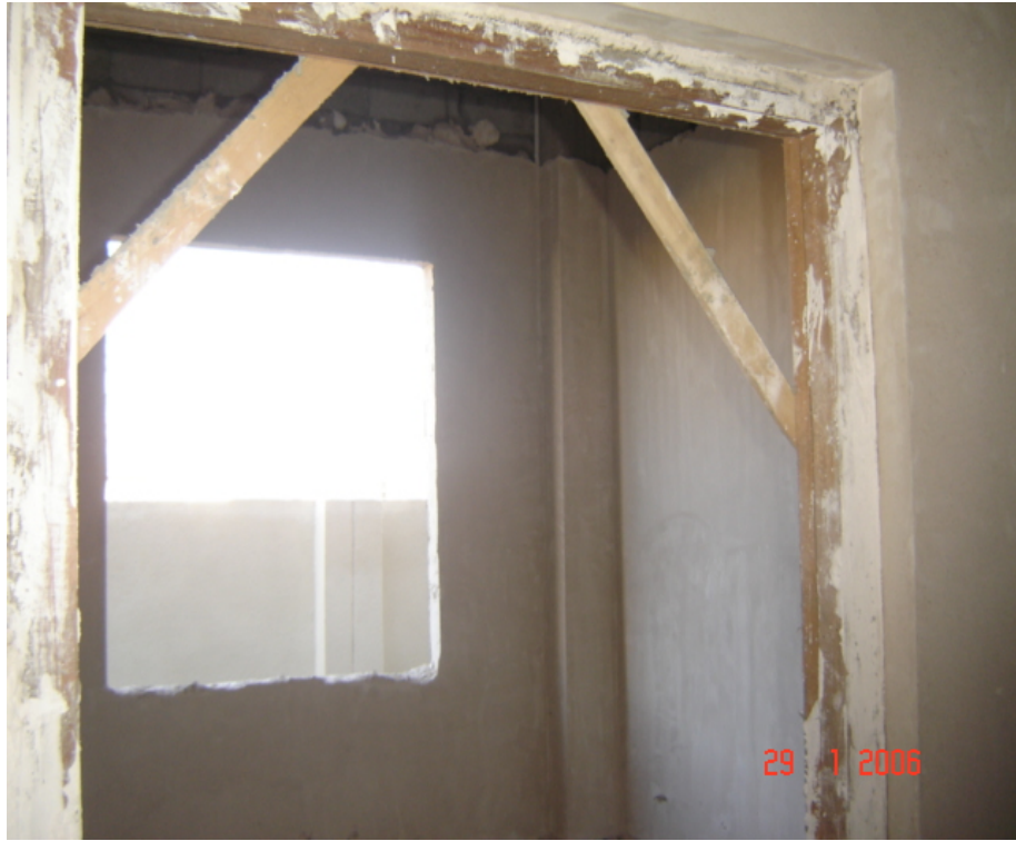
Site Photo 74. Example of window without window frame and grilles (Photo courtesy of the USACE)
