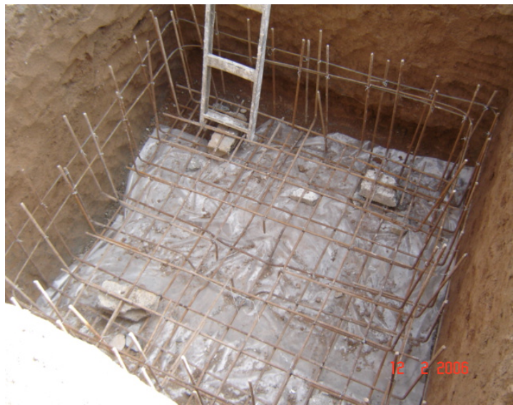
Site Photo 63. Excavated hole for septic tank (Photo courtesy of the USACE)
