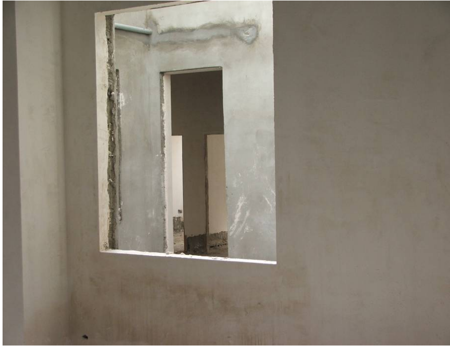
Site Photo 49. Window opening without window frame
