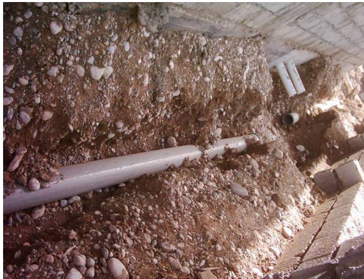
Site Photo 83. Partial installation of sewer drain (Photo courtesy of the USACE)
