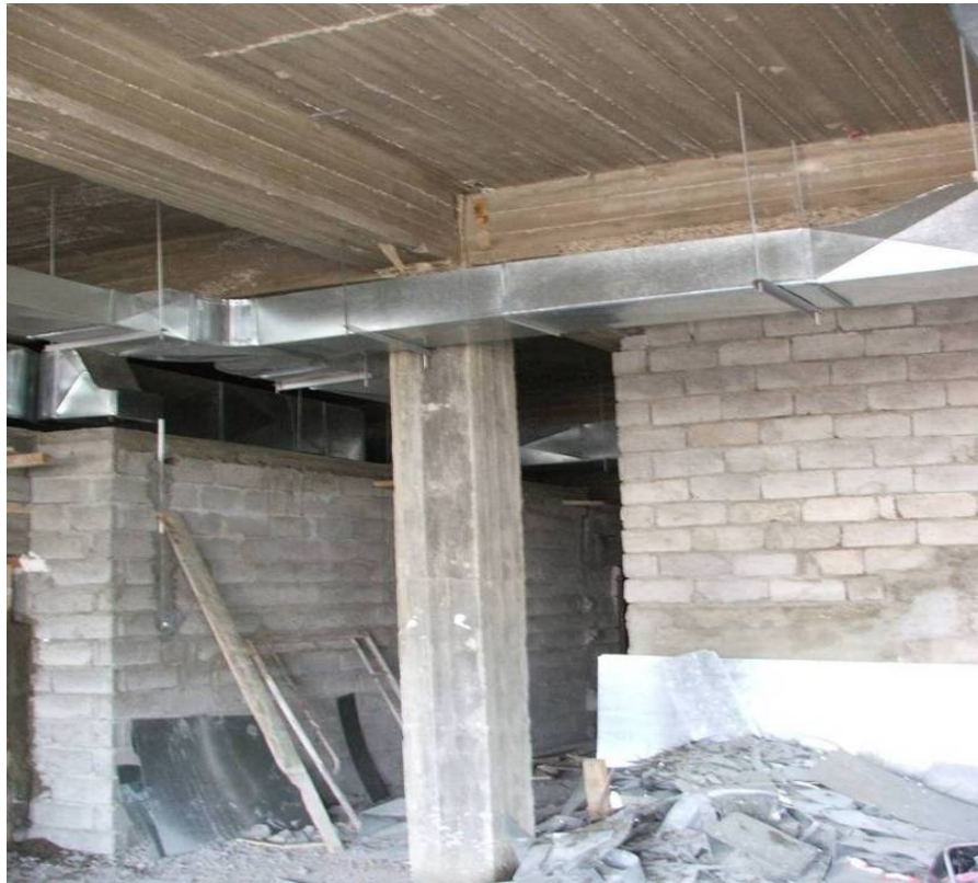
Site Photo 4. Column that is not plumb (PHC Hai Alasra Wa Al Mafqoodeen)
