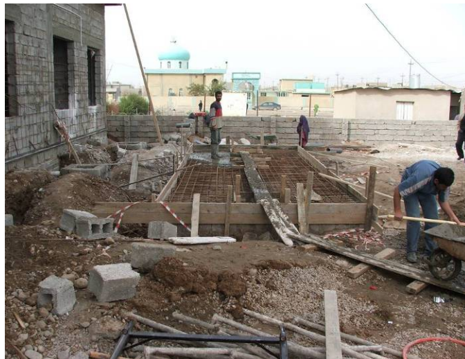
Site Photo 76. Rebar and formwork for the top of the septic tank
