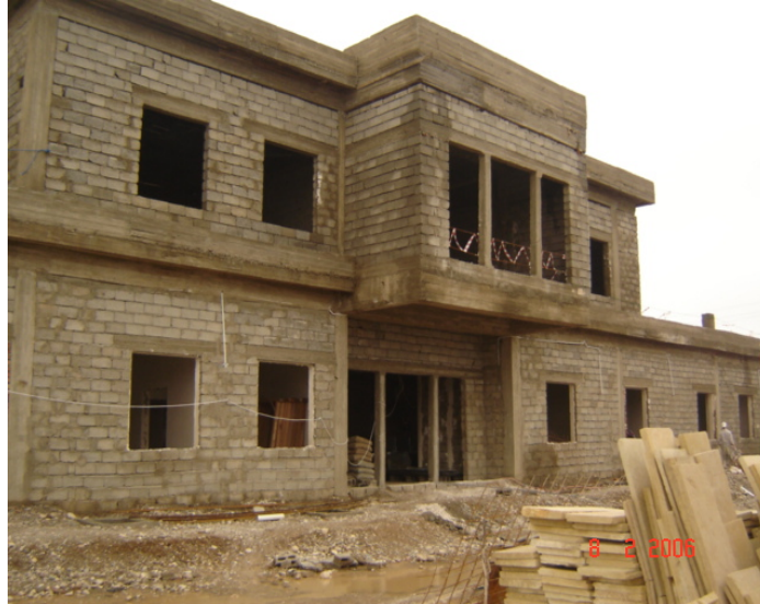
Site Photo 62. View of outside of Hai Al Wesity PHC (Photo courtesy of the USACE)
