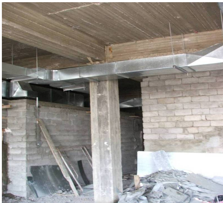
Site Photo 4. Column that is not plumb (PHC Hai Alasra Wa Al Mafqoodeen)
