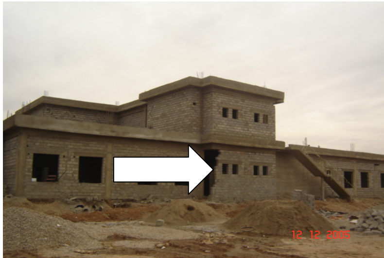
Site Photo 18. View of Hai Alhajjaj on 12 December 2005. According to the PCO construction database, this PHC was 56% complete (Photo courtesy of the USACE)
