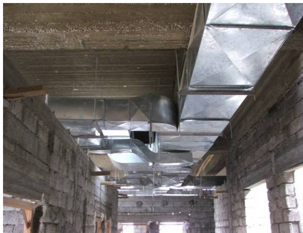
Site Photo 82. Completed ventilation ductwork
