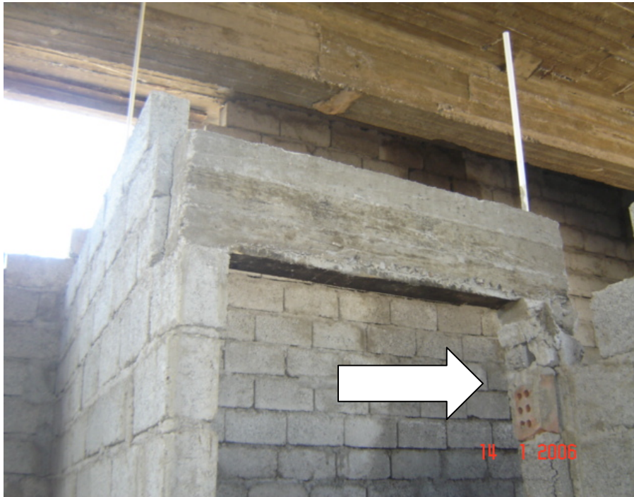
Site Photo 23. Example of a site photo included with the daily report. Taken by the USACE LN QA for PHC Shiqaq Hai Musalla (Photo courtesy of the USACE)
