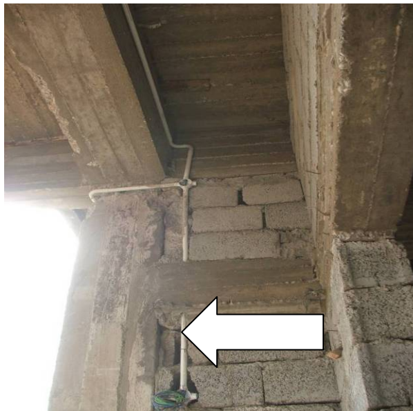
Site Photo 32. Example of broken blocks used in wall construction
