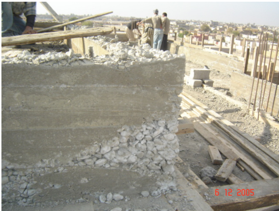
Site Photo 25. Extensive segregation of concrete in the parapet
