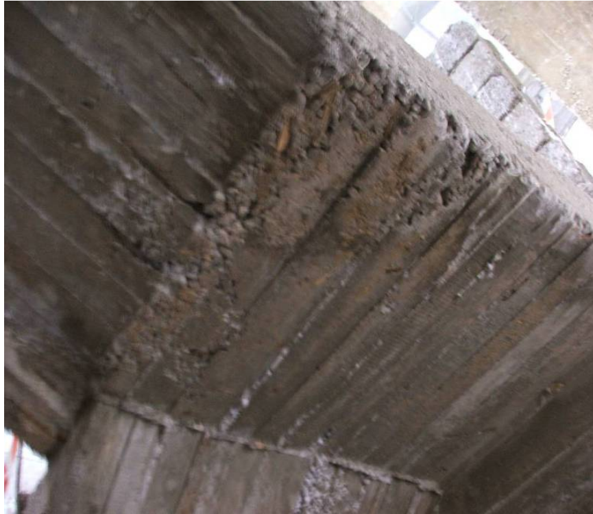
Site Photo 10. Concrete segregation underneath stairwell (PHC Hai Al Wasily)
