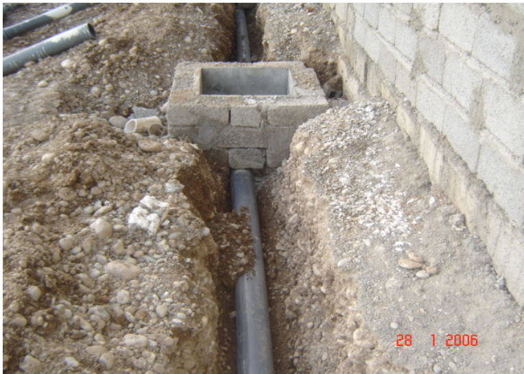
Site Photo 71. Partial installation of sewer drain (Photo courtesy of the USACE)
