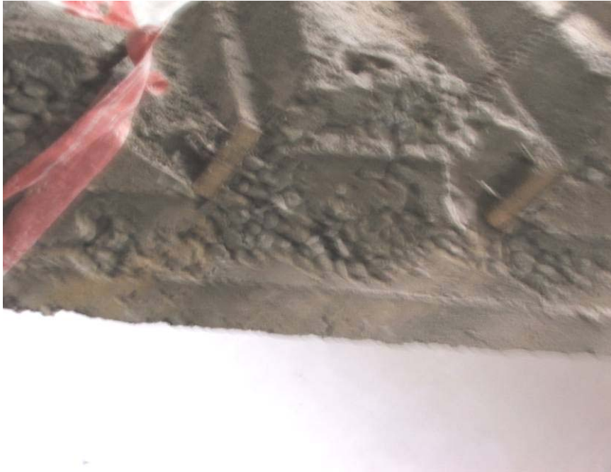
Site Photo 12. Close-up view of concrete segregation on stairwell (PHC Hai Al Wasity)
