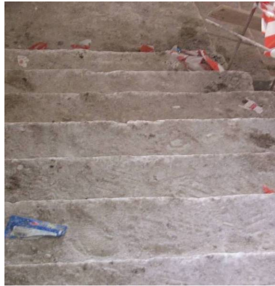
Site Photo 8. Chipped steps (PHC Hai Alhajjaj)
