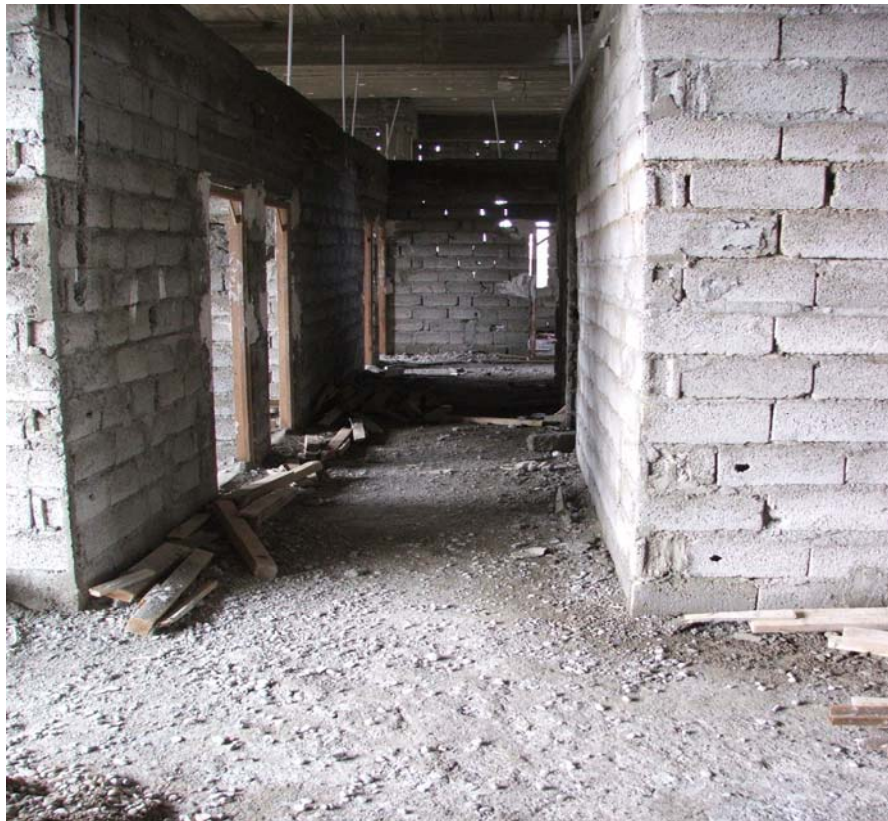
Site Photo 6. Sunlight through gaps in walls (PHC Hai Tis'een)
