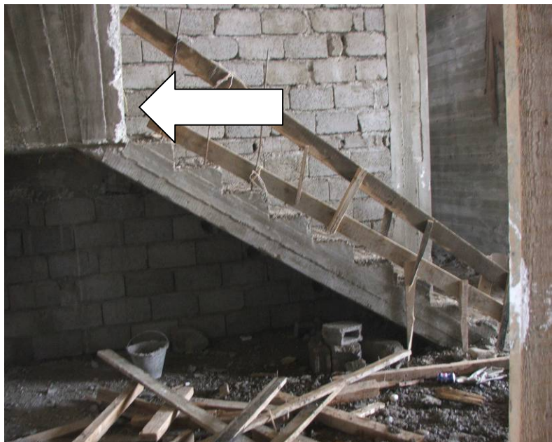
Site Photo 9. Concrete honeycombing on side of stairwell (PHC Hai Tis'een)
