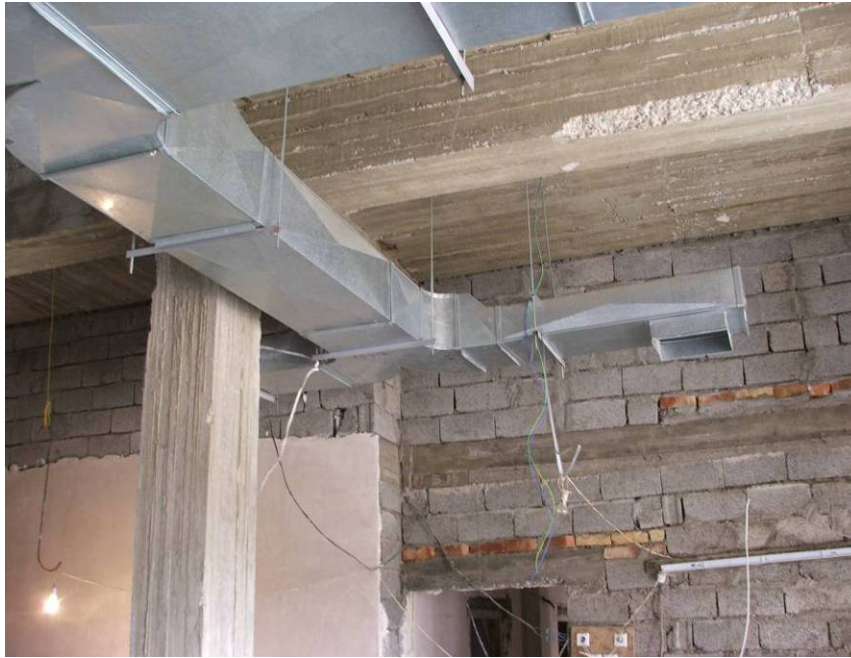
Site Photo 69. Ventilation ductwork
