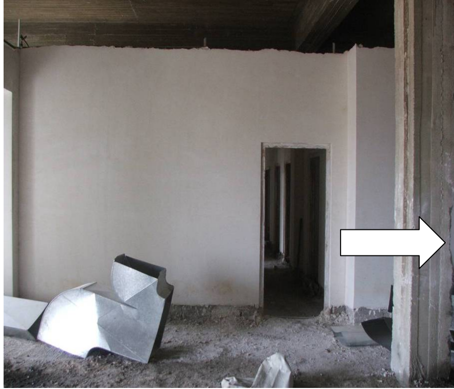
Site Photo 3. Honeycombing of concrete column (PHC Hai Alhajjaj)
