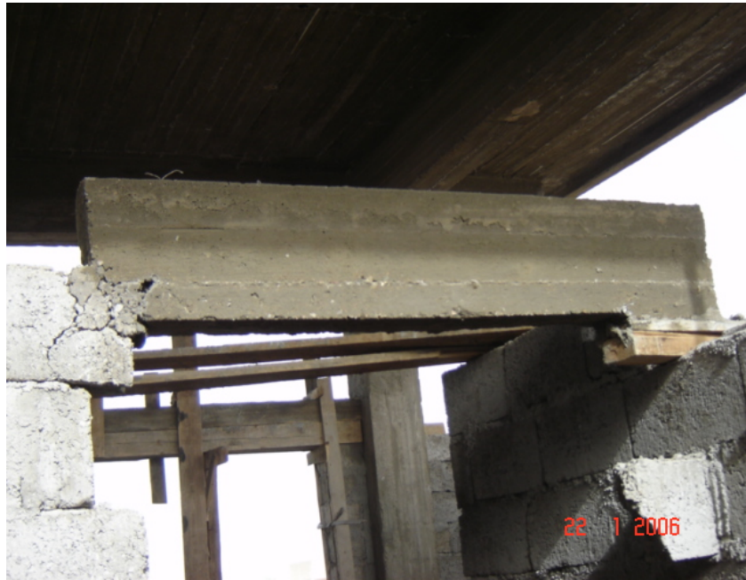
Site Photo 24. Example of a site photo included with the daily report. Taken by the USACE LN QA (Photo courtesy of the USACE)
