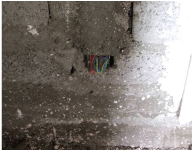
Site Photo 68. Wires within outlet box
