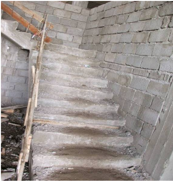
Site Photo 7. Uneven steps (PHC Hai Tis'een)
