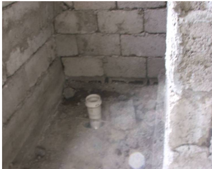
Site Photo 46. Bathroom plumbing pipes
