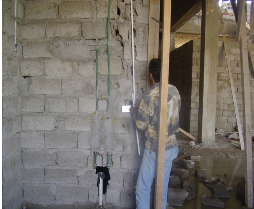
Site Photo 5. Example of poor block laying (PHC Hai Tis'een) (Photo courtesy of the USACE)
