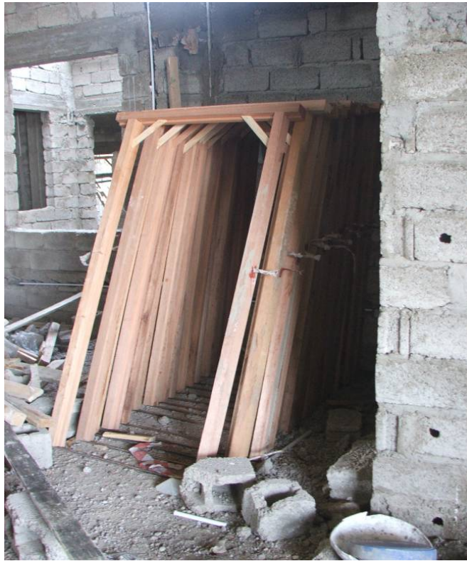
Site Photo 60. Doorframes on site but not installed
