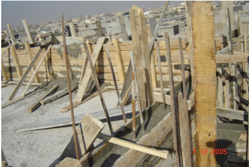
Site Photo 22. View of Hai Alasra Wa Al Mafqoodeen on 7 December 2005. According to the PCO database, this PHC was 50% complete (Photo courtesy of the USACE)
