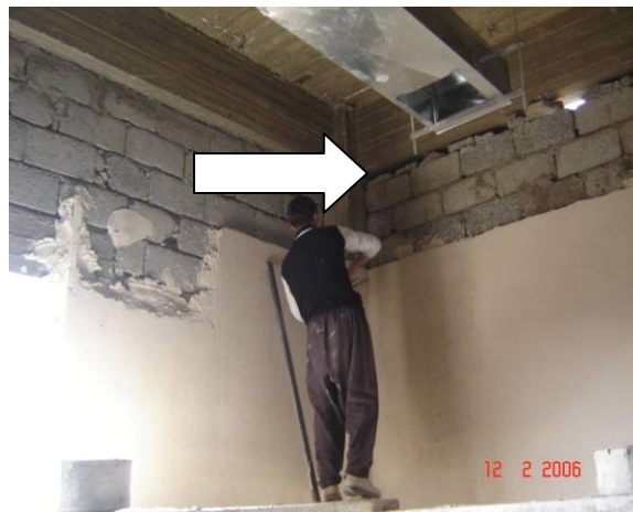
Site Photo 65. Example of broken and different sized blocks used in wall construction (Photo courtesy of the USACE)
