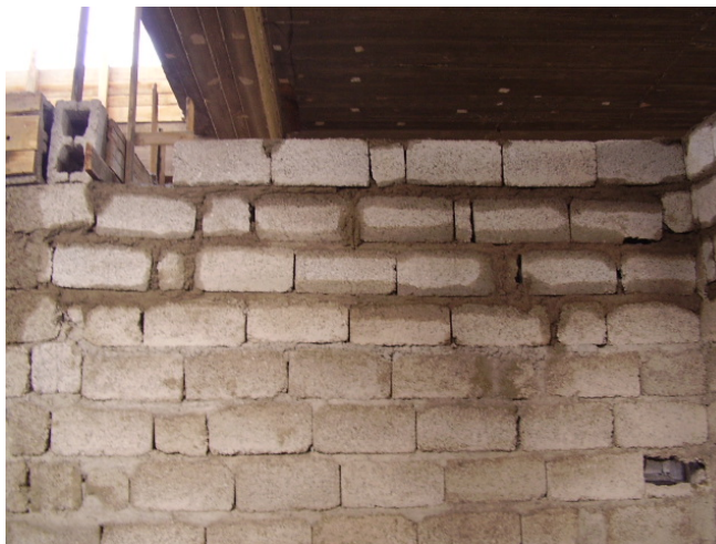
Site Photo 54. Example of different sized blocks in wall construction (Photo courtesy of the USACE)
