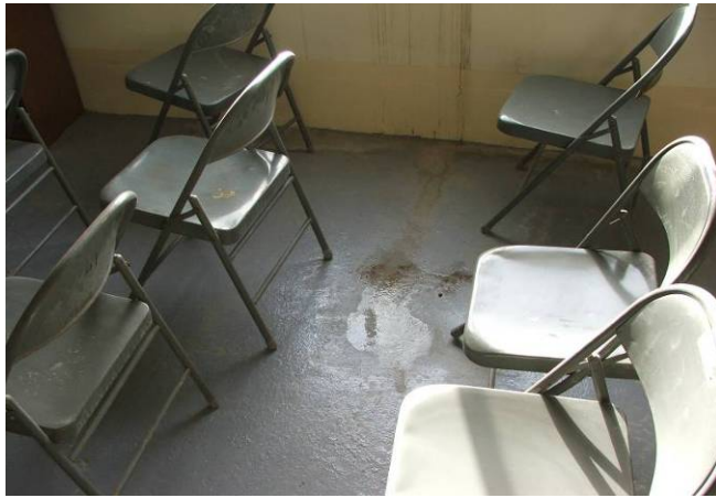
Site Photo 10. Water on floor because of window leakage
