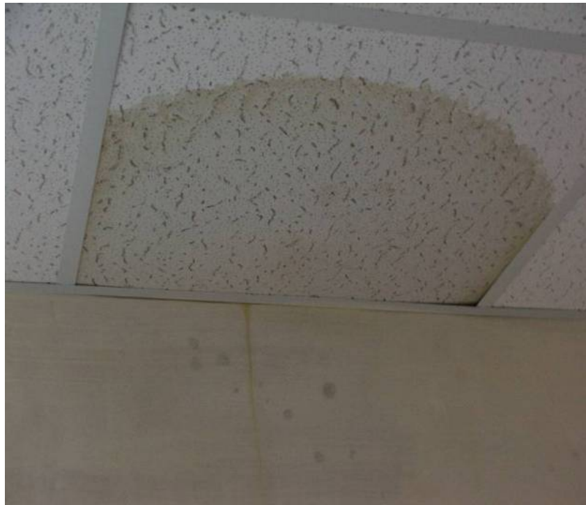
Site Photo 27. Evidence of water leakage
