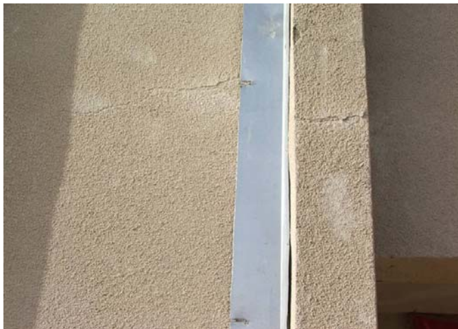
Site Photo 30. Cracks in the outside wall stucco
