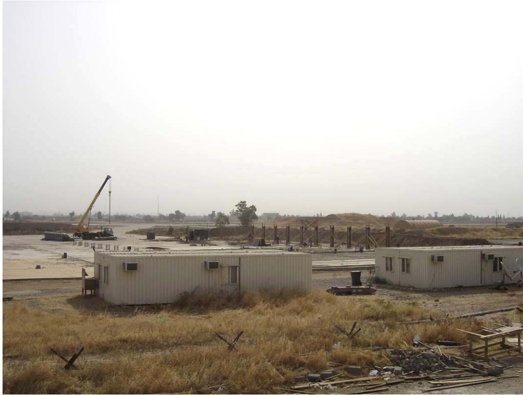
Site Photo 1. Preconstruction location of future hangar site (beyond trailers) (Photo courtesy of ECC)
