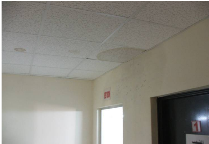
Site Photo 28. Example of water leakage
