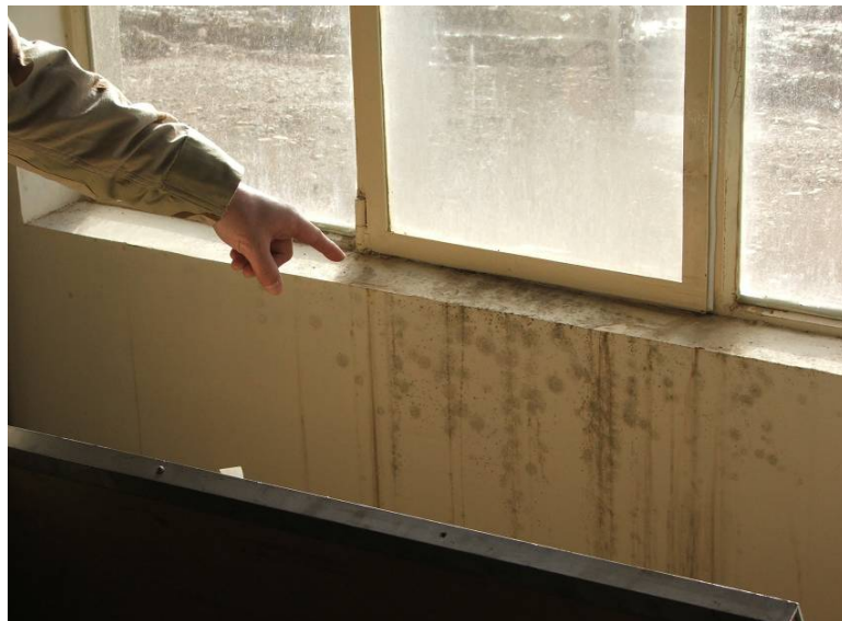
Site Photo 9. SIGIR Engineer pointing out water leakage
