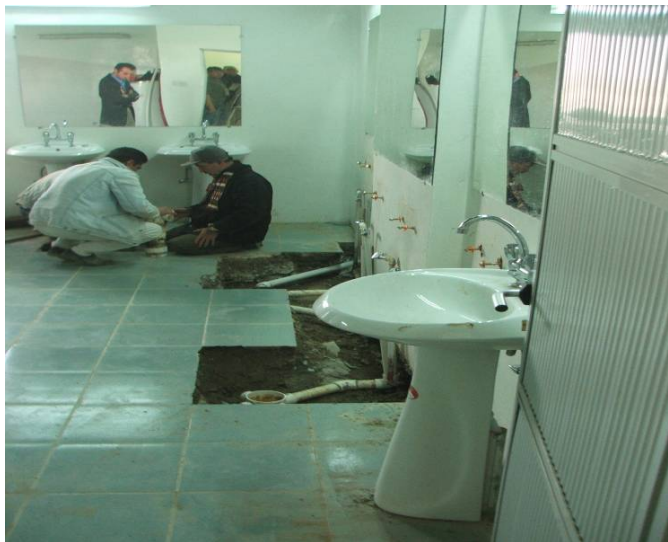
Site Photo 29. Floor tiles removed to determine cause of leak
