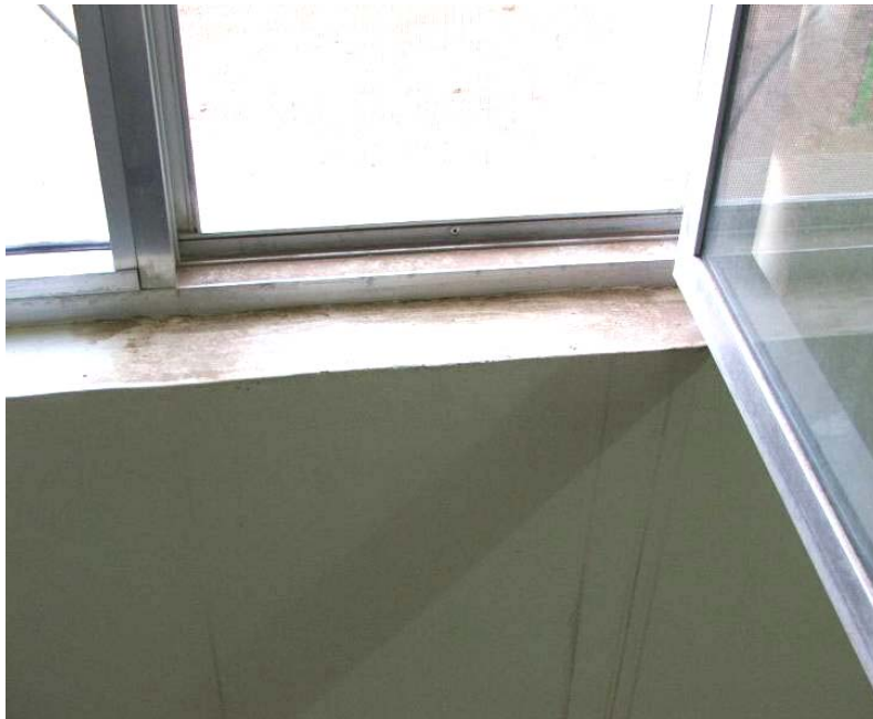
Site Photo 21. Close-up view of water leaking through window
