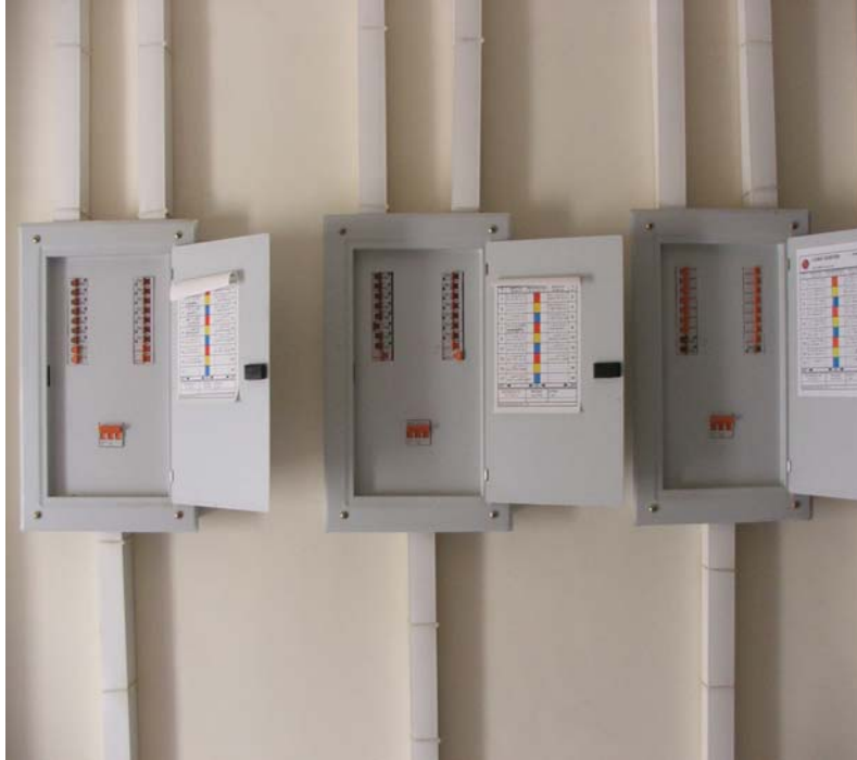
Site Photo 20. Circuit breaker
