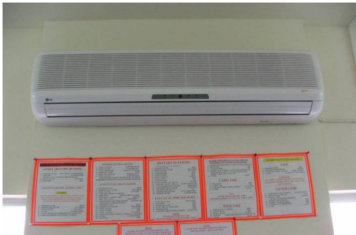
Site Photo 16. Split A/C unit in rooms
