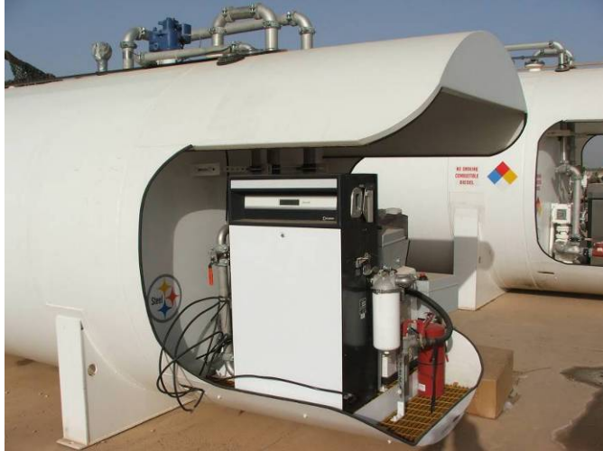
Site Photo 33. Close-up of fuel tank
