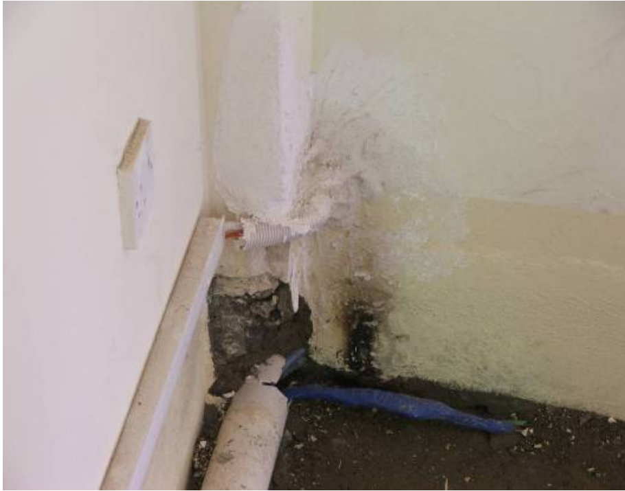
Site Photo 13. Small fire damage and repair to the wiring
