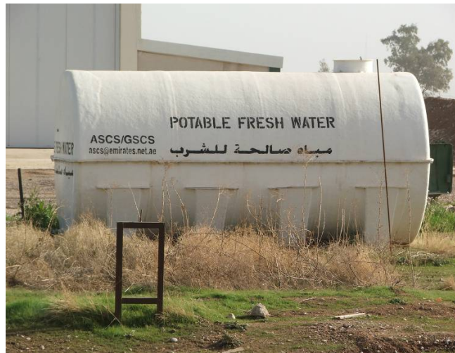
Site Photo 31. Potable water supply
