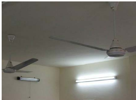
Site Photo 19. Ceiling fans within each living quarters
