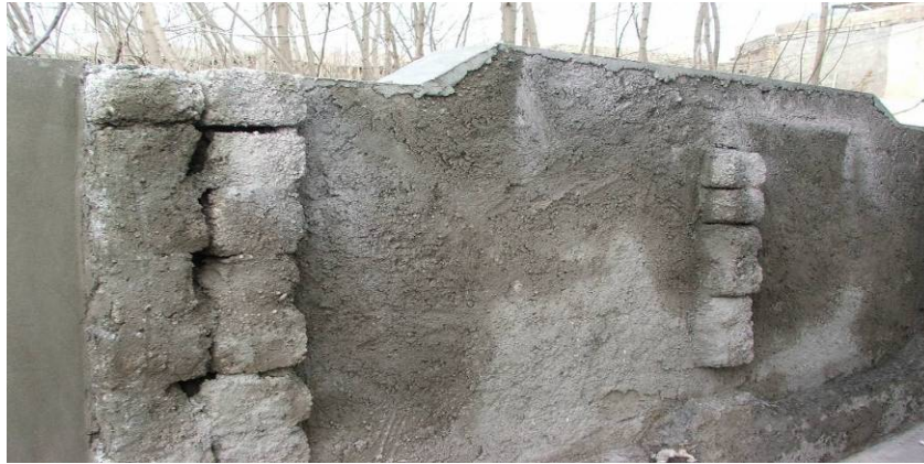
Site Photo 12. Unfinished perimeter wall
