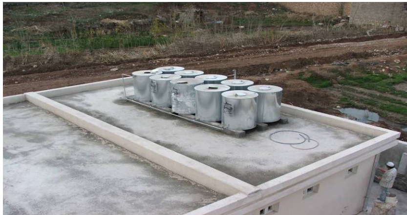
Photo 4. Water tanks installed on roof of the auxiliary building
