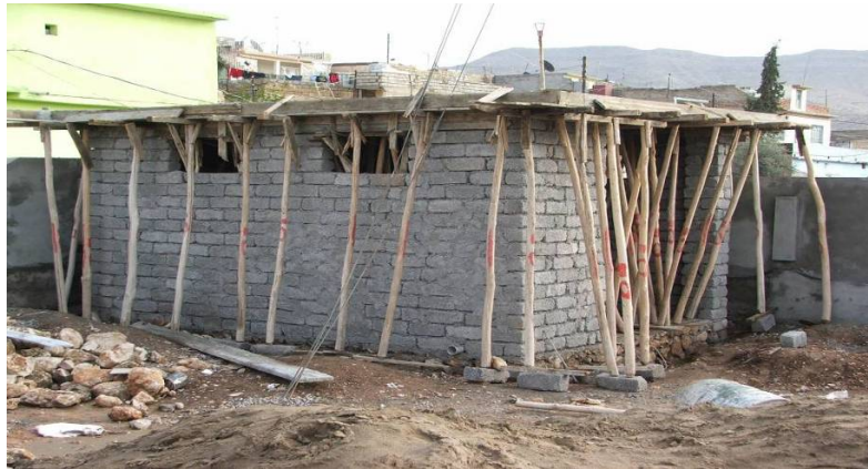
Site Photo 9. Generator building
