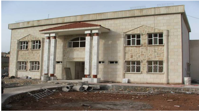
Site Photo 3: Front of the building at the time of the assessment
