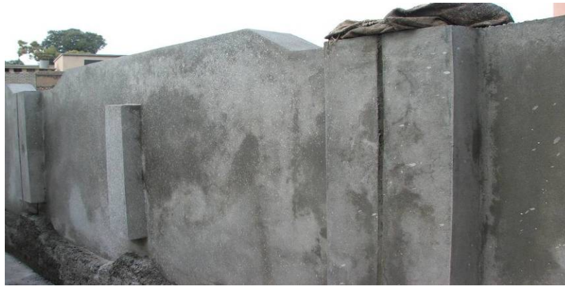
Site Photo 13. Perimeter wall with unpainted cement finish
