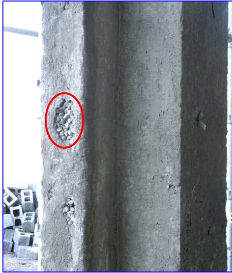
Site Photo 5. Honeycombing after surface coating
