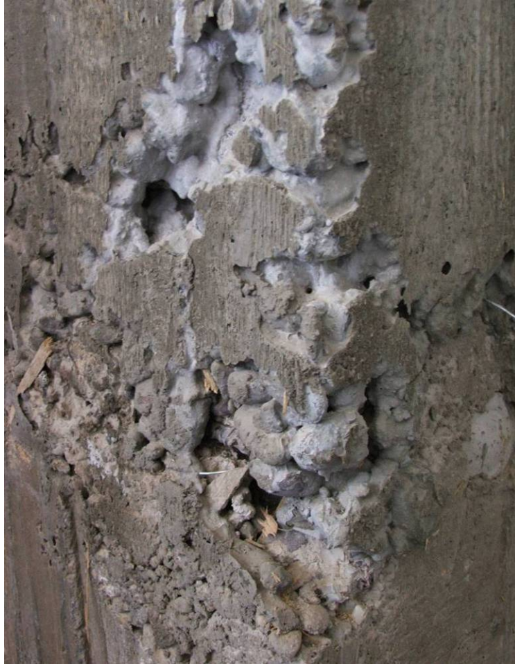
Site Photo 8. Honeycombing on Level 2 column
