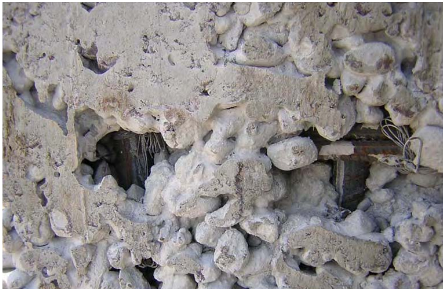
Site Photo 7. Honeycombing and exposed rebar in concrete on Level 1. Photo provided by USACE.
