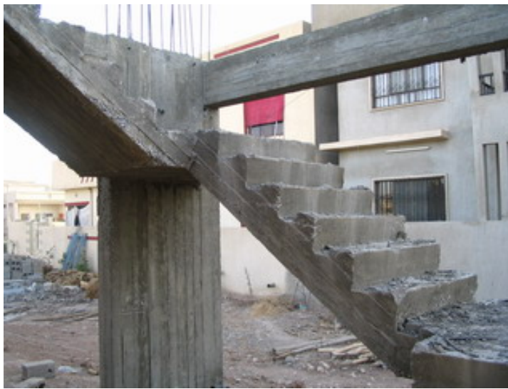
Site Photo 10. Staircase construction and supporting shear wall. Photo provided by USACE.
