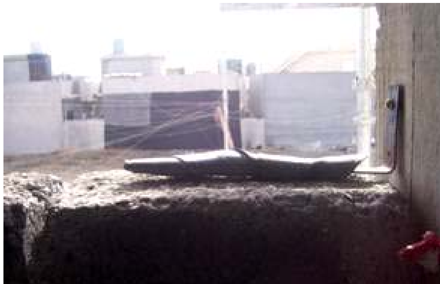
Site Photo 15. Concrete block wall tie-in connection to structural frame. Photo provided by USACE.
