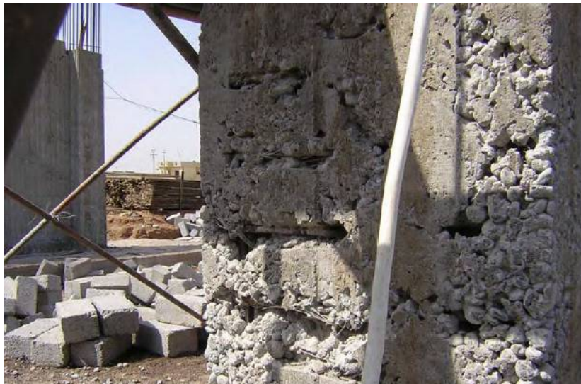
Site Photo 4. Honeycombing/exposed reinforcing steel in concrete column on Level 1 - Photo provided by USACE.
