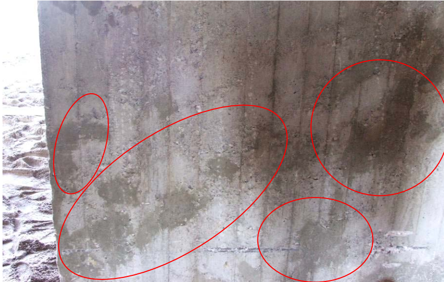
Site Photo 9. Rich cement-sand patches made on a Level 1 shear wall
