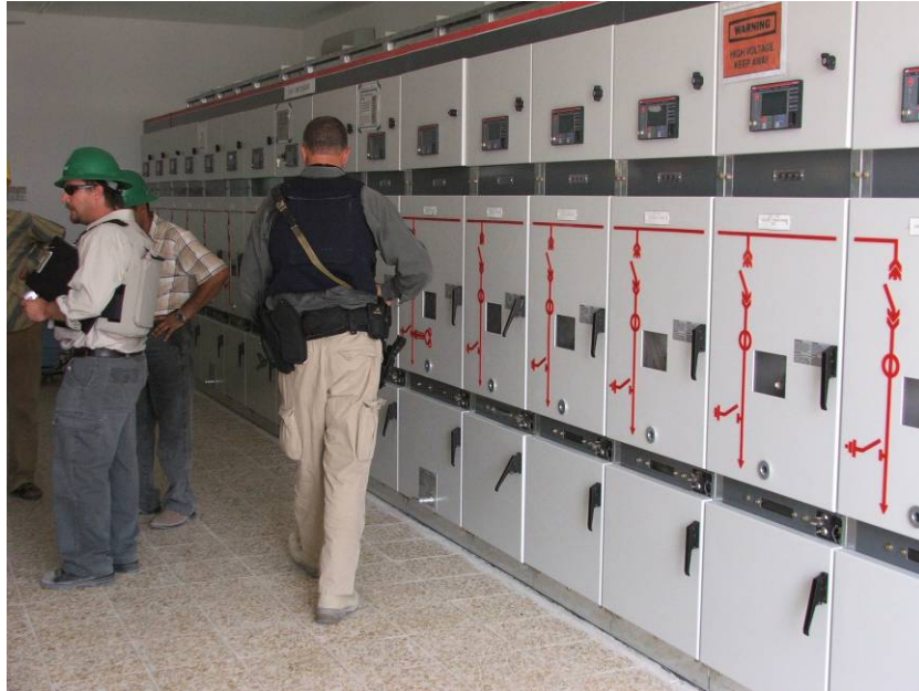
Site Photo 4: 11 kV switchgear
