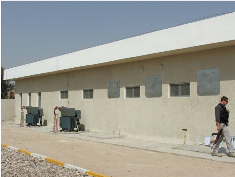
Site Photo 1: Substation building exterior view
