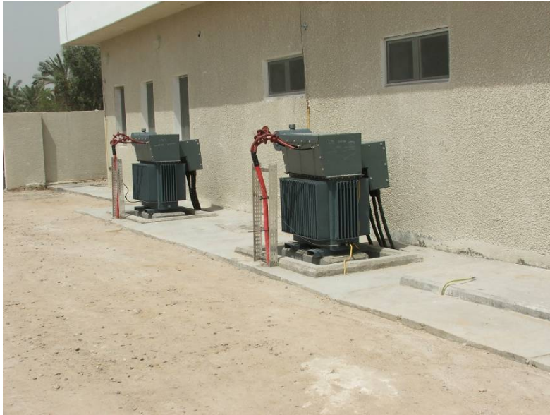
Site Photo 6: 11 to .4 kV auxiliary transformers
