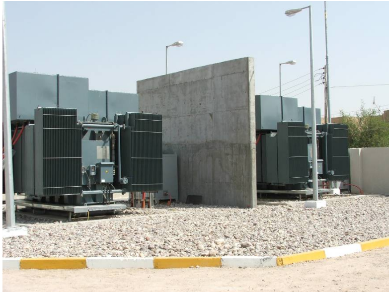
Site Photo 5: 33 to 11kV transformers
