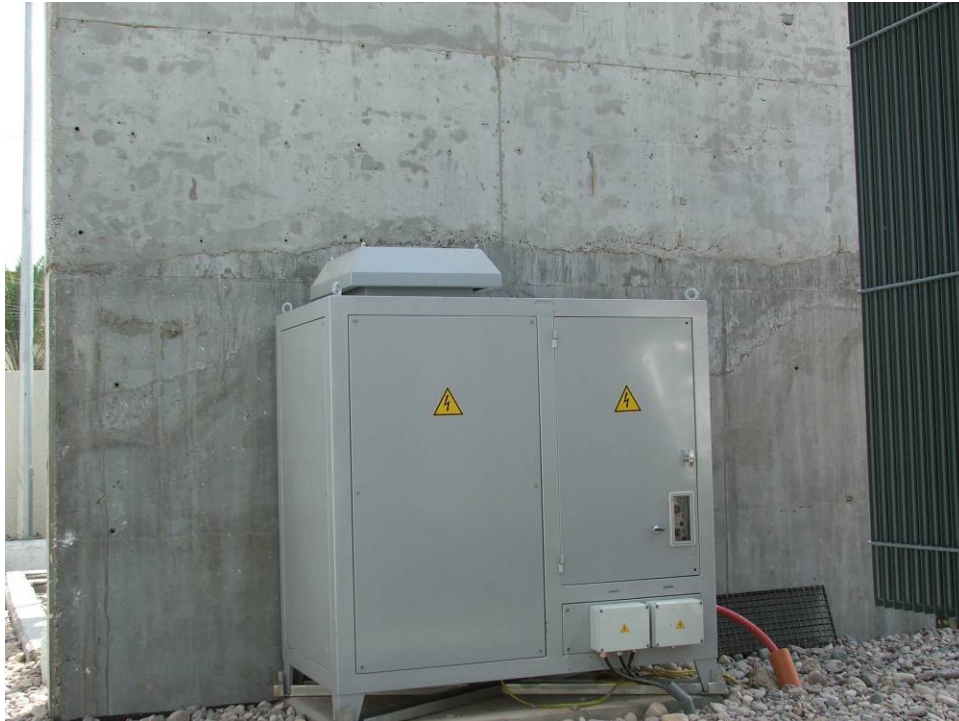
Site Photo 7: Grounding system
