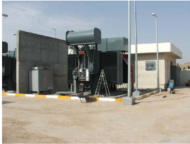
Site Photo 5: 33 to 11 kV transformer
