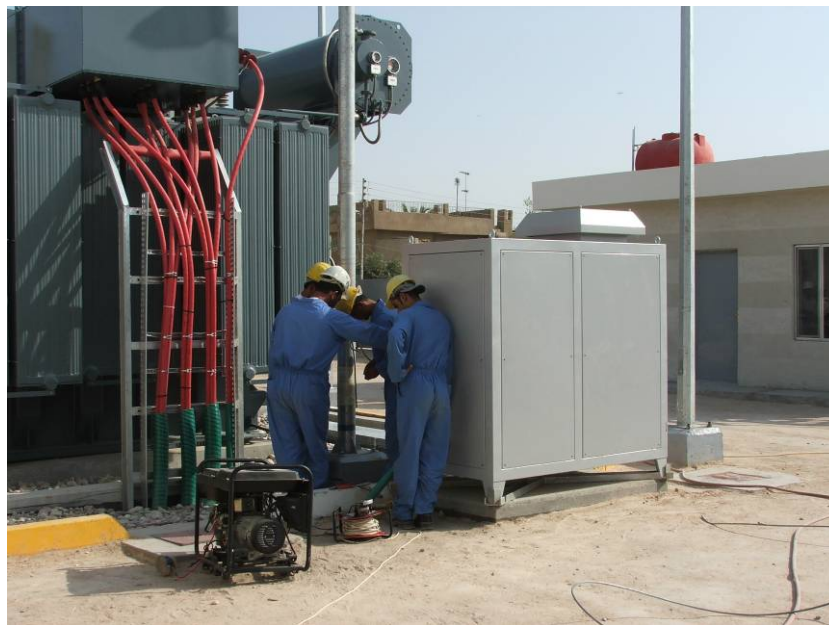
Site Photo 7: Grounding system
