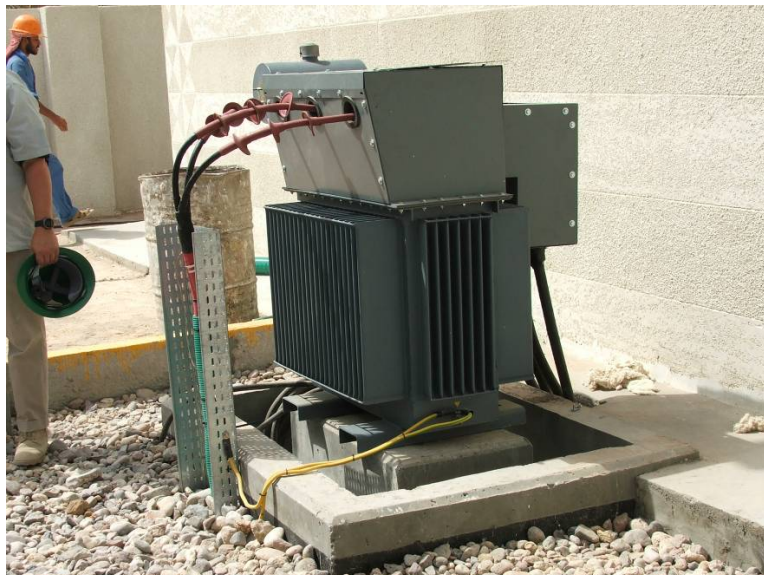
Site Photo 6: 11 to 0.4 kV auxiliary transformers
