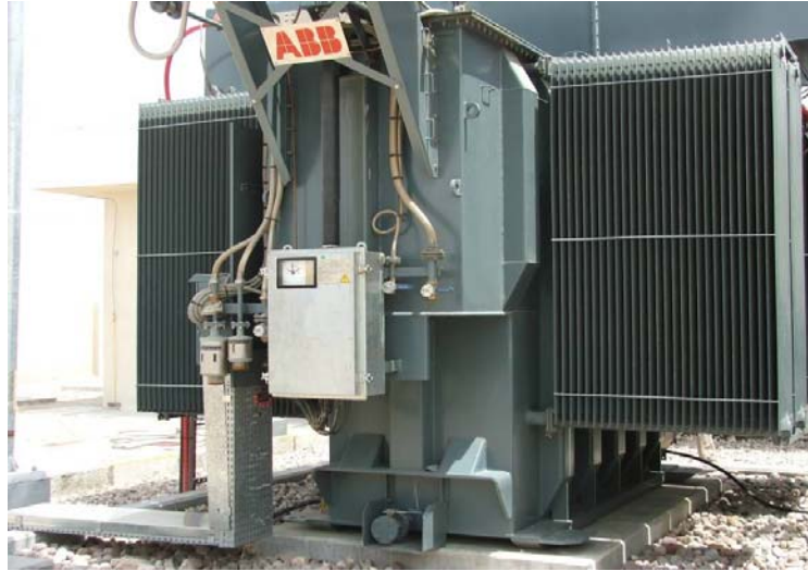
Site Photo 5: 33 to 11 kV transformer
