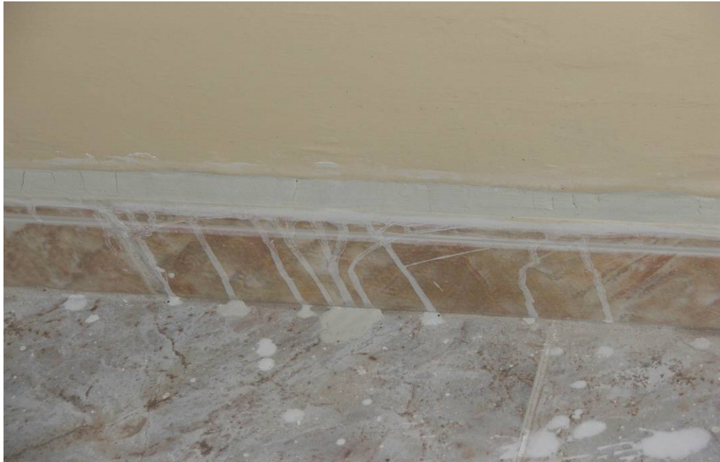
Site Photo 16. Paint and Molding in Need of Correction
