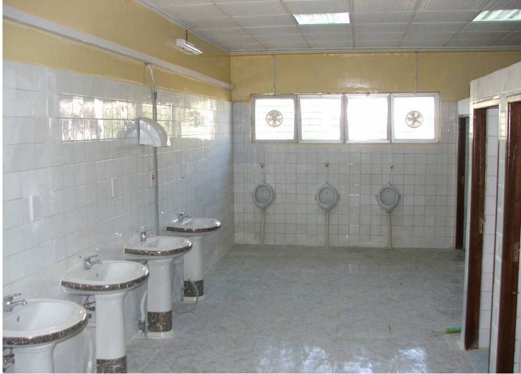
Site Photo 7. Bathroom Sinks, Exhaust Fans, and an Electric Hand Dryer
