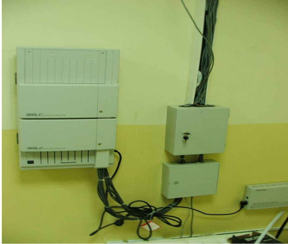
Site Photo 14. Wiring for the Security Surveillance System
