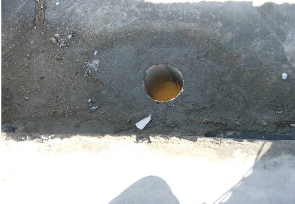
Site Photo 6. Example of Down Spout. A recent rain resulted in a leak in this area.
