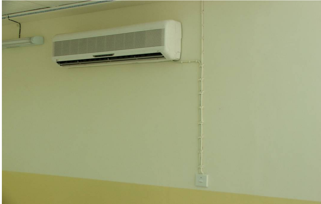
Site Photo 9. Interior wall mounted part of split A/C Unit
