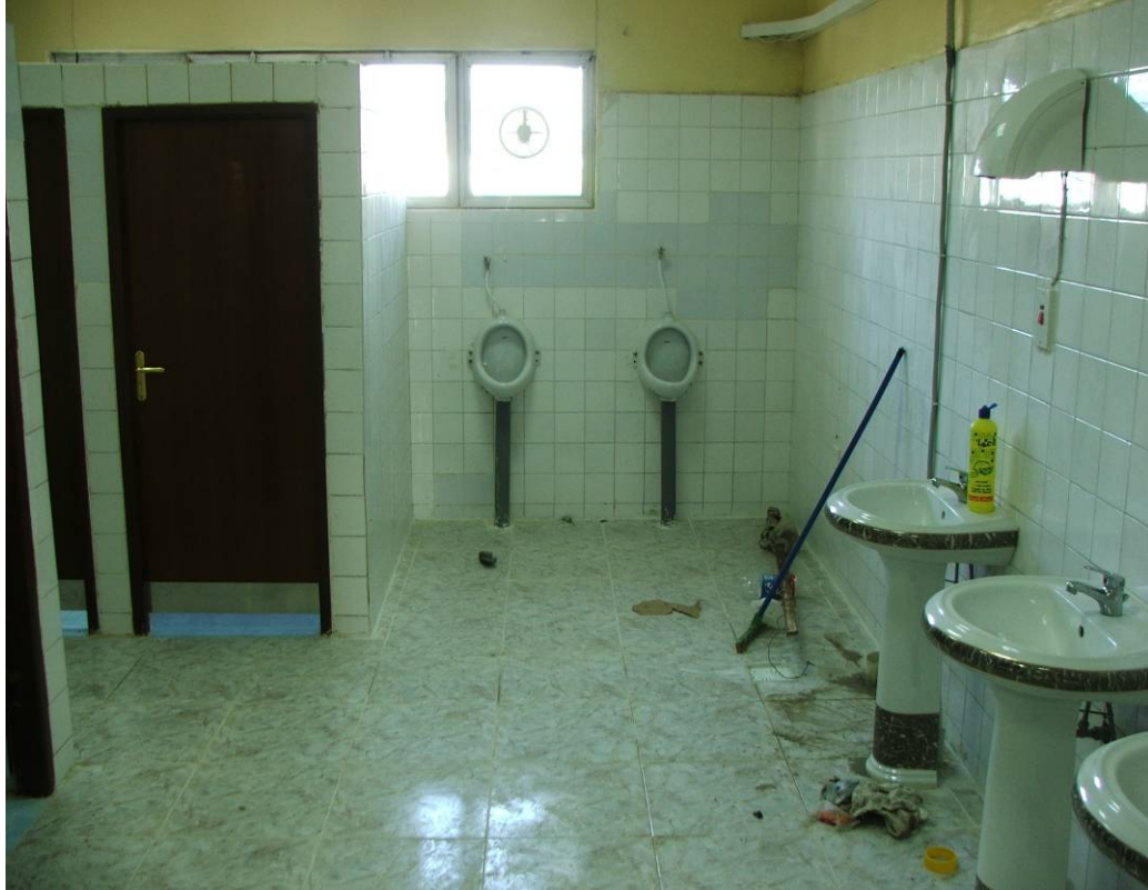
Site Photo 15. Bathroom with Additional Repairs Required
