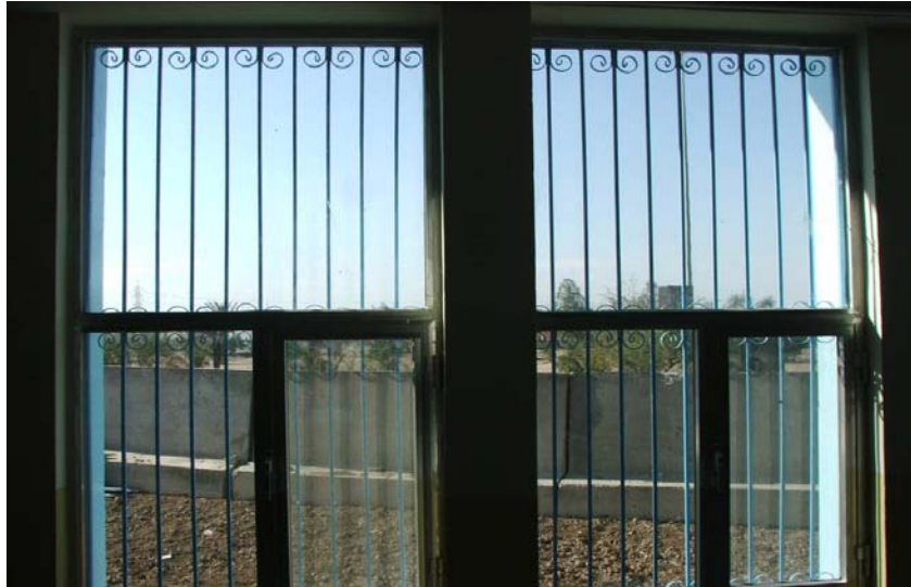
Site Photo 12. Window Security Bars
