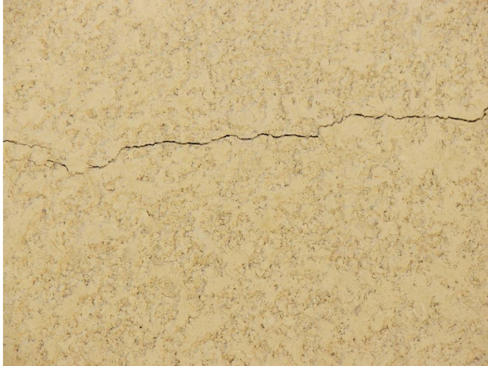
Site Photo 7. Crack in Stucco Wall Outside the ASP
