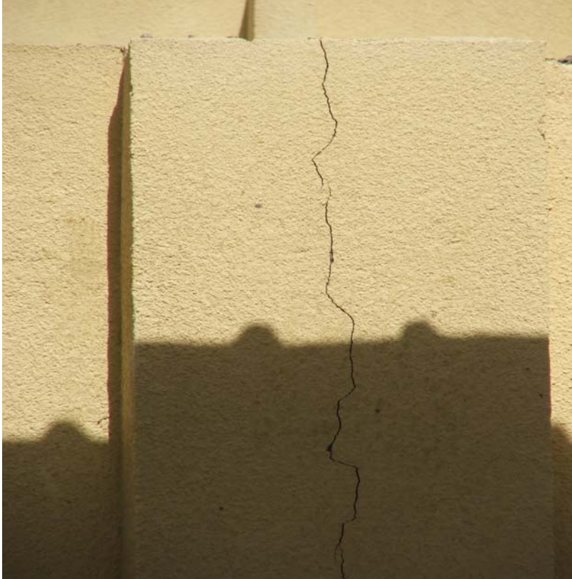
Site Photo 21. Cracks in Stucco of Interior Security Wall
