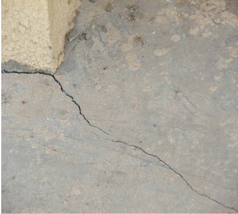
Site Photo 20. Cracks in Concrete Sidewalks of Renovated Building #2
