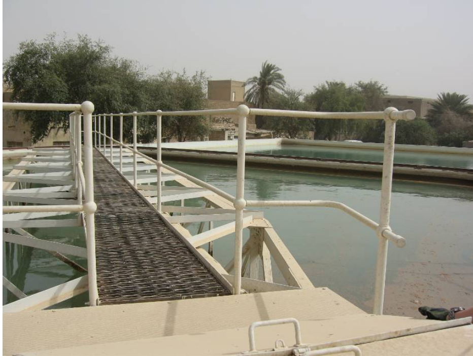
Site Photo 1: Clarifier tank
