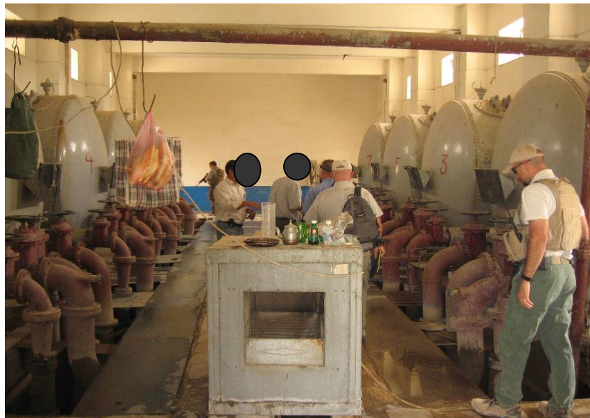
Site Photo 7: Pressure filters and piping
