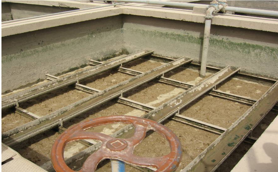
Site Photo 5: Rapid sand gravity filter
