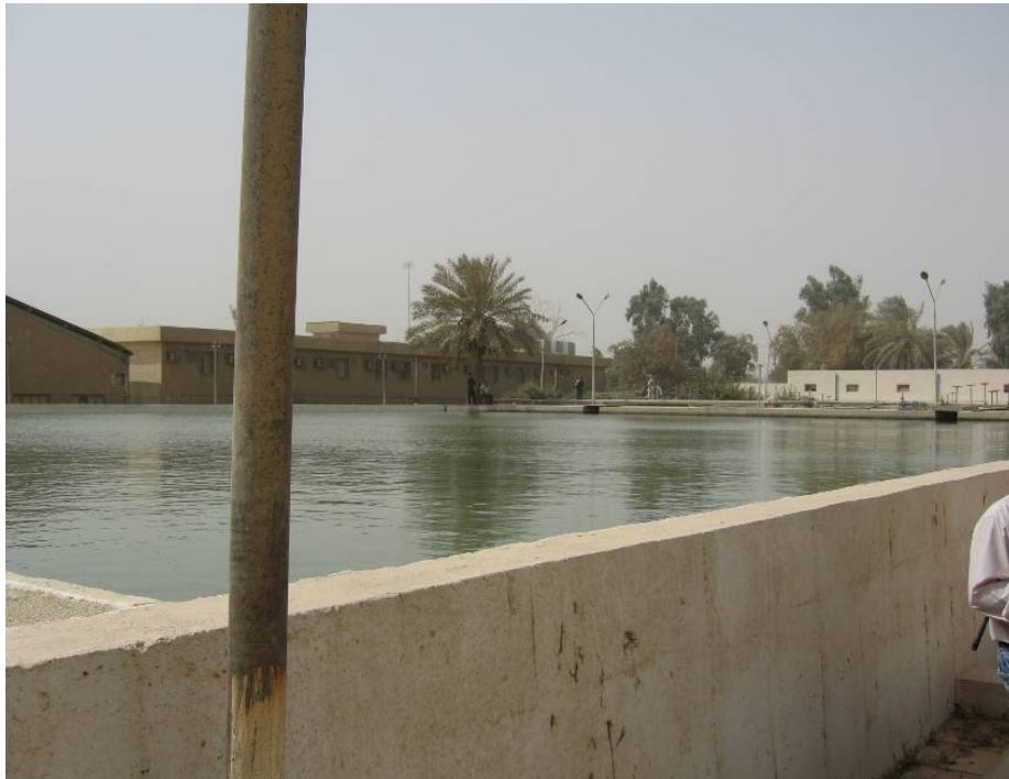
Site Photo 2: Settling tank
