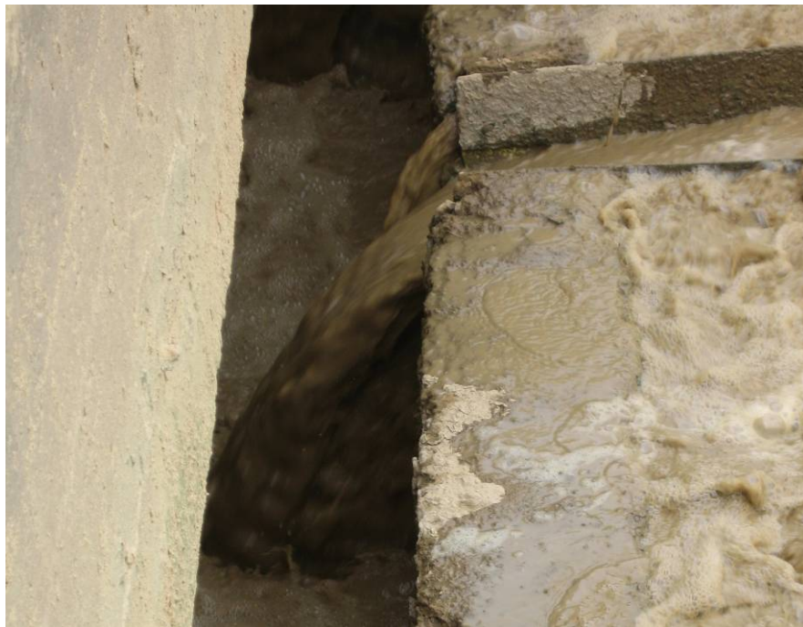
Site Photo 6: Backwash effluent
