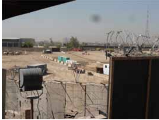
Ongoing renovation work at Forward Operating Base Shield, the main PDP basing area.
