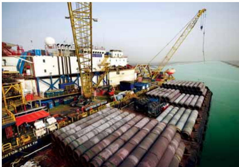
Pipelines being laid off al-Faw Peninsula to connect Iraq's offshore crude oil loading facilities (now under construction) with onshore tank farms. (Leighton Offshore photo)
