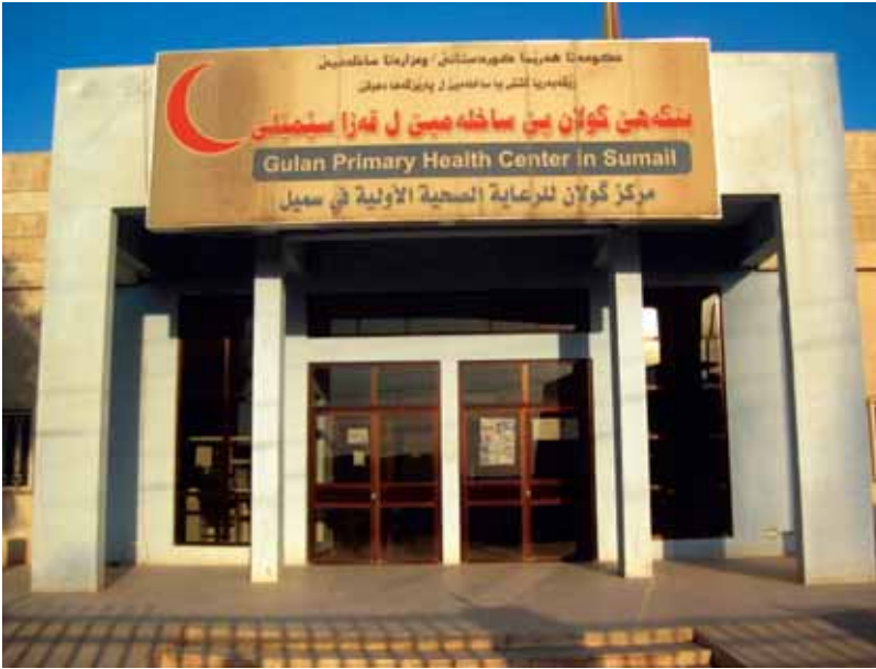
Primary health care center in need of repairs to prevent radiation leakage from x-ray equipment. (USACE photo)
