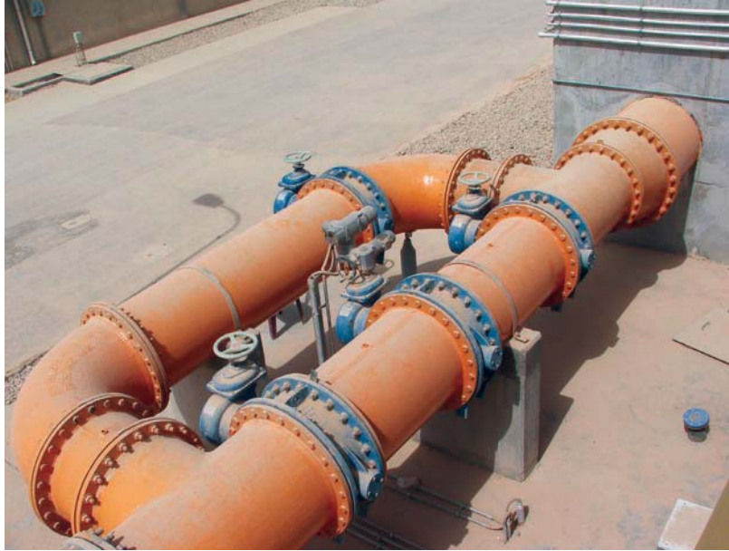
Sadr City water project: raw water metering and flow-control station.
