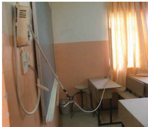
Improper electrical connection at the Al Mualameen school.
