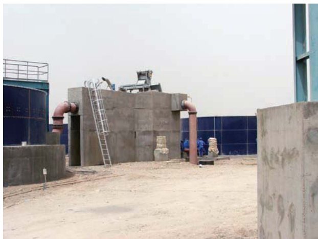
Falluja wastewater project: Inlet tank and screen structure.
