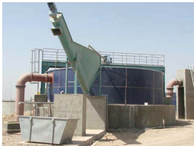
Falluja wastewater project: Oil and grit tank and classifier.
