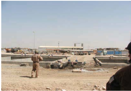
SIGIR's comprehensive review of the Falluja Waste Water Treatment System found that the project will cost three times original estimates, be completed three years late, and serve far fewer homes than originally contemplated.
