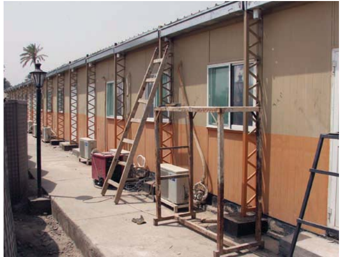
Reinforcement for collapsing building roofs at Hilla Police Academy: another example of poor construction under a contract awarded to Bloom.
