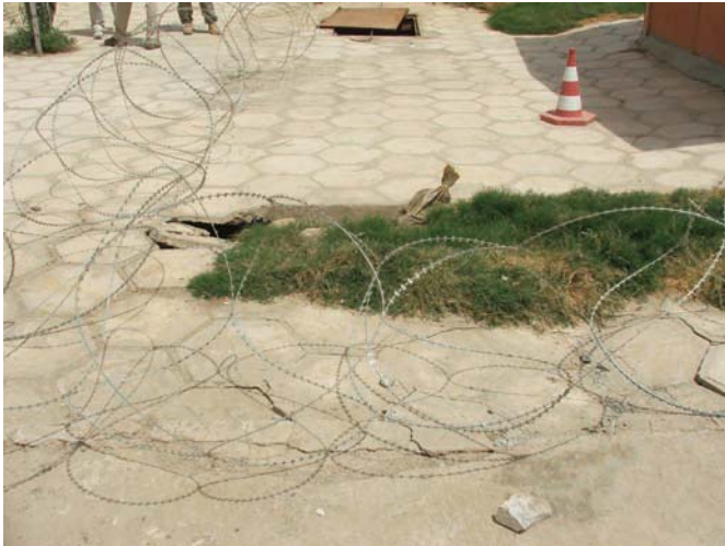
Collapsing septic system at Hilla Police Academy: an example of poor construction under contracts awarded to Philip Bloom.
