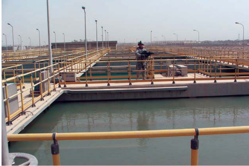
Sadr City water project: flocculation tanks.
