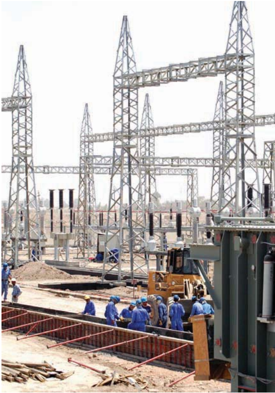
Construction of the Diwaniyah 132kV AIS Substation in Qadissiya now completed. (USACE photo)
