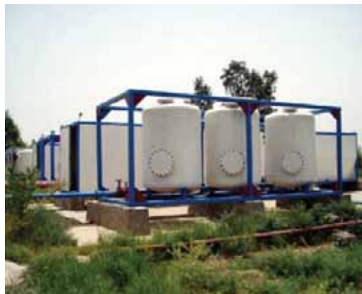
A typical water treatment unit located in Basrah province. (USAID photo)
