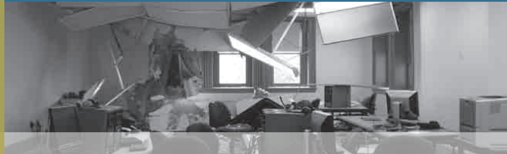
During the earthquake, stone and debris crashed through the roof into our offices.
